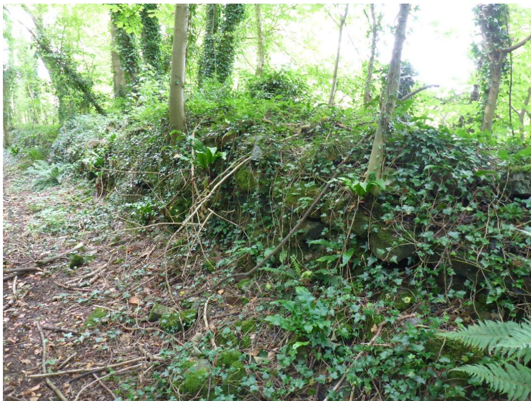
Plate 26: Retention wall 137 at the north side of the railway cutting, viewed facing west
