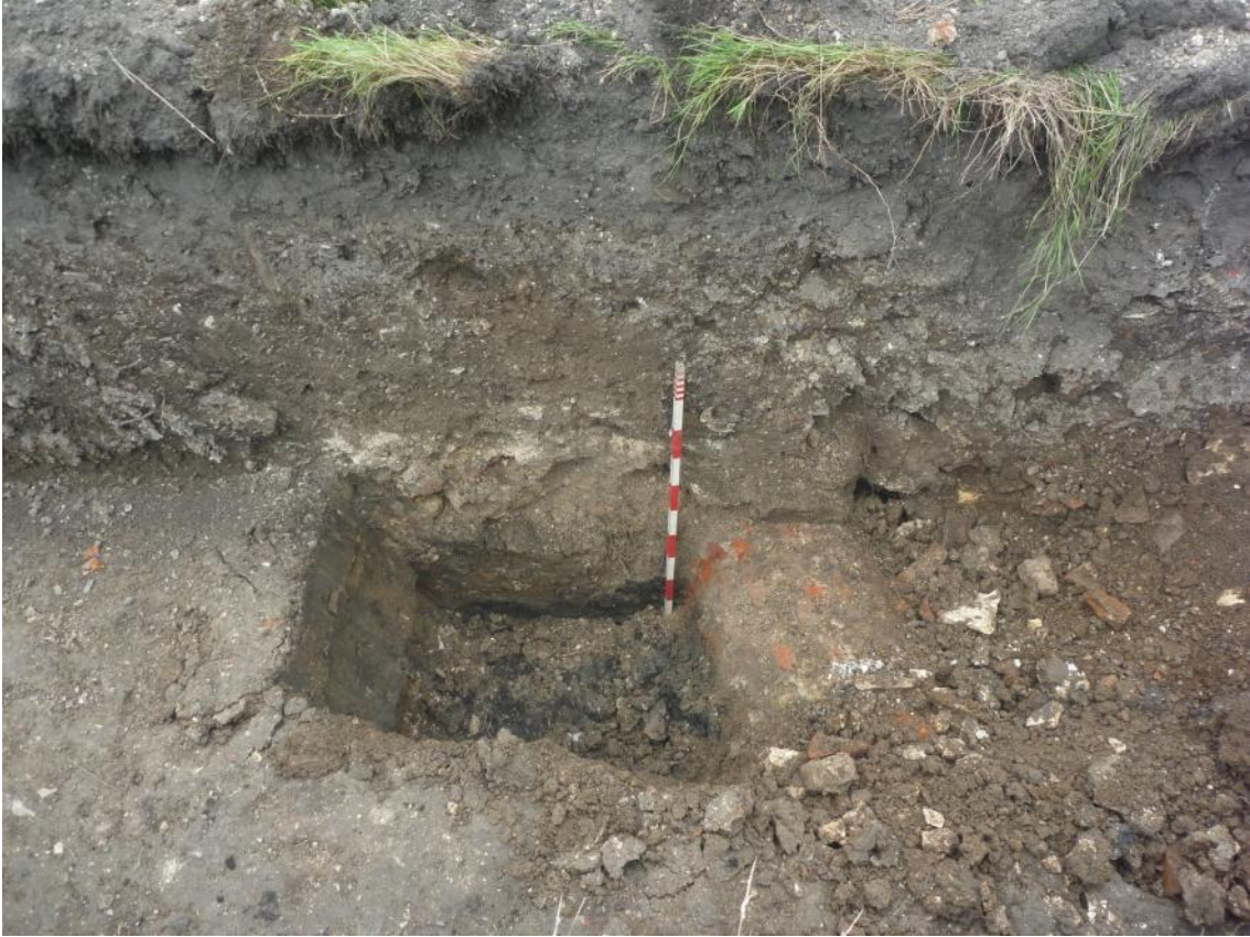
Plate 27: Pit [5003], Trench 5, following further excavation with machine, revealing a brick-built sewer. An organic layer was also observed beneath (5006). Looking north-west, scale 1m
