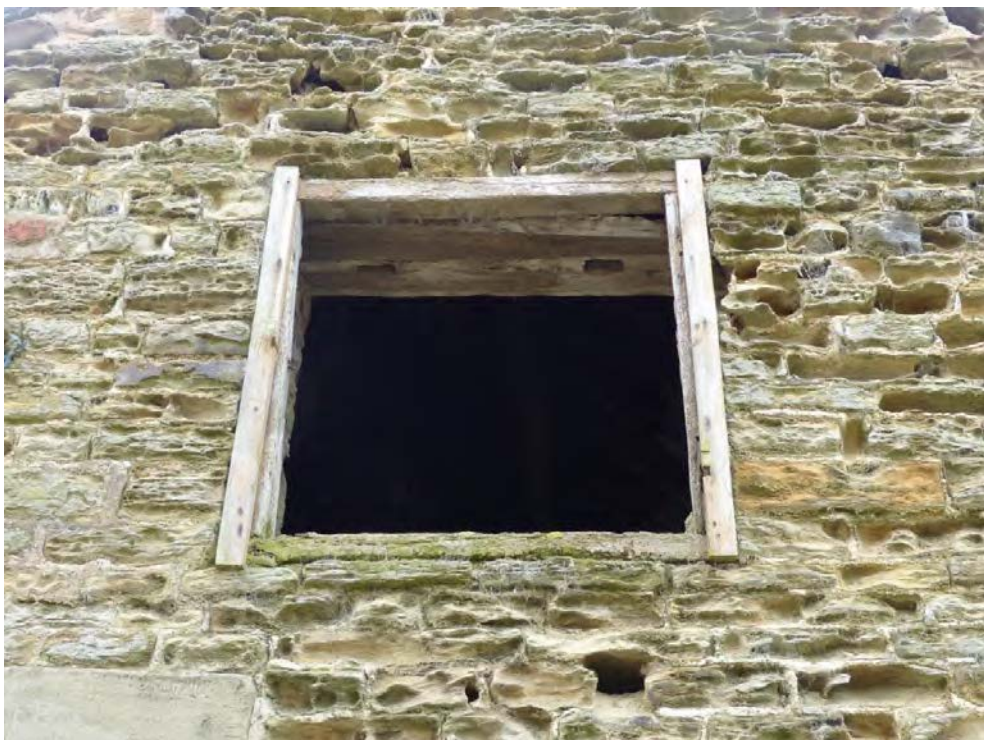
Plate 14: Cruck 1 looking south showing empty mortice holes in the underside of the collar
