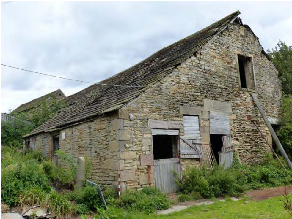
Plate 19: the outshot on the west side of the cruck barn, looking north-east
