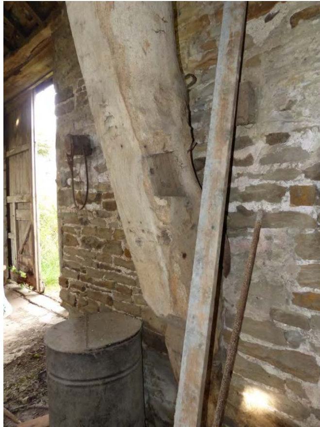
Plate 17: Cruck 4 looking north-east and showing empty dovetail joint for a further horizontal timber
