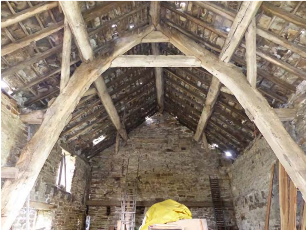
Plate 33: Bay 5 showing remains of floor joists in east, west and south walls
