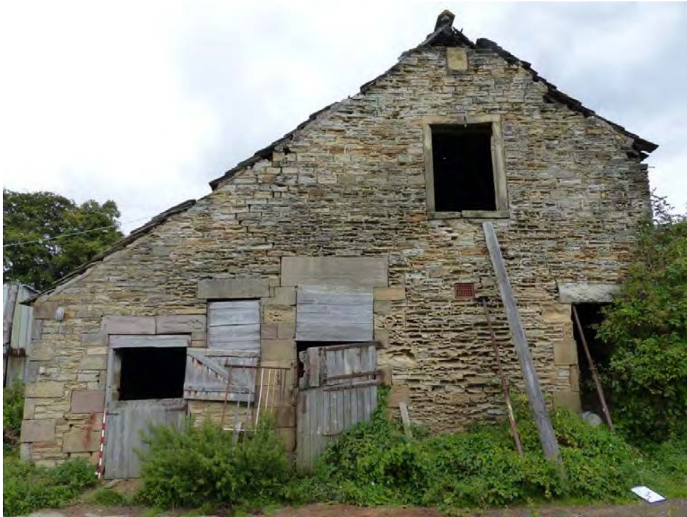
Plate 27: South gable looking north from right to left, the doorways give access to the staircase to Area F, Area B and Area C
