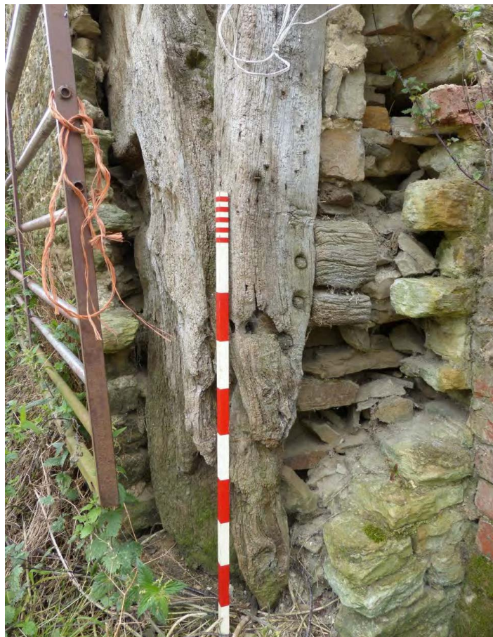
Plate 12: Cruck 1 base looking south-east and showing sawn-off horizontal timber
