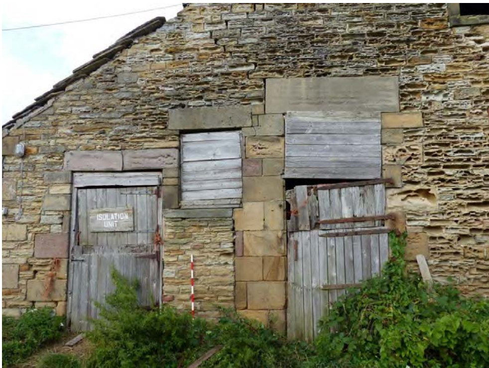
Plate 28: South gable looking north, detail of masonry blocks surrounding doorways and window
