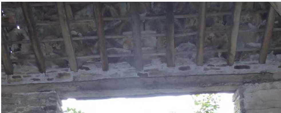
Plate 16: The shaped brackets of the original harr-hung door (each with three oak pegs) can be seen in the wall plate above the opening (one to each side)
