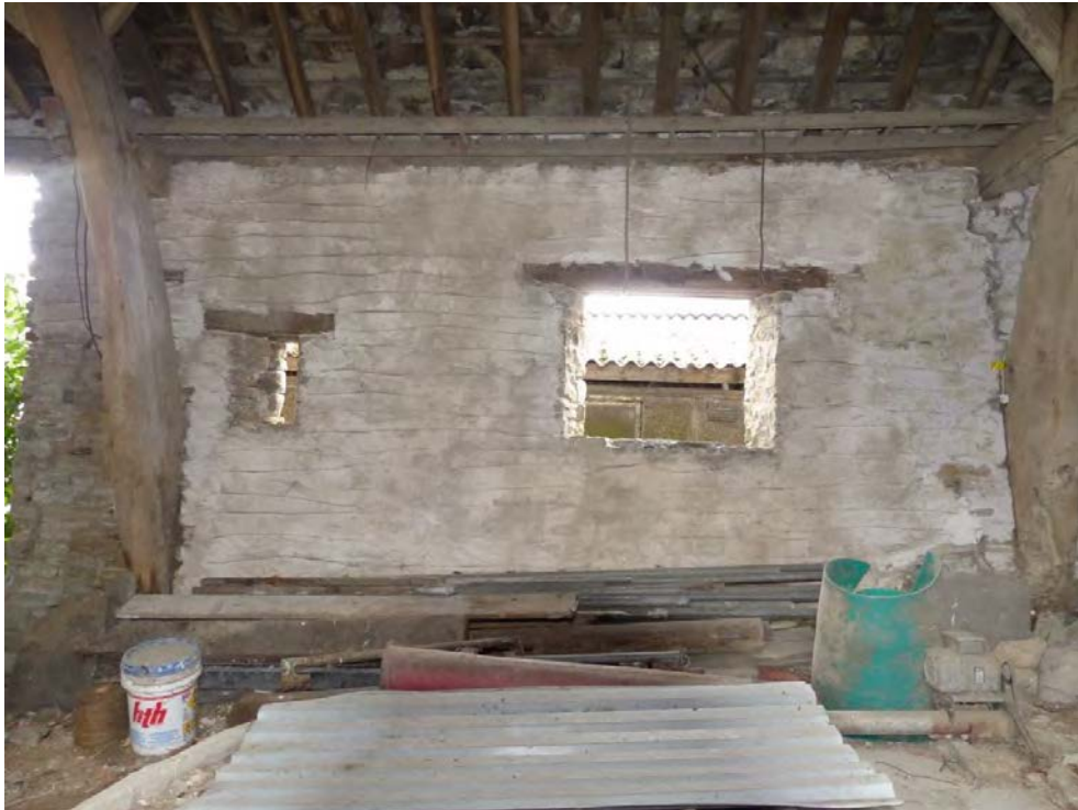
Plate 21: Bay 2 looking west and showing a slit window to the left of the photograph and a square window to right
