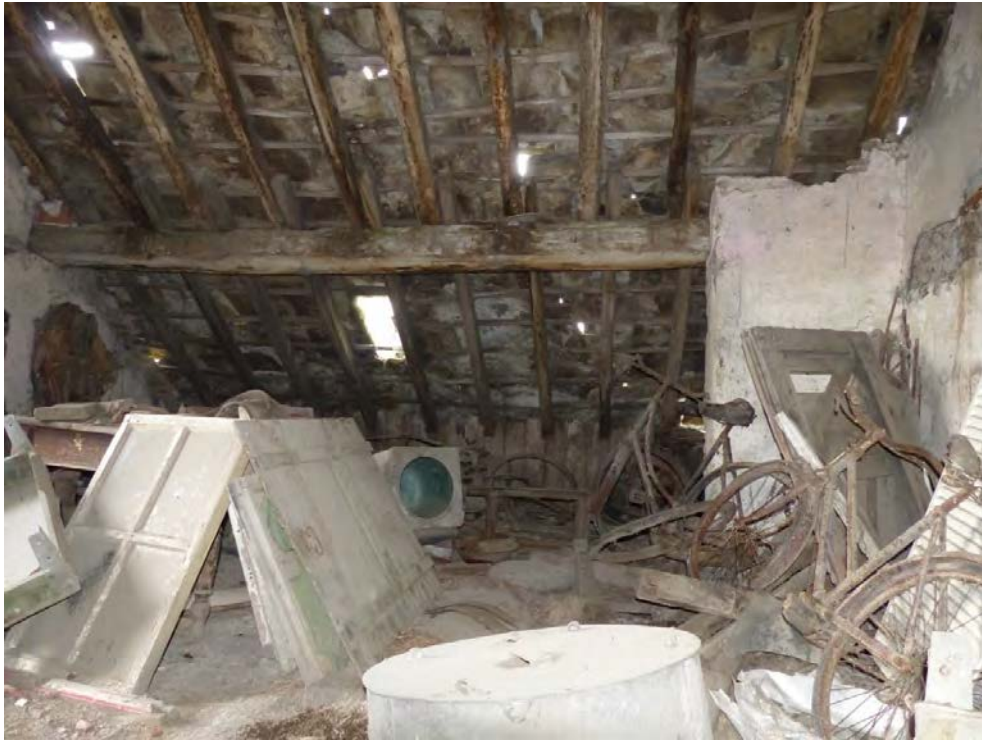
Plate 15: Bay 5 (Area F) looking west. Empty mortice holes on the underside of the tiebeam (above roof light)
