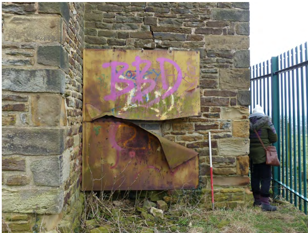
Plate 13: Detail view of blocked opening to north elevation of stair turret, looking south
