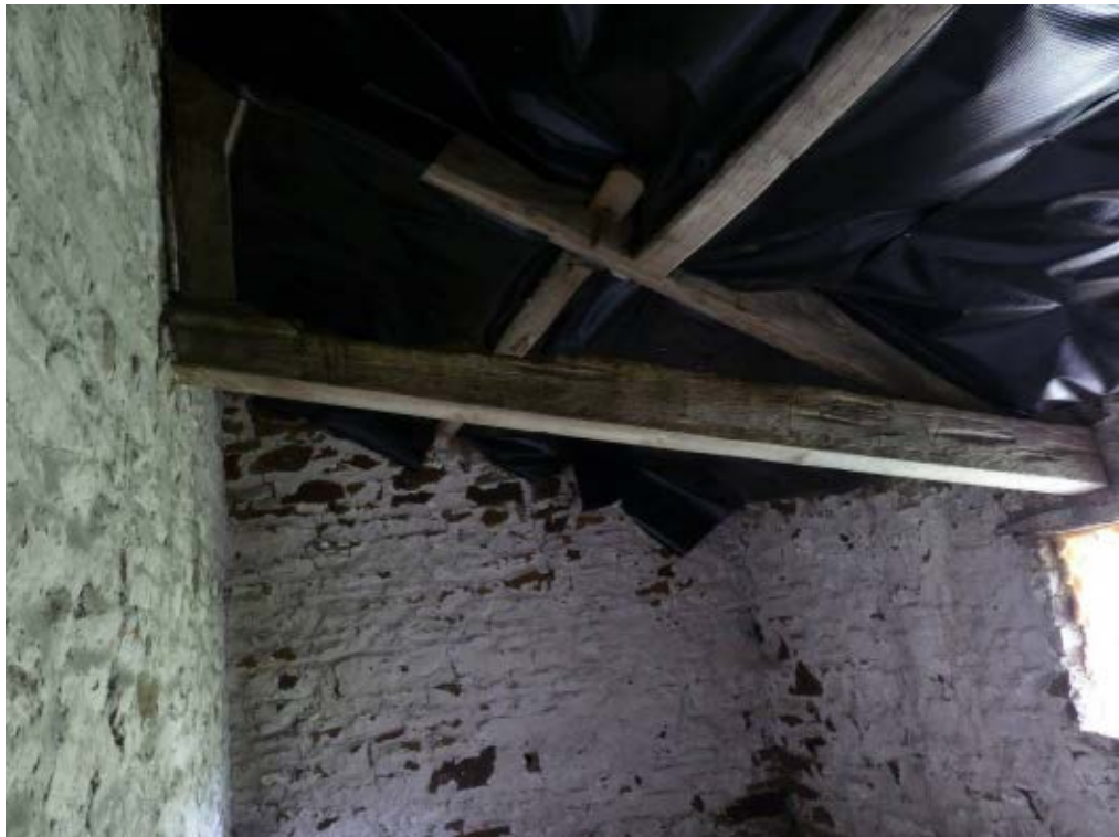
Plate 20: First floor of lean-to, merchant's marks are visible on the right of the tie beam, facing north
