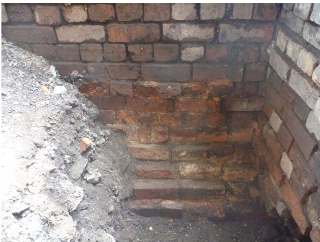
Plate 12: Detail of stepped out bricks at base of wall 129, viewed facing south
