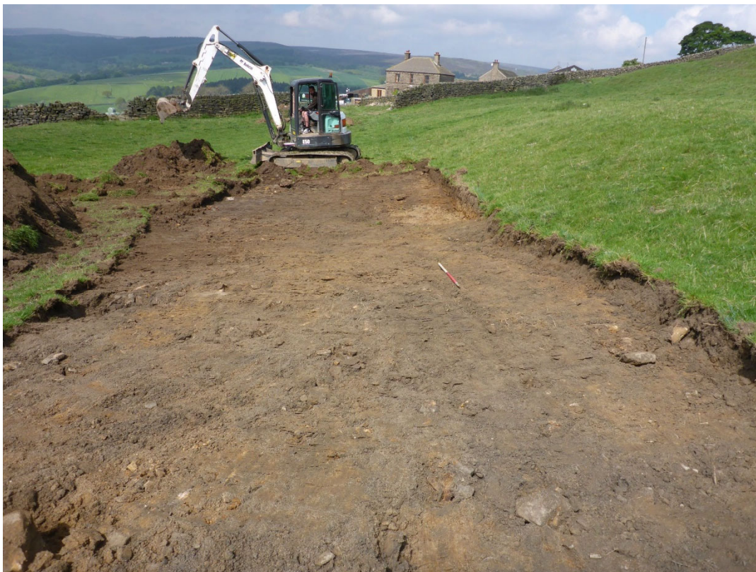
Plate 1: Stripping of easement in Field 2, showing low bank to the left, viewed facing west
