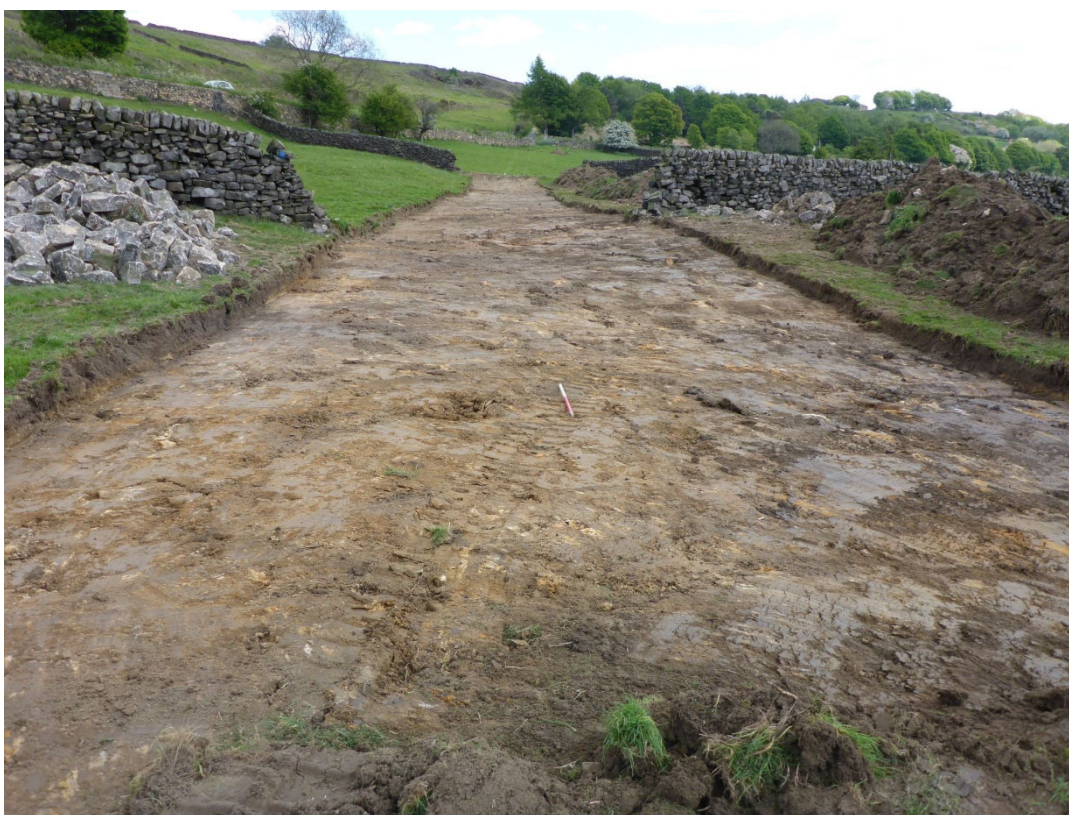
Plate 6: Stripped easement in Field 3, viewed facing east towards Field 2 (Note: scale in all photos in 50cm increments unless otherwise stated)
