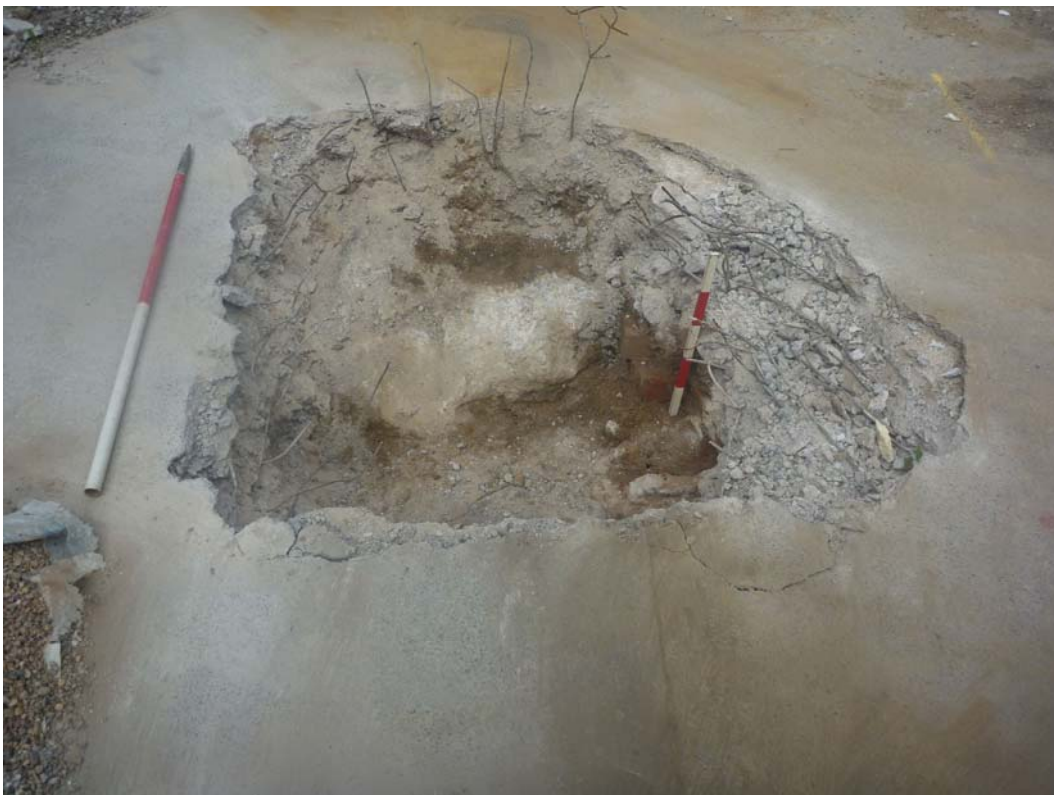
Plate 1: Trial pit at north end of Trench 1, showing concrete surface 101 and underlying concrete 109, viewed facing north (scales in 50cm and 10cm divisions)
