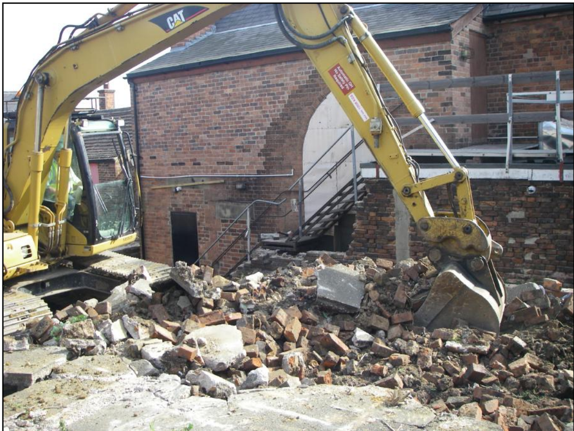
Plate 4: Removal of concrete platform and part of the boundary wall behind the Masonic Hall, Ilkeston.
