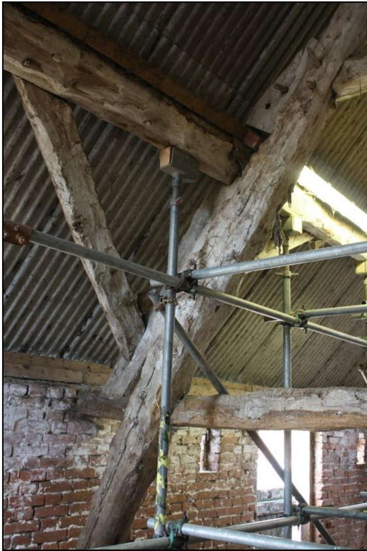
Plate 13: View of the centrally-placed cruck frame in the animal shed at Holywell Farm , showing upper and lower packing pieces behind the blade, with a brace halved lap jointed with the lower one.
