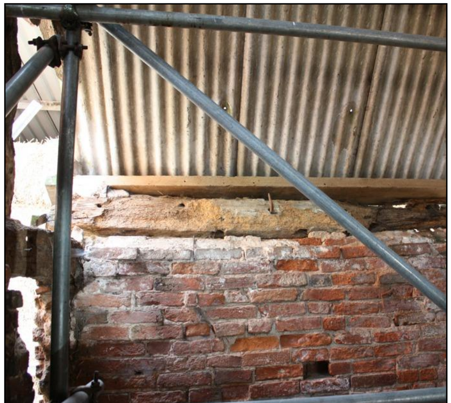
Plate 8: Part of the wall-plate resting on the south side brick wall with holes showing on its underside, indicating former timberwork beneath it. The plate rested on the tie-beam showing to left.
