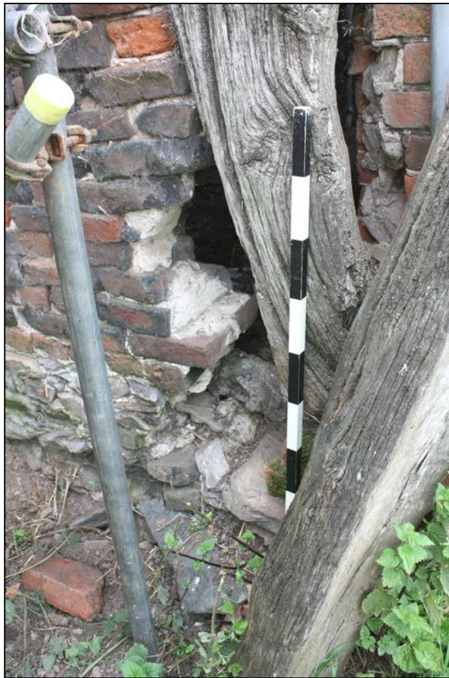
Plate 4: Rubble stone base and displaced base of cruck blade showing in the north-east corner of the building
