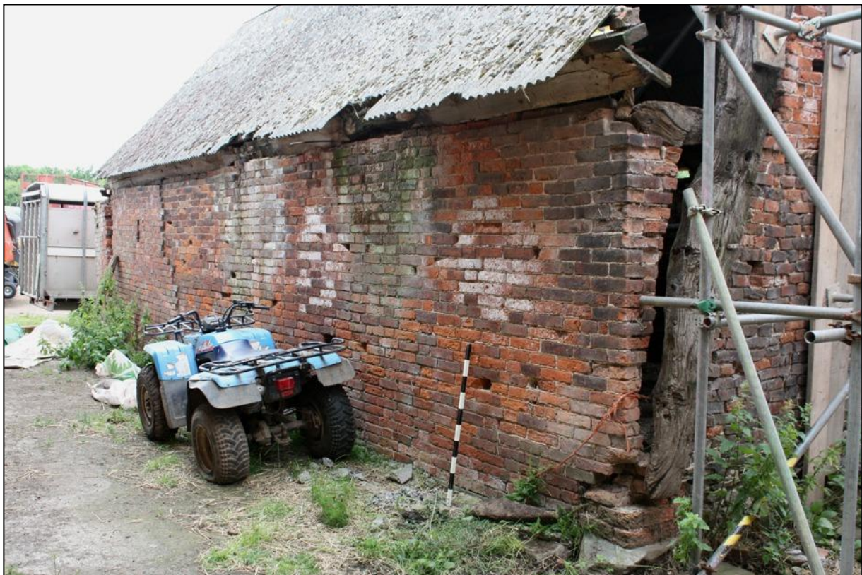
Plate 2: South side of the animal shed at Holywell Farm showing, to left, crack in the walling and, to right, the displaced south blade of the east-end cruck frame. The original wall-plate rests on top of the brick walling.
