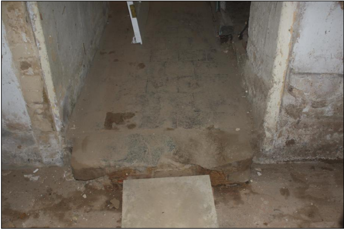
Plate 42: Possible threshold stone to what may have been an original south entrance into the Phase 2 building.
