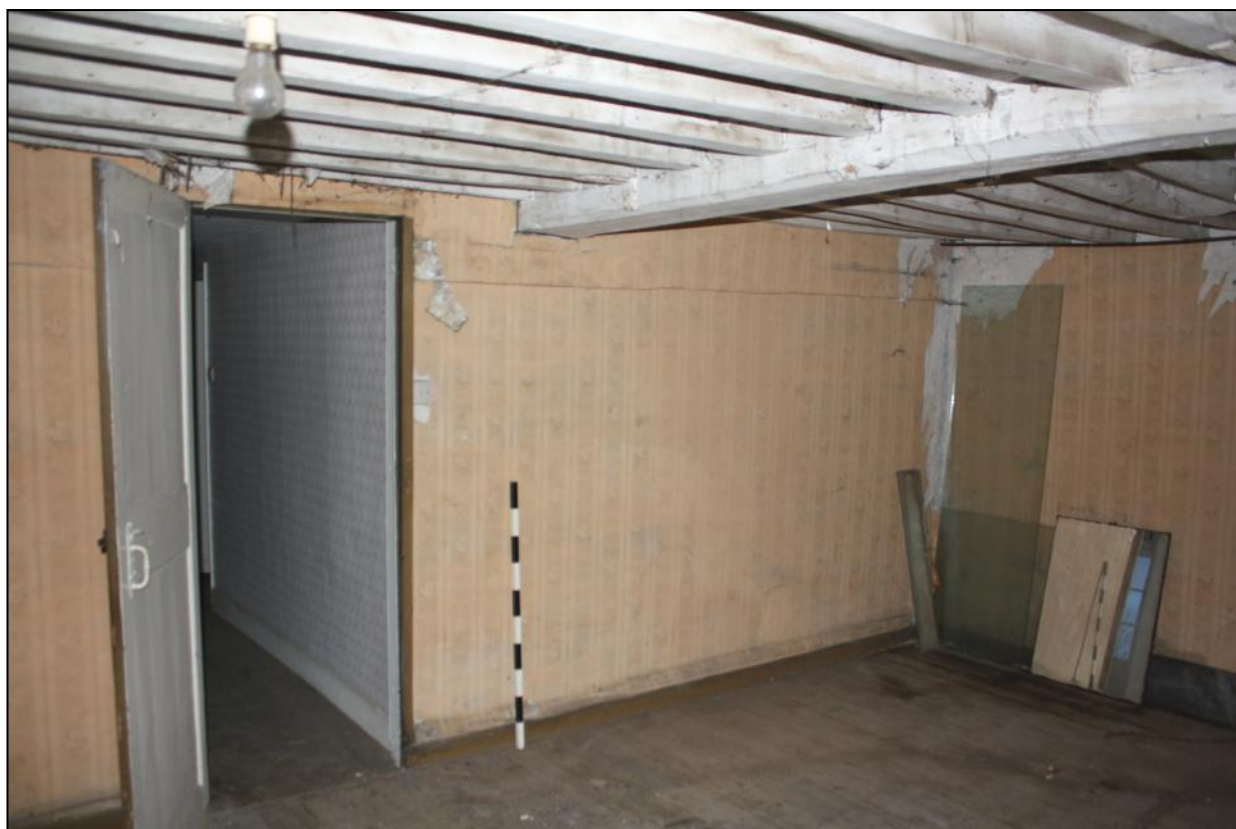
Plate 15: Timberwork in the ceiling and walling and a 2-panelled door in Bedroom 6.
