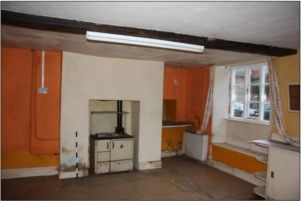
Plate 10: Existing kitchen in what is possibly the oldest part of Parkfield House, Belton-in-Rutland.
