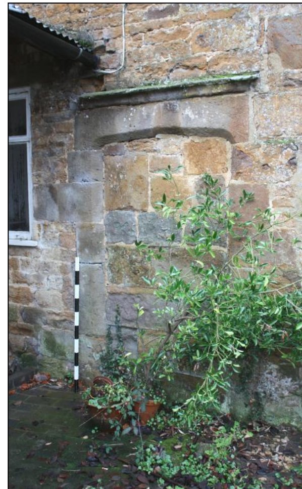
Plate 7: East side doorway to the through-passageway in the older part of Parkfield House.
