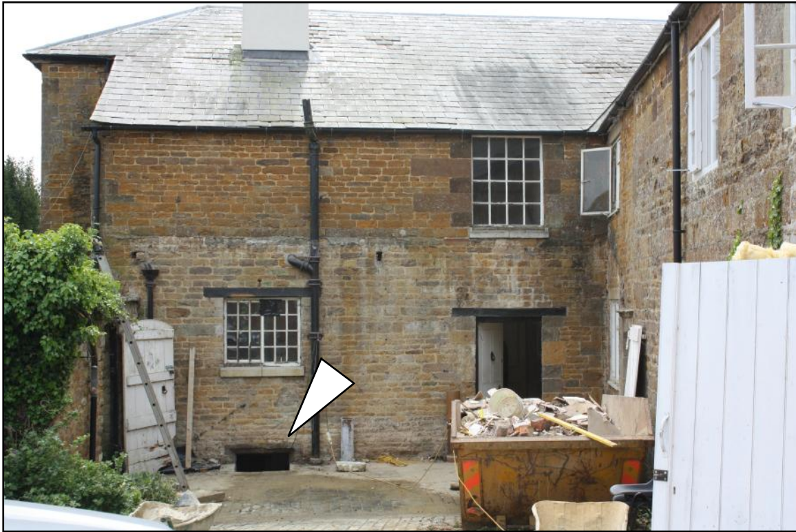
Plate 48: Back wall of the Phase 4 south wing service part, with former canopy removed and an arrow pointing to the position of a light-well to the cellar.
