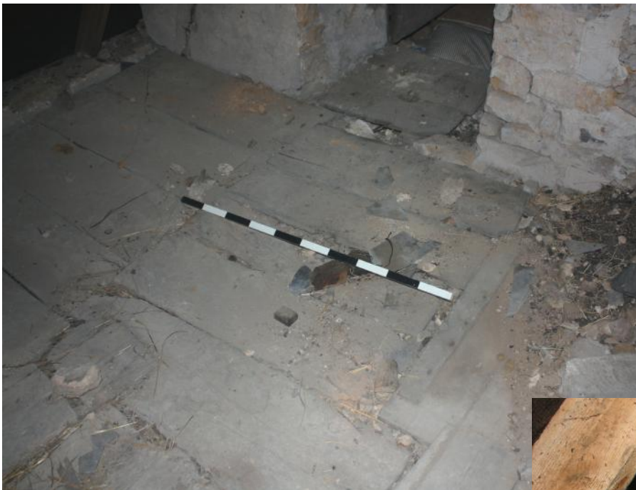
Plate 20: Possible former position of original stair(case) access into Attic 2 showing in floor near present entrance.
