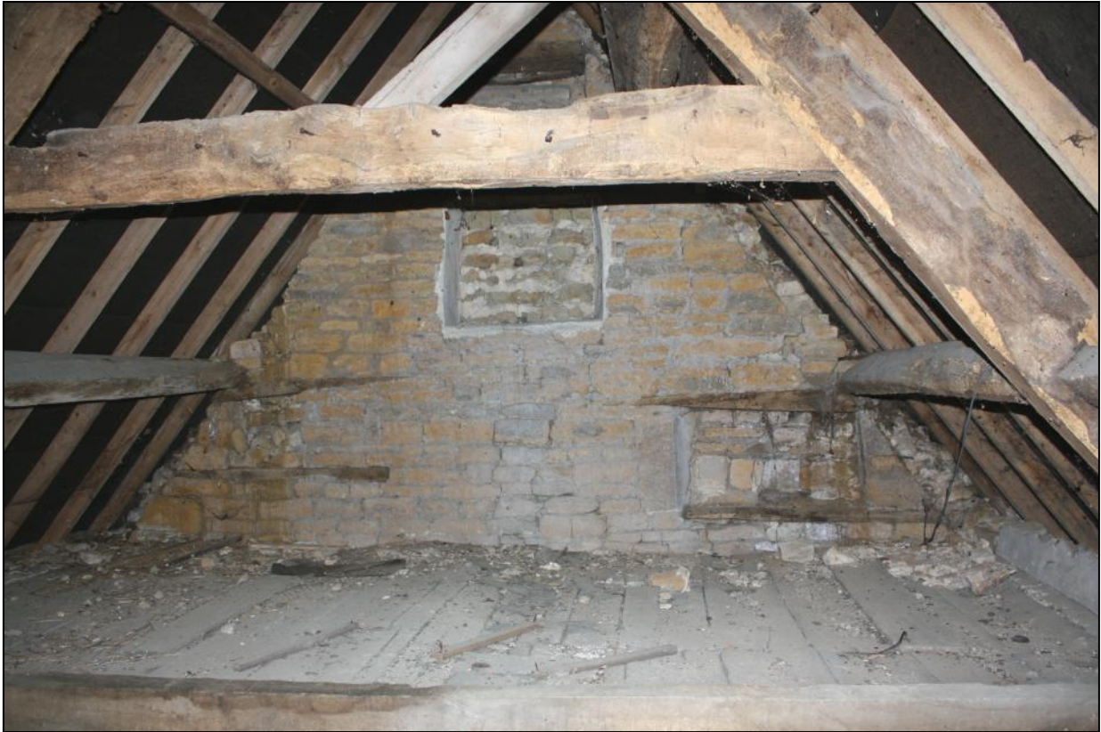
Plate 19: View towards north end gable wall in Attic 2 showing infilled garret window and two low cupboards.
