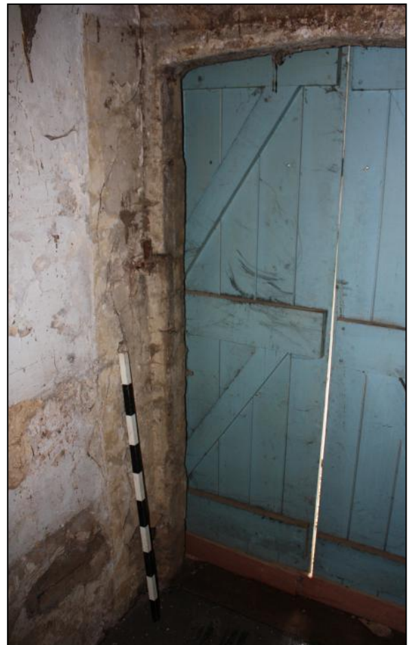
Plate 44: With infill removed from former east side entrance, no clear distinction showing between Phase 2 walling to left and Phase 3 entrance.
