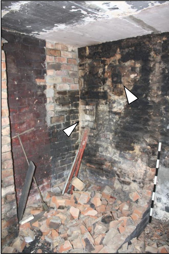
Plate 39: Removal of store doors and partitioning in former washroom revealing staining on the back wall from a former fireplace, an infilled cupboard and a wooden block (position highlighted by right arrow).
