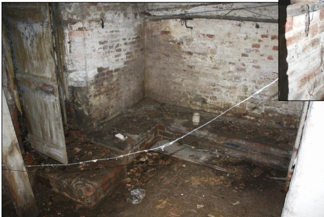
Plate 31: Brick-lined cellar with low thralls and former external entry (to left) beneath the present toilet. ▼
