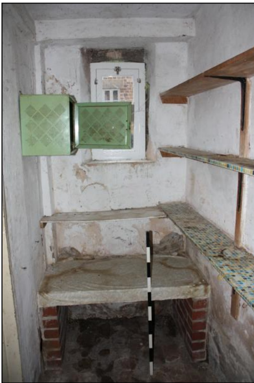
Plate 11: Pantry with thrall and shelves in the former through-passageway. Facing the infilled former front doorway.
