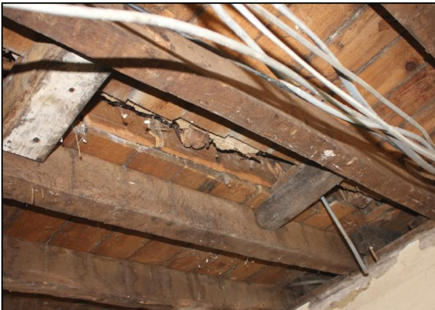
Plate 46: An irregular break between the floor planking showing where there is a first floor corridor partition above.
