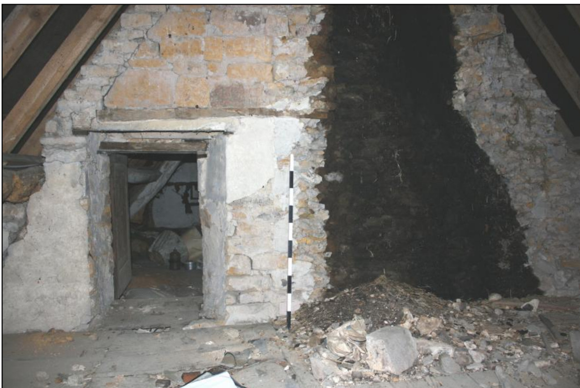
Plate 18: View of the same wall as above, as seen from Attic 2, with small entrance and part of exposed chimney flue.
