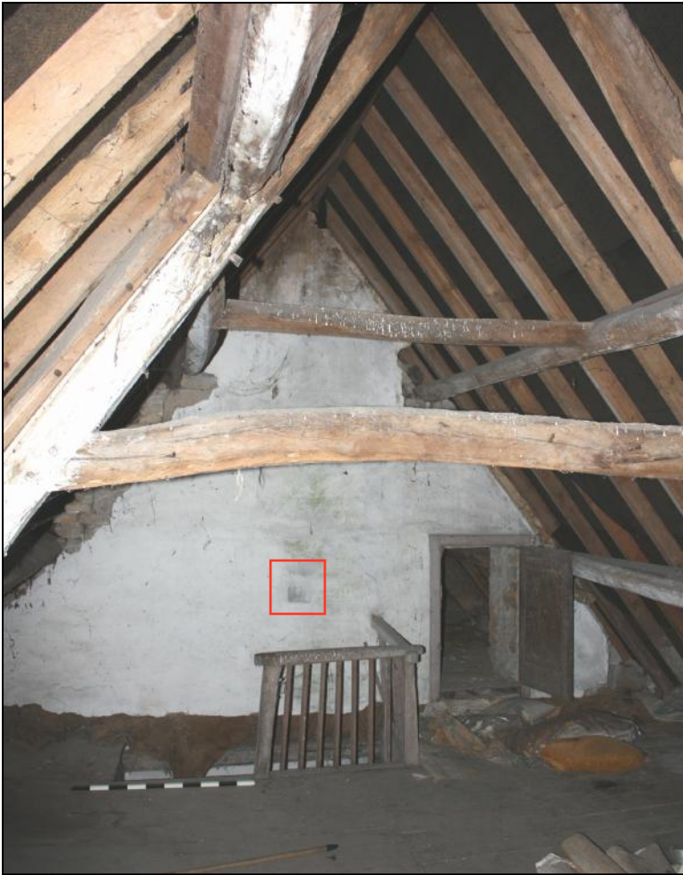
Plate 16: View inside Attic 1 looking towards the north wall with staircase and, highlighted, a timber showing in the walling, possibly a former ridge-plate.
