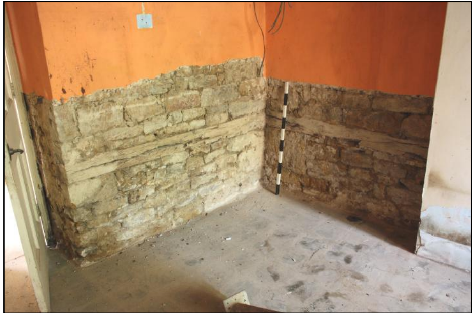
Plate 45: Timber plates showing in the south end walling of the Phase 3 former kitchen.
