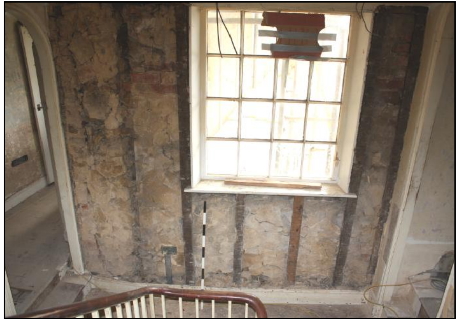
Plate 50: Exposed stone walling at the first floor back wall of the Phase 4 south wing service part showing rough stone finish and vertical studs for support of former plasterwork.
