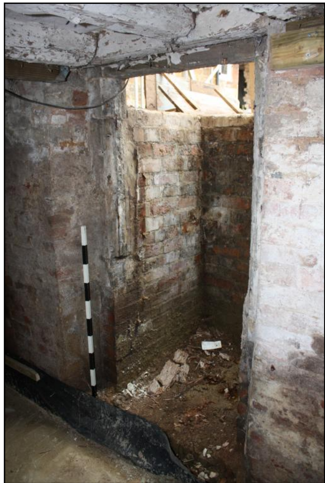
Plate 49: Light-well seen from inside the cellar, showing external brick surround and reused moulded stonework edging the window opening.
