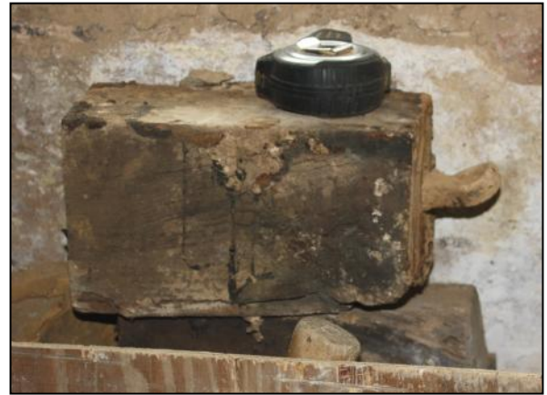
Plate 40: Wooden block removed from former fireplace walling prior to a new doorway being created.
