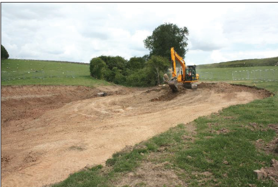
Plate 9: View back along length of former stream with depression for lagoon being excavated.
