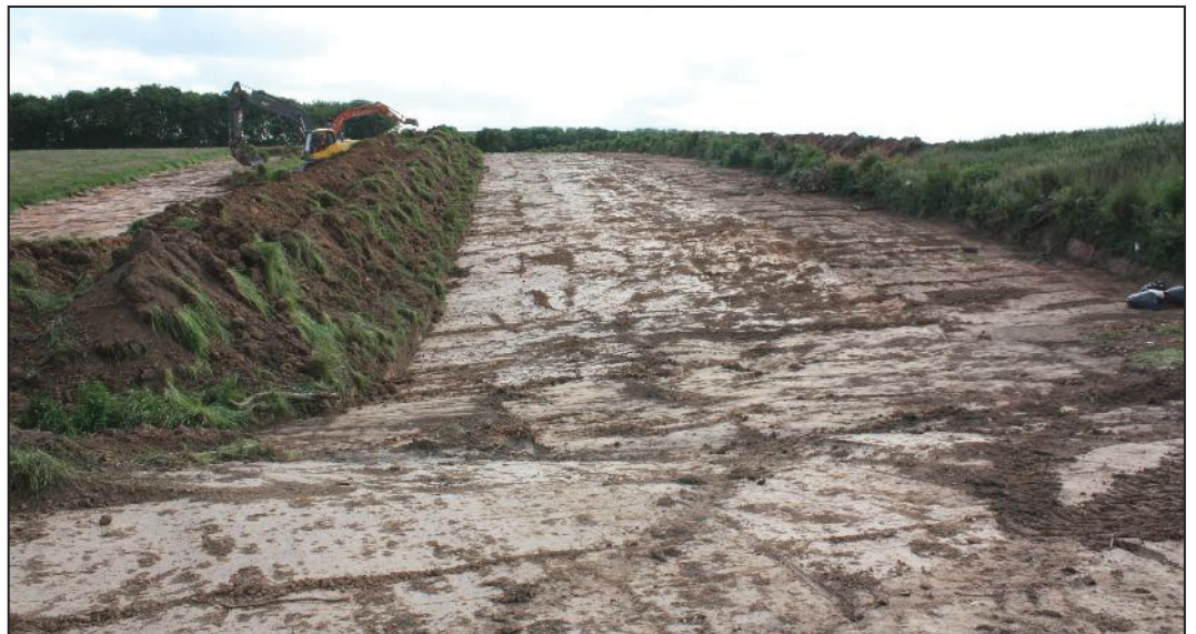
Plate 2: View of one of the long strips running uphill with topsoil having been stripped off.
