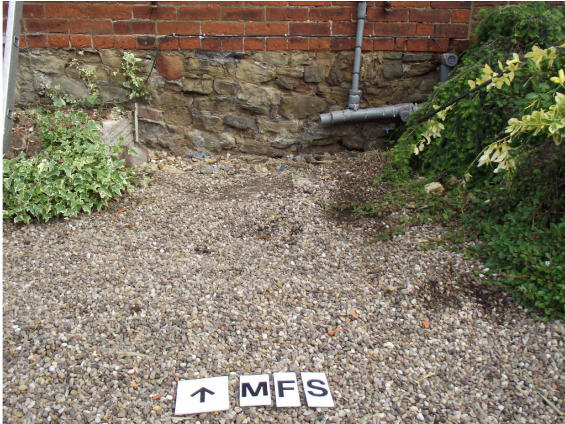
PLATE 2. The low stone foundation, 0005, in part of the south wall of the demolished extension. Looking north.
