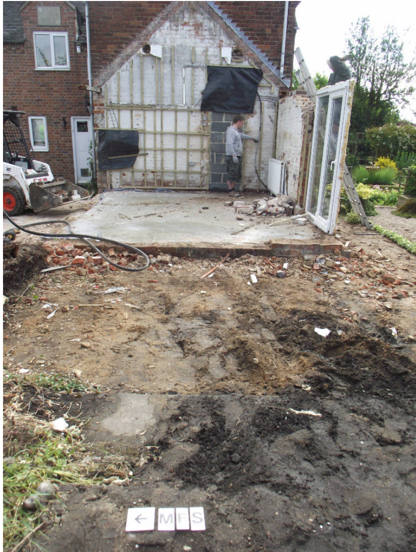
PLATE 1. Area 01 with modern extension in the process of demolition. The concrete slab, 0001 can be seen on the background and 0002 and 0003 in the mid and foreground respectively. Looking east.
