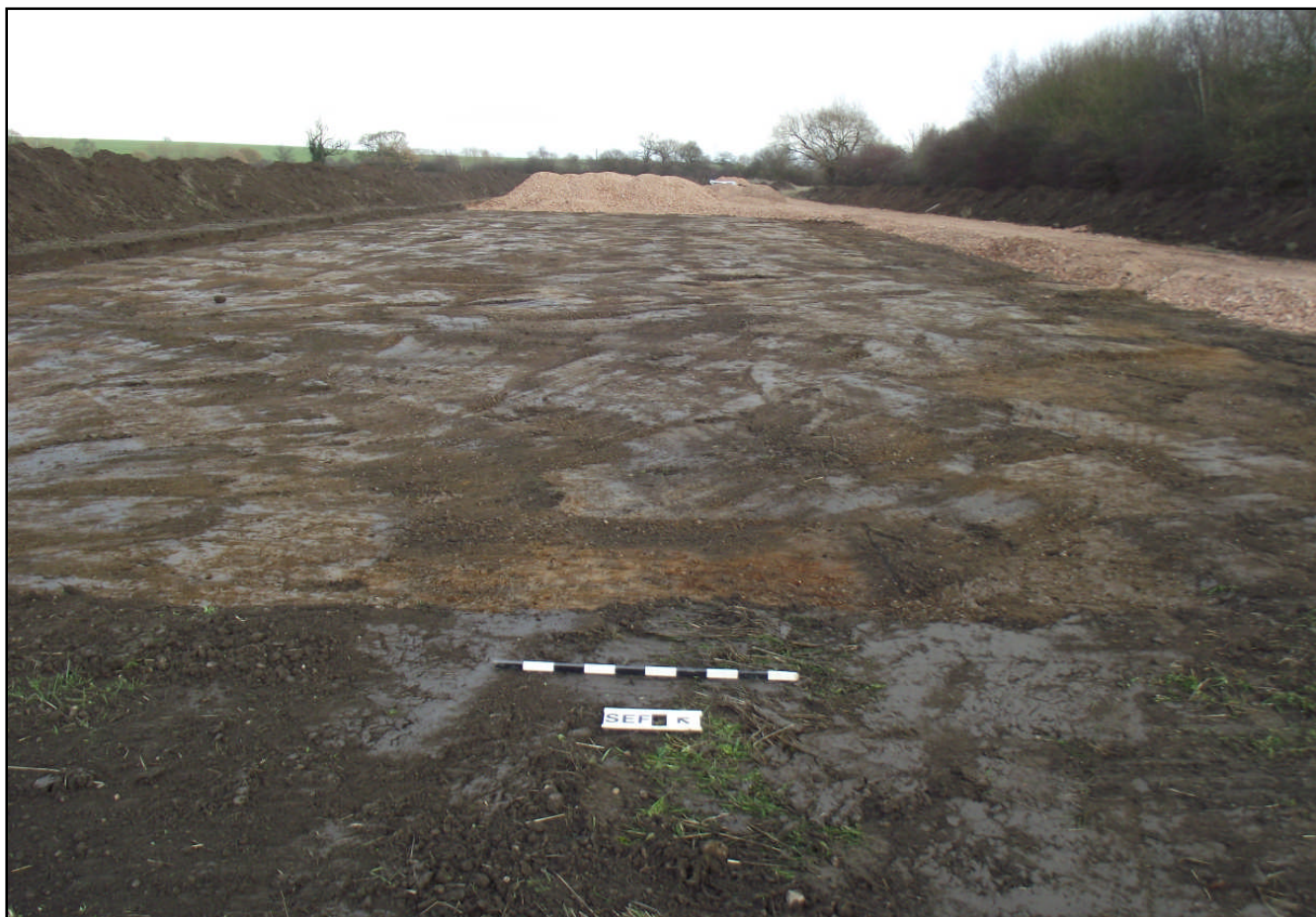
Plate 5: Area 04, Topsoil strip for the proposed construction of the pullet rearing Building, Looking East
