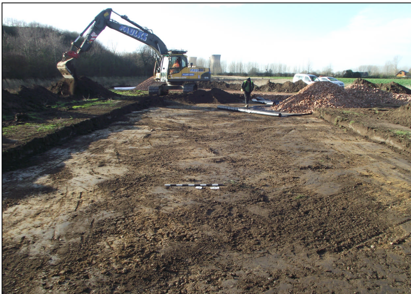
Plate 4: Area 03, Topsoil strip for the proposed construction of the mobile home platform, Looking West
