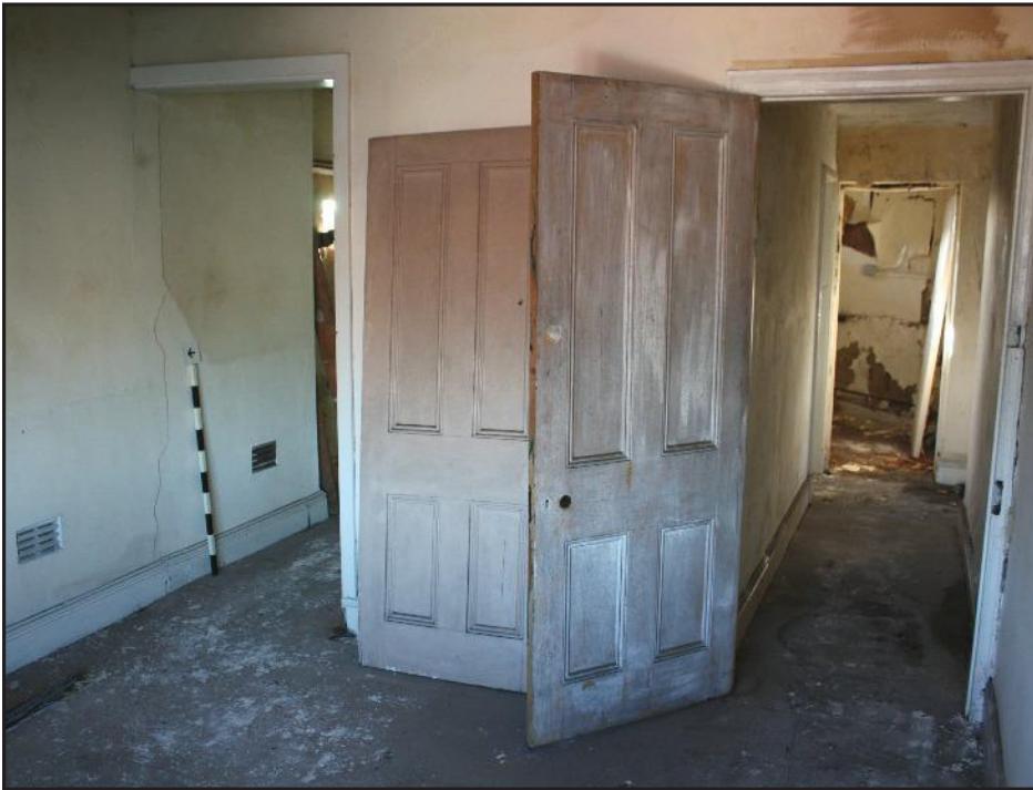
Plate 13: View on the first floor from Room 7 showing corridor and, to left, where part of the walling was removed for a doorway into Room 8. 1m scale shown.
