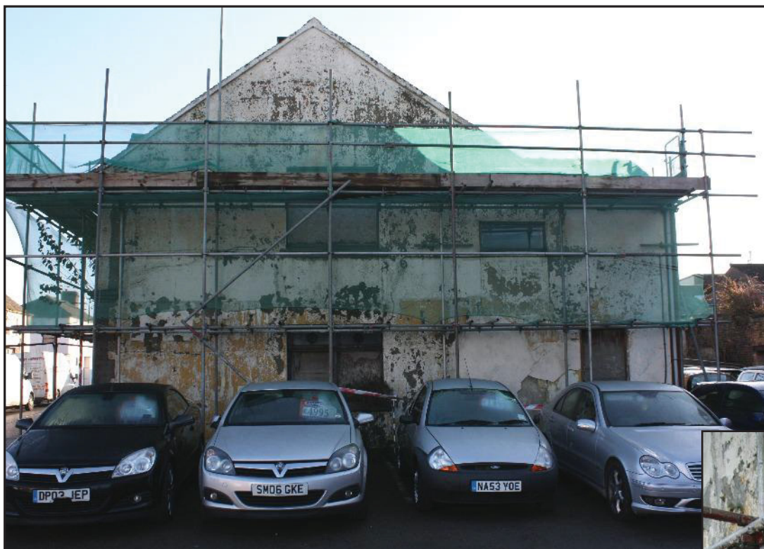
Plate 5: West elevation of 124 Uttoxeter Road, Longton, with shortened end to right - compare with Plate 2. 1m scale shown.
