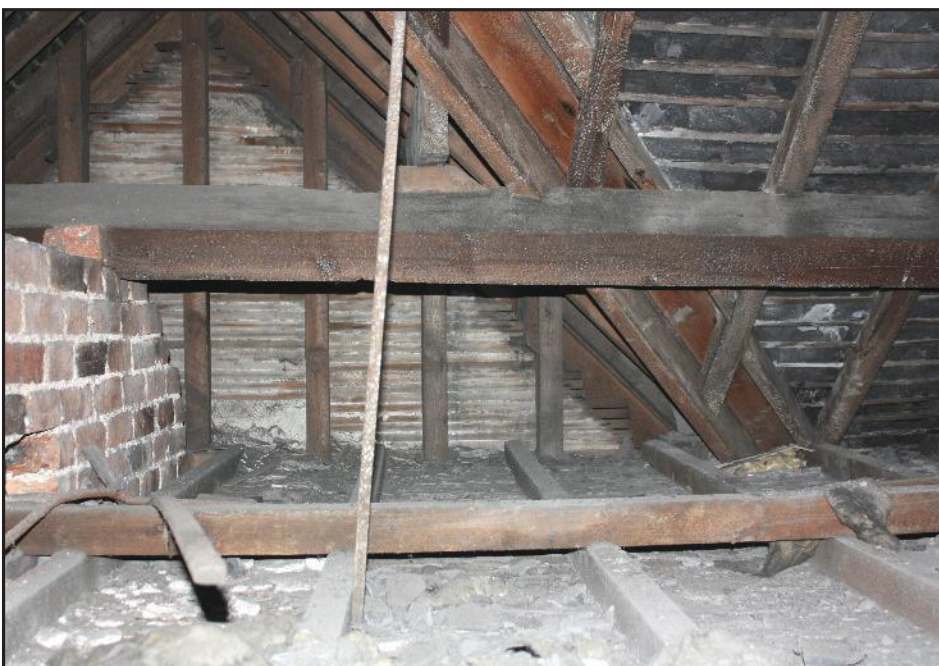
Plate 15: View of attic showing stack brickwork and timberwork at the front of the building.
