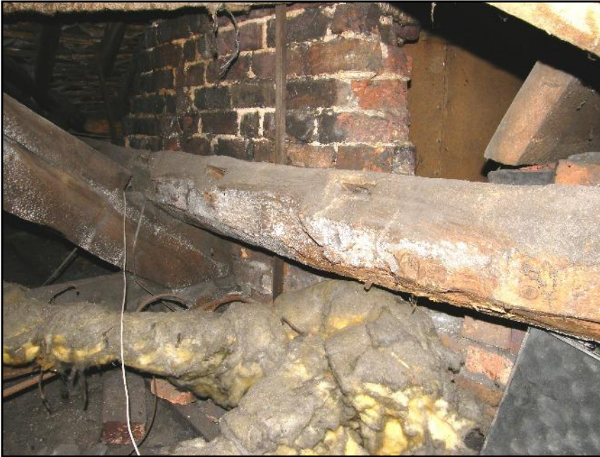
Plate 21: South Roof, north lower purlin with empty mortice holes indicating it is a reused timber, viewed looking north-west.
