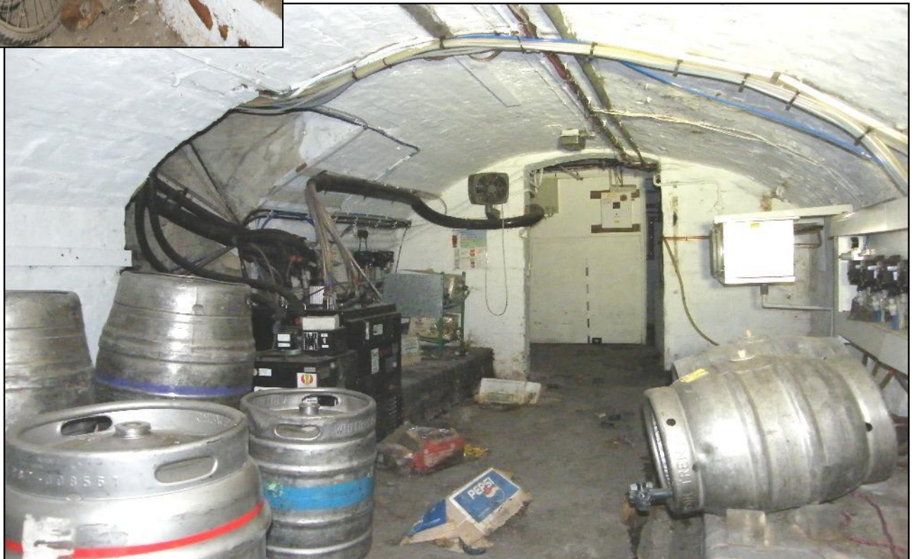
Plate 17: View of Cellar 1, looking towards Cellar 2, with former entrance showing to left, behind barrels.
