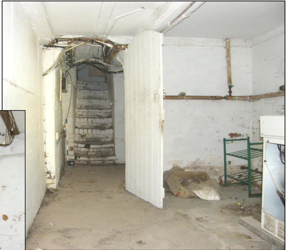
Plate 15: View of the Cellar 2 looking towards current staircase, and showing ceiling beams.
