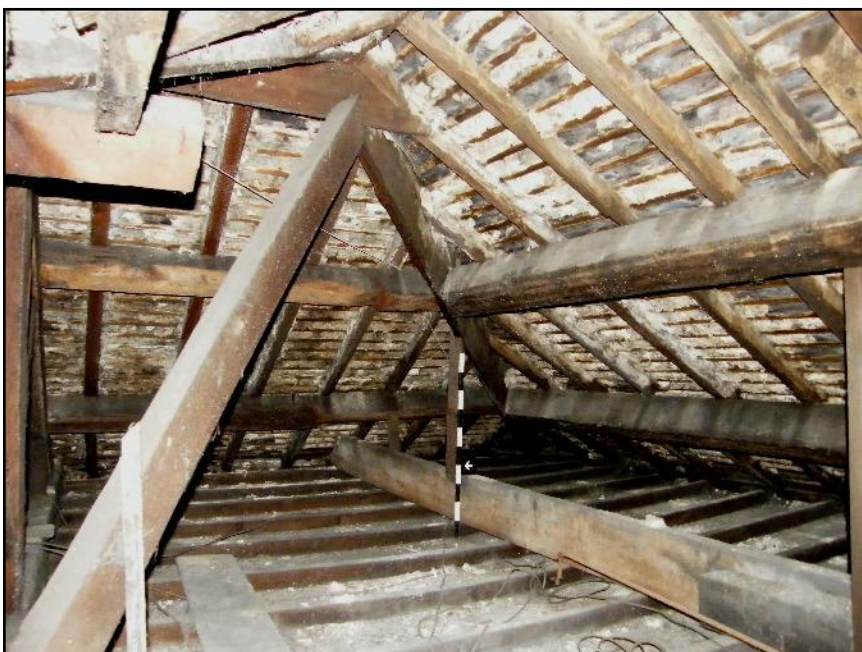
Plate 23: East Roof, with the hip rafter in the background and the timber support for the ridge and hip rafter in the foreground, viewed looking south-east.
