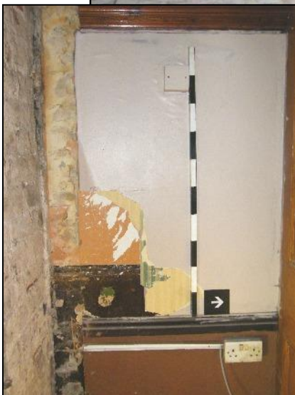
Plate 7: Evidence of a former decorative scheme revealed next to where the kitchen range used to be.
