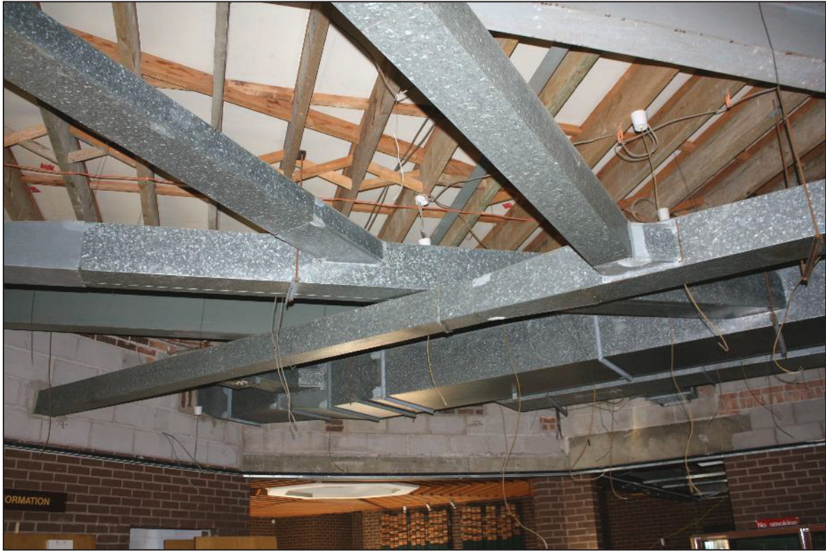
Plate 21: Area above the ceiling of the enquiry area showing upper blockwork and brick construction and a complex of ducts, cables, straps and the timber super-structure beneath the roof covering.
