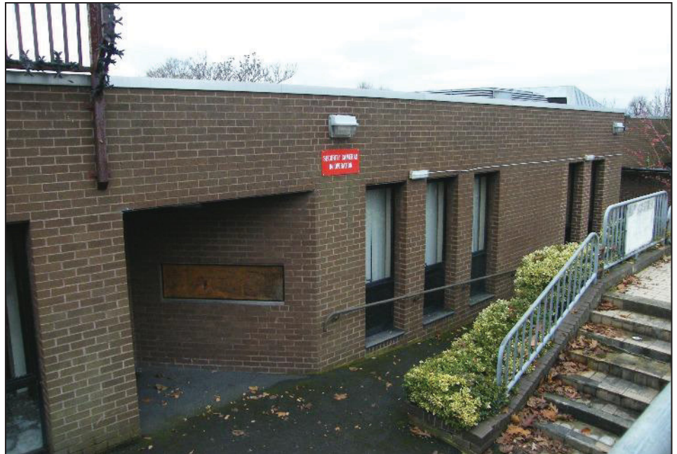
Plate 4: Brickwork facade around one of the non-public entrances off New Lawn Road.
