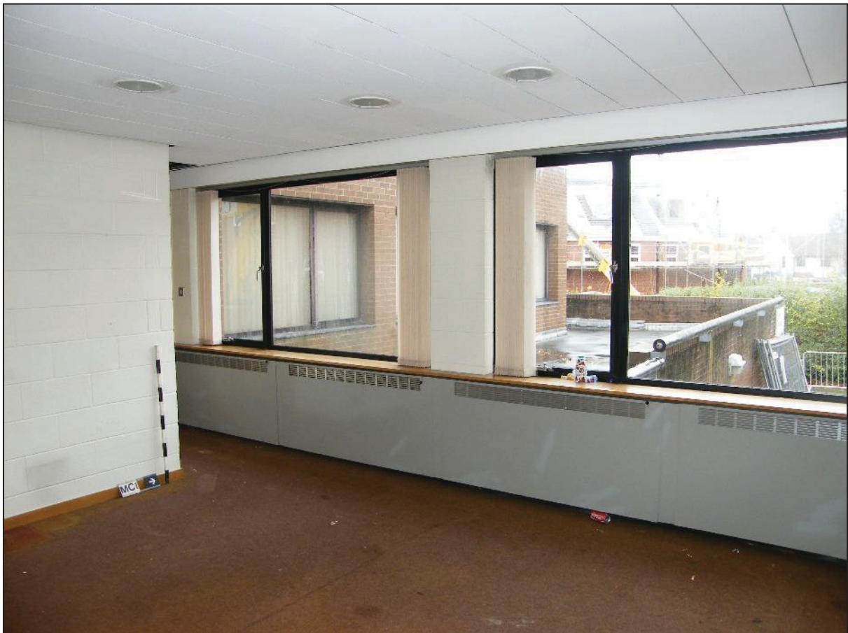
Plate 14: Well-lit and raised area at the north end of the building reserved for attending magistrates.
