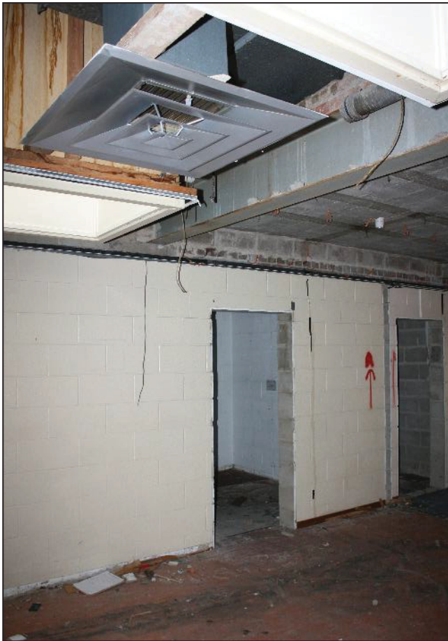
Plate 22: Cafeteria area with ceiling removed (showing as dark line) and tall upper structure and lighting revealed.
