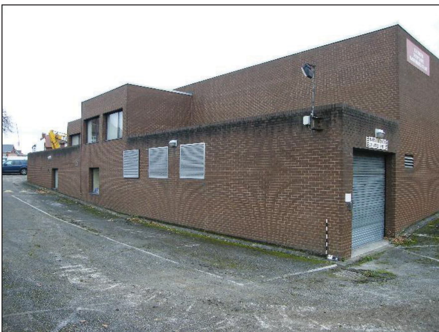
Plate 5: Austere brickwork showing at the north end of the Court House. The steel shutters are at the entrance to the prisoner's van dock.
