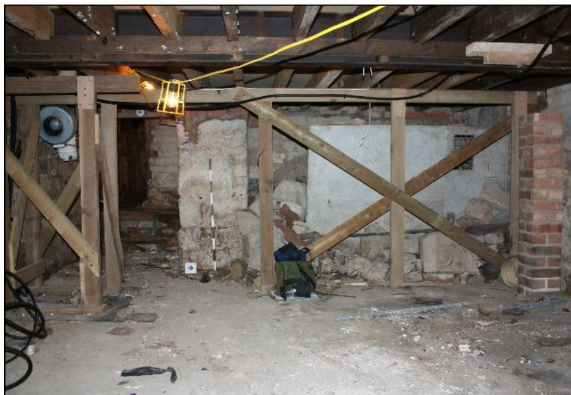
Plate 12: View of the west end of Cellar 1 showing stone pillar and, to right, possible position of former stairway entrance.
