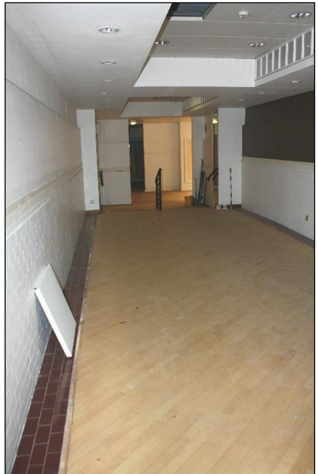
Plate 9: Ground floor area at back of No. 201A High Street (unit J) looking east and showing skylight.
