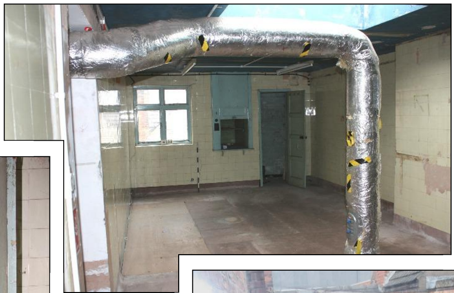
Plate 35: View looking westwards at the second floor level of unit F, showing lift and entry to water-tower.
