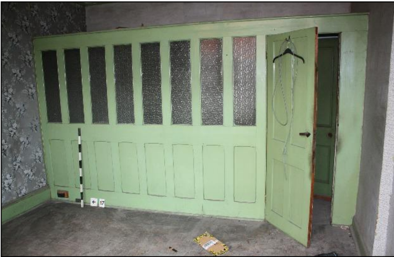
Plate 29: Panelling hiding an added stairway to the first floor room in unit H.
