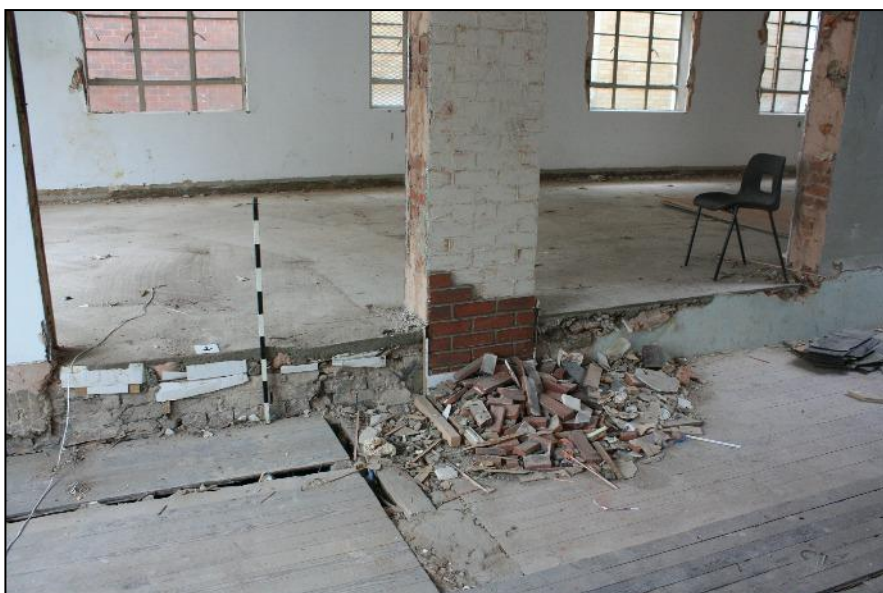
Plate 24: Brickwork exposed in first floor dividing wall between Nos. 200 and 201 High Street.
