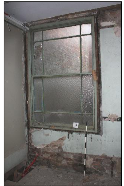
Plate 23: Sash window in west wall of unit E exposed during soft strip.
