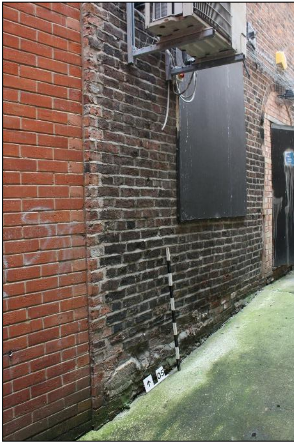
Plate 4: West end of unit A with altered brickwork indicating that it once extended further to the west.
