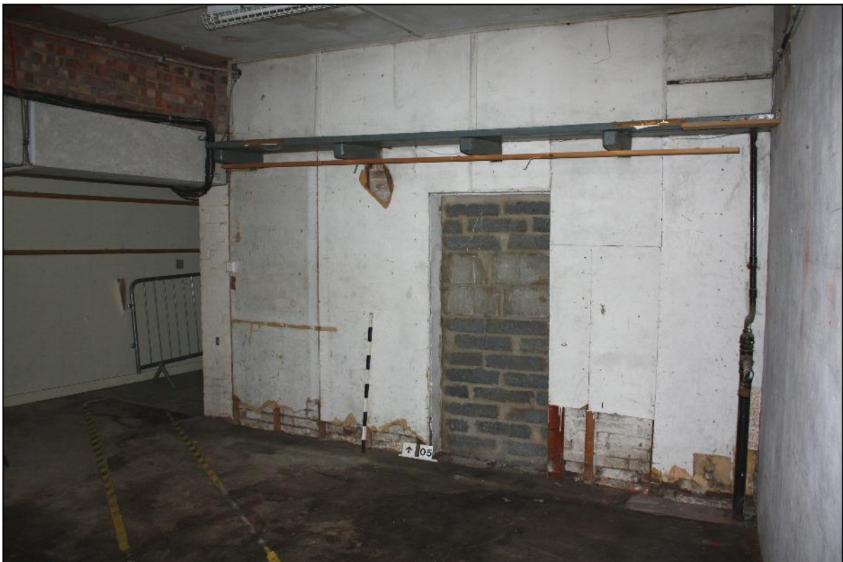
Plate 10: Back wall to unit A in No. 200 High Street, showing blocked doorway, exposed brickwork and removed west wall.
