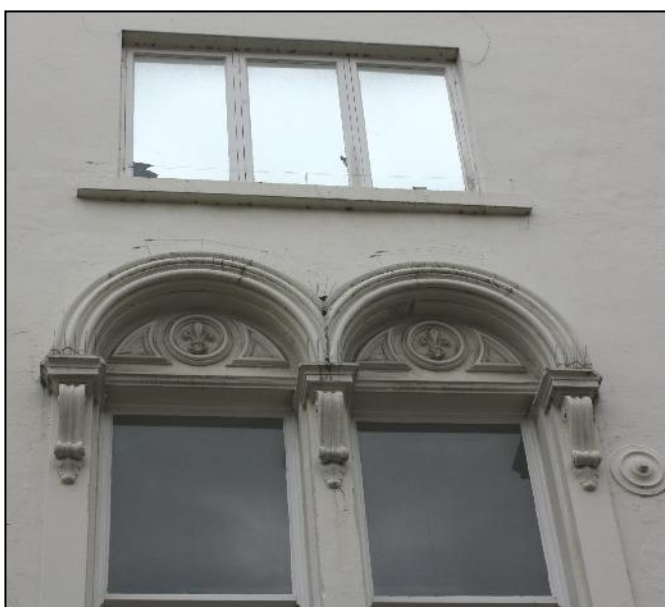
Plate 2: Detail of highly ornamental window head at one level and plain window above.
