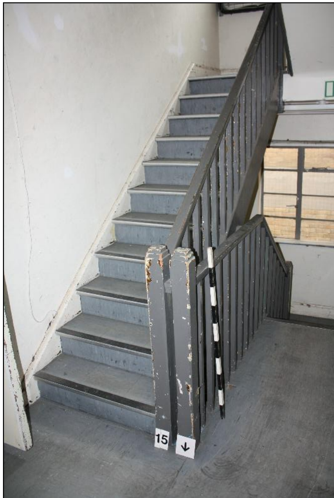
Plate 28: Staircase positioned in unit C, giving access from outside alley to three floor levels of No. 200 High Street.
