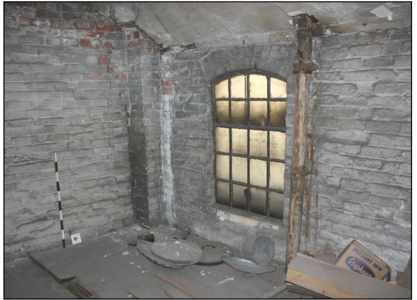
Plate 26: South-east corner of unit B, upper level, with brick-lined flue and iron-framed window.
