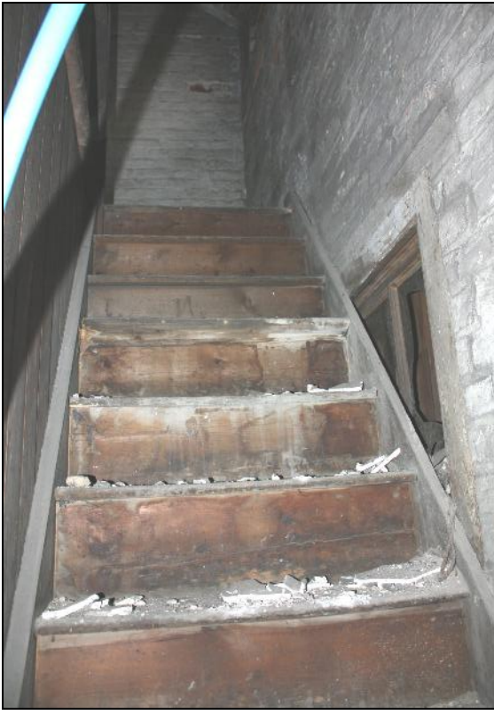
Plate 25: Blocked-off staircase to added upper level of unit B, No. 200 High Street with obscured sash window showing far right.
