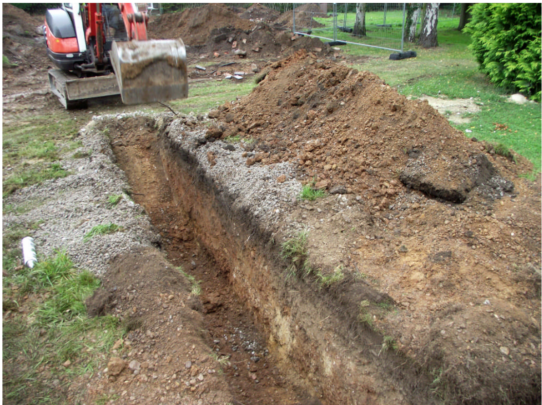
Plate 6. South facing section of Area 12 with top soil, 0001, lying directly over the natural sand and gravel, 0002 and 0003. Looking north west.
