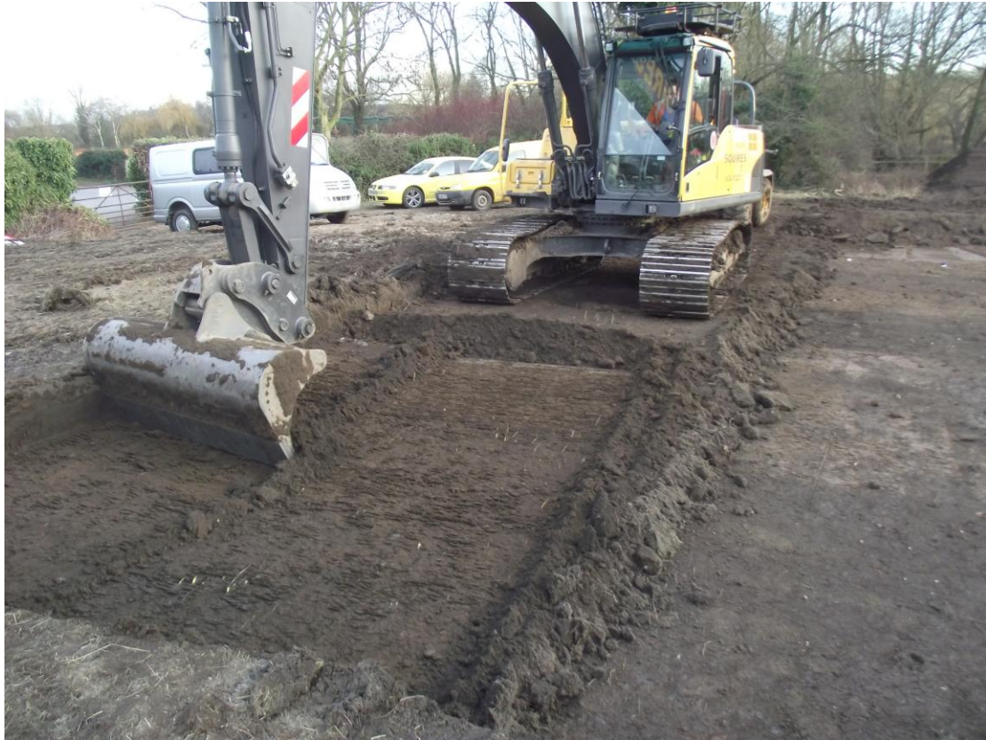
Plate 9. Soil stripping at the north east end of the site. Looking south east.
