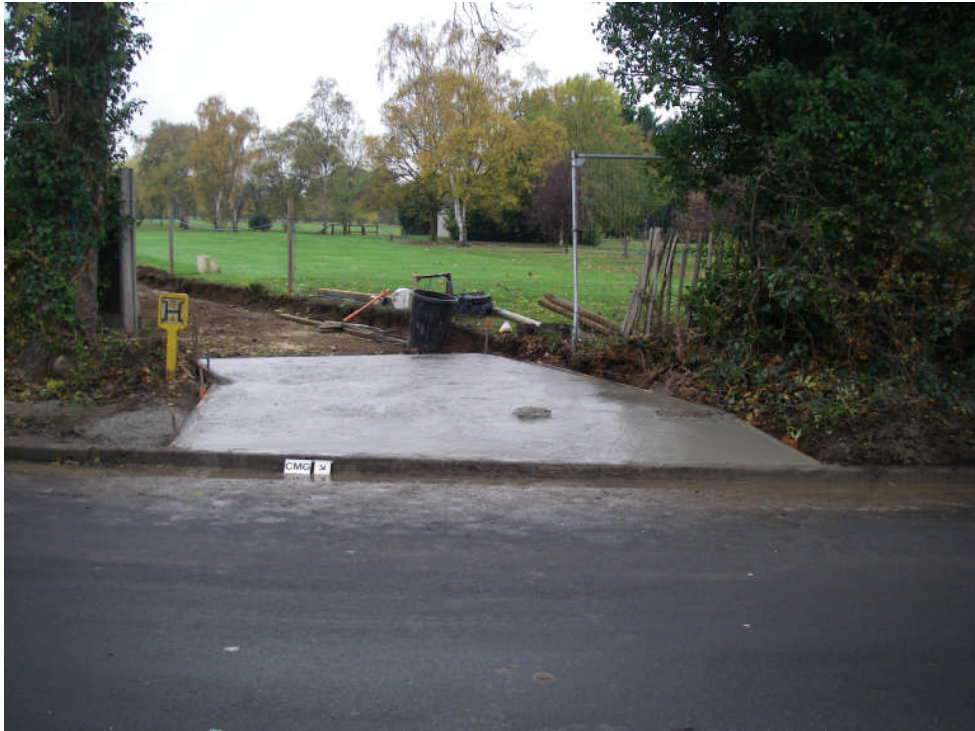
Plate 9. Concrete access ramp constructed after topsoil strip at meadow lane entrance. Looking south west.
