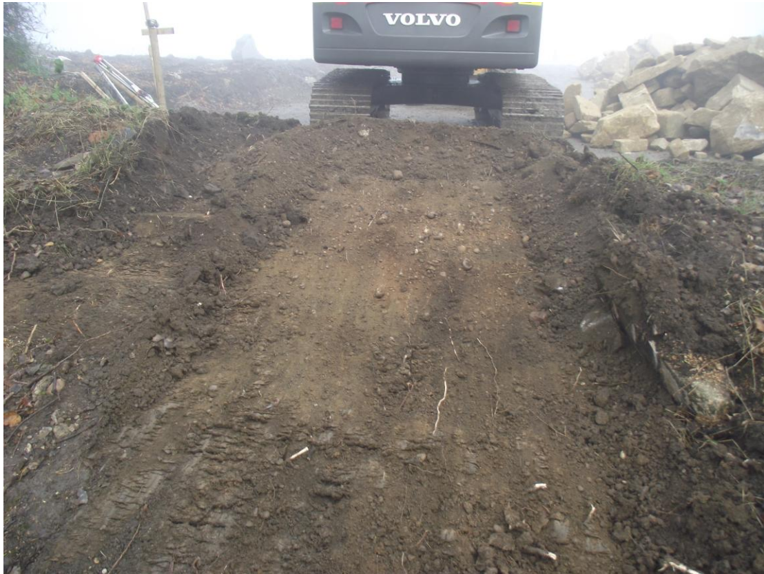
PLATE 4. Excavating through the river bank to provide a smooth surface. Looking north east.
