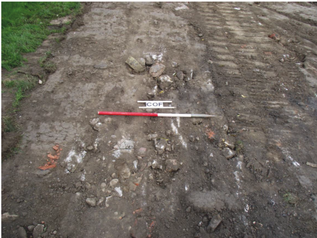
PLATE 4. detail of rubble directly beneath the topsoil on the flood defence in Area 02.
