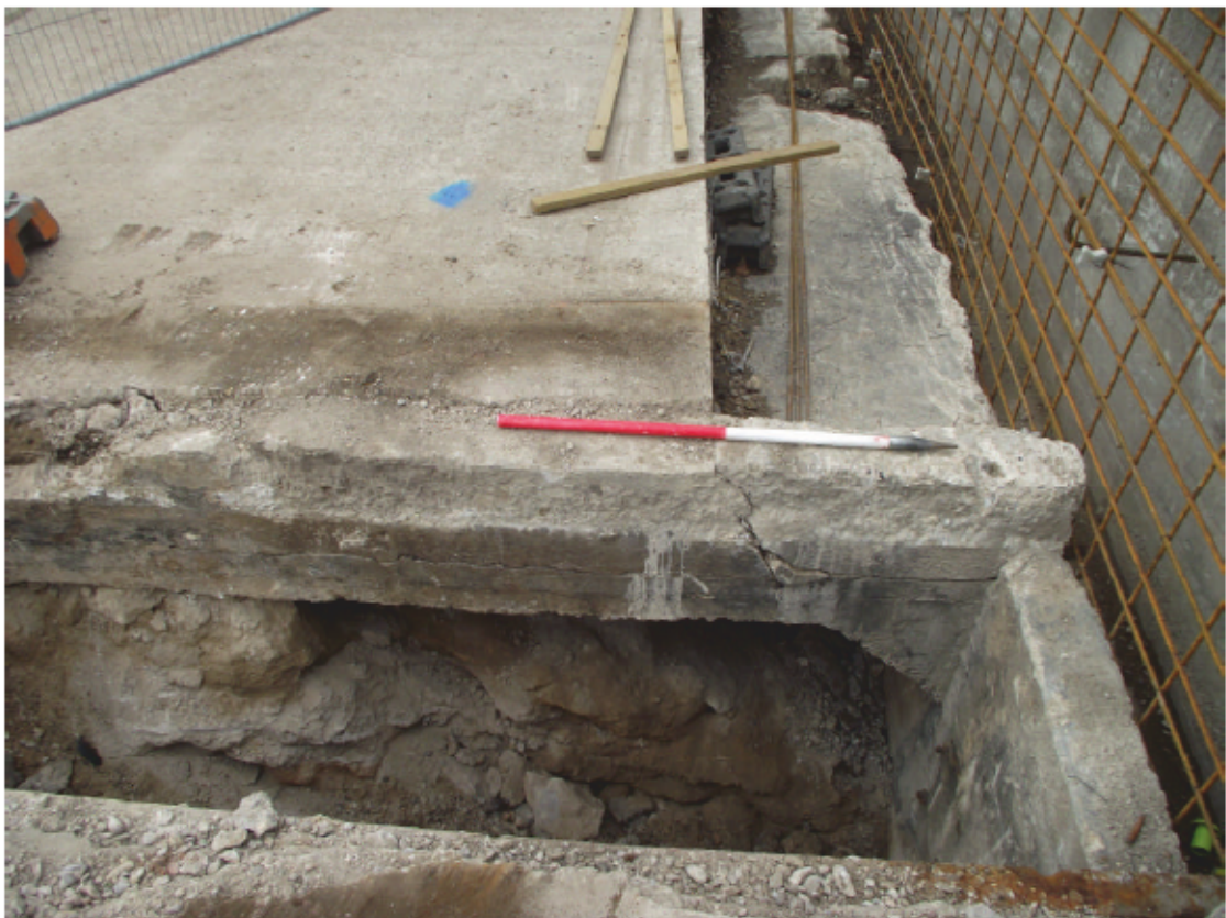
PLATE 2. Partially exposed entrance to the chamber. The original upper surface is immediately below the scale with the newer surface above.
