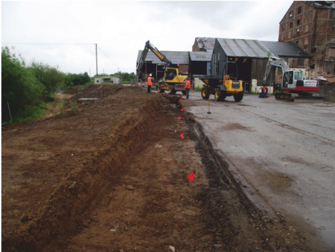
PLATE 5. Topsoil stripping on the edge of the existing flood defence in Area 03. Looking south-east.
