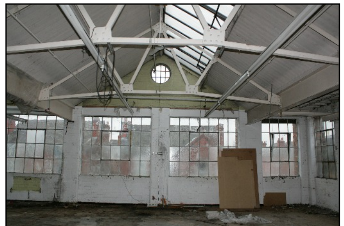
Plate 15: The roof trusses used on the first floor of Phase F, viewed looking west.
