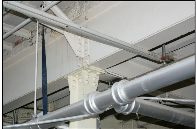
Plate 13: Detail of the roof truss, steel post and plate in the single storey range in Phase F.
