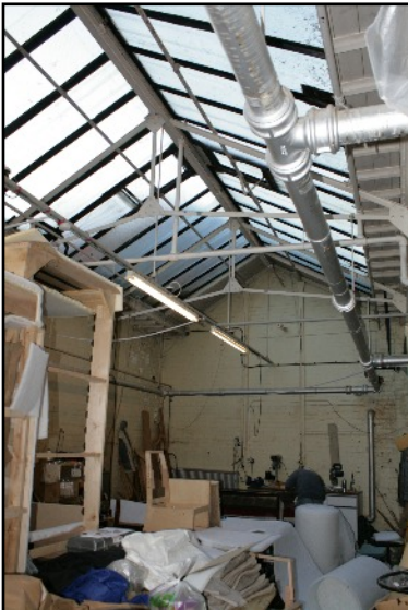
Plate 12: The single storey glass range in Phase F range viewed looking south-east.
