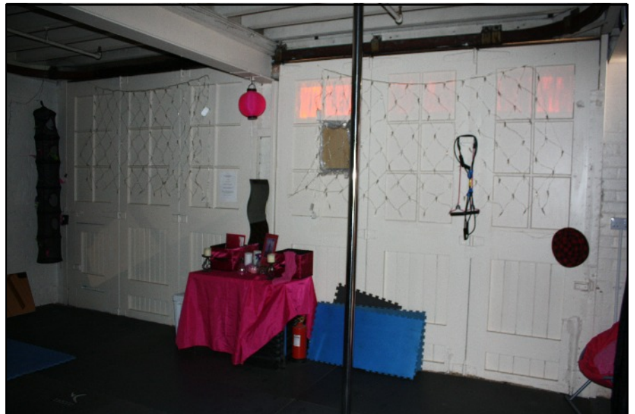
Plate 9: Interior of the dispatch building (Phase E) showing the original doors behind the bricked in entrances of the west wall, viewed looking south-west.
