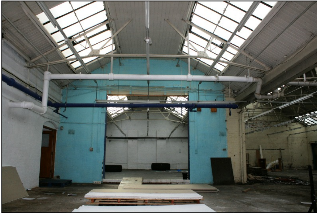
Plate 16: General view of the eastern most range of Phase F1, viewed looking south.
