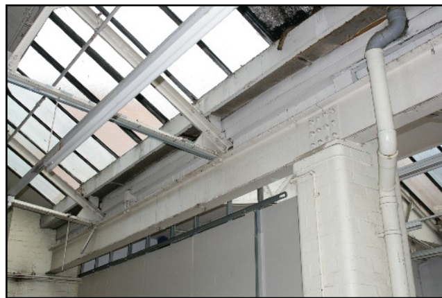
Plate 17: Detail of the roof truss, steel plate and brick posts in the eastern range of Phase F1.
