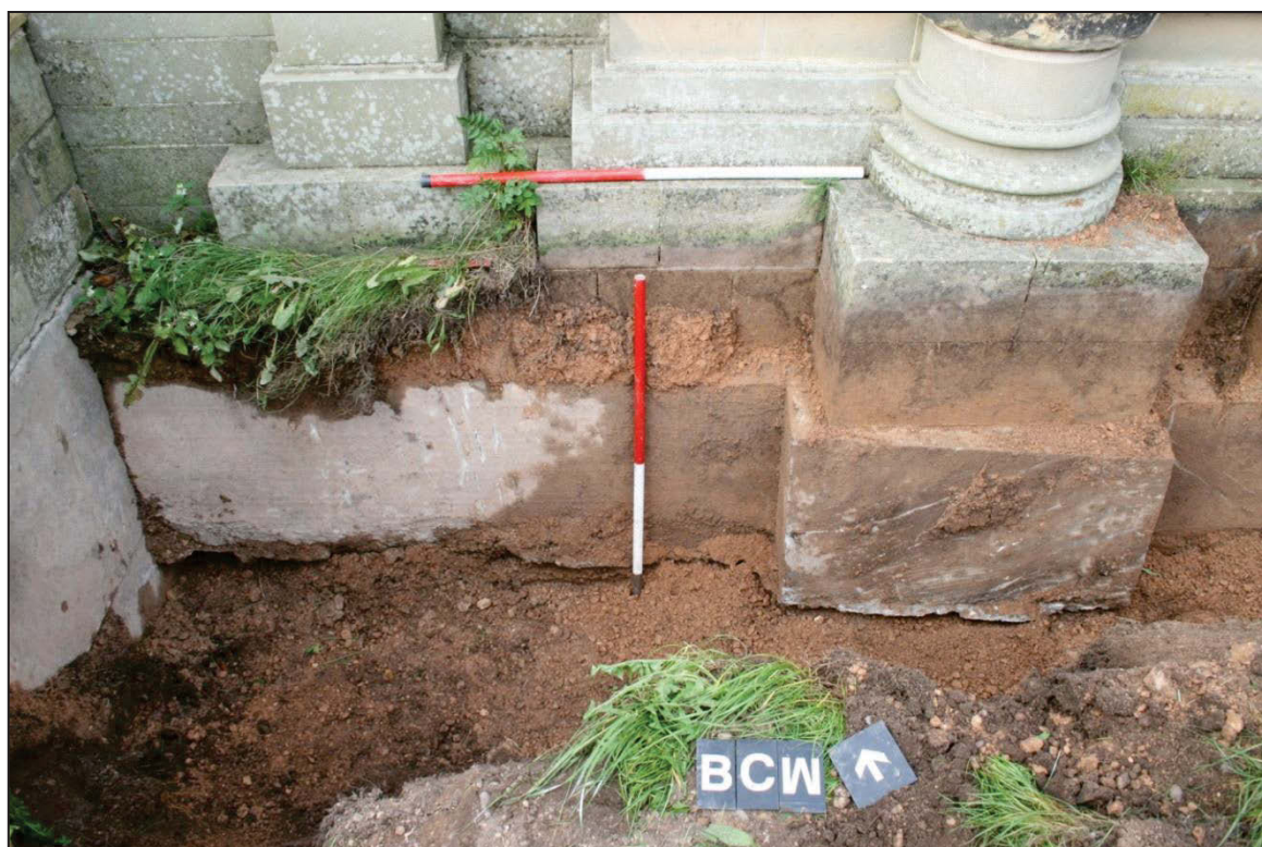
Plate 10: Section at concrete base of the southern side of the gate wall
