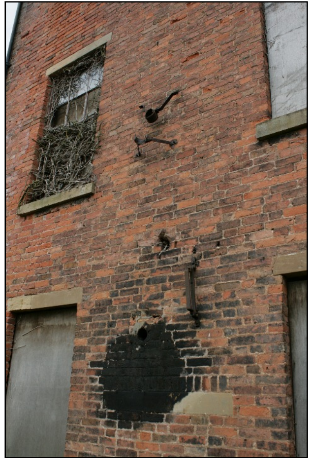
Plate 27: Exhaust brackets and sawn off pipe on the west gable for the engine housed on the ground floor, viewed looking north-east.
