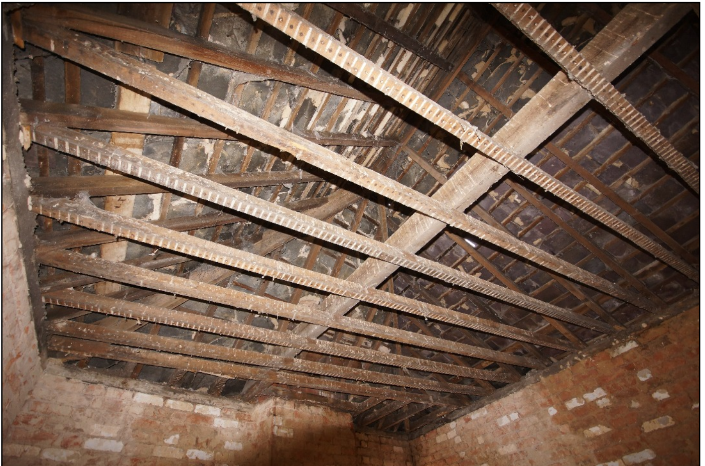
Plate 55: The roof of the house viewed looking south-east from the first floor of the east unit.
