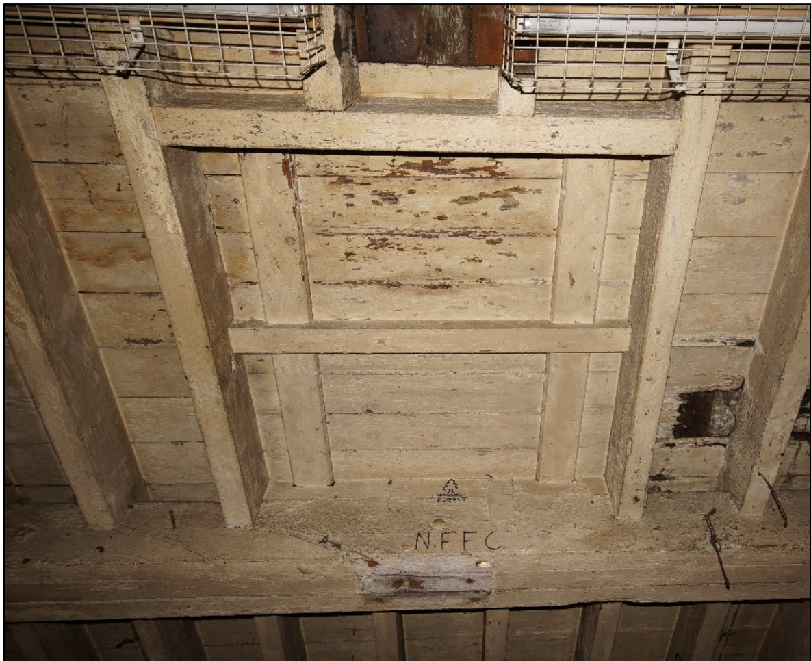
Plate 30: Hatch, or original access, between the ground and first floors, viewed looking east.
