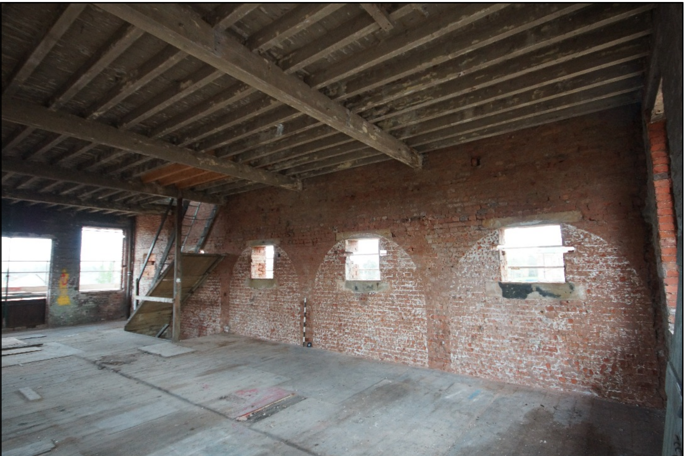
Plate 32: The south wall of the first floor of the west wing with the former cells outlined in the brickwork, viewed looking south-east. Note how the staircase truncates the cell.
