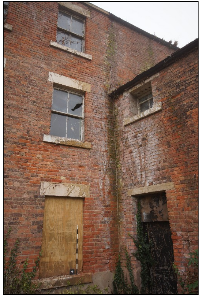
Plate 43: West elevation of the west wing abutted by the west unit of the house which is earlier than the east unit of the house which is tied into it, viewed looking north-east.
