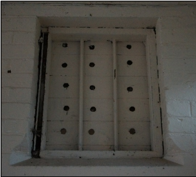
Plate 45: Original prison window in the wall dividing the ground floor, viewed looking south.
