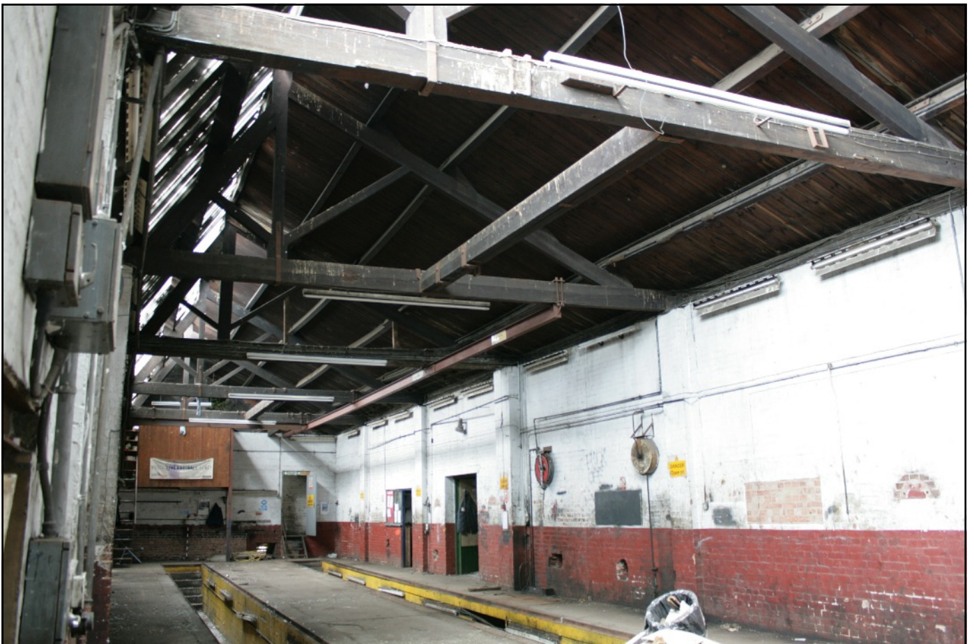
Plate 9: The interior of the former lace factory, converted into a garage during the mid to late 20th century, viewed from Bay 1 Unit 7 looking east.
