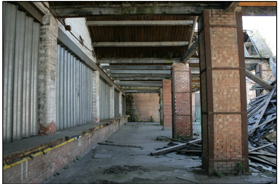
Plate 5: Openings in the wall dividing Bays 3-4 of Units 1-5, viewed looking south from Bay 3 Unit 1. Note the brick pillars that were rebuilt following the fire in the 1970s.
