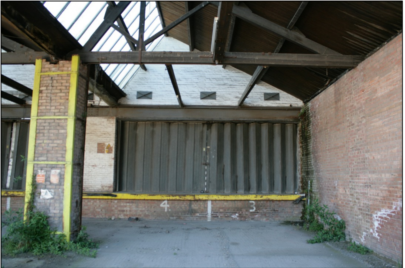
Plate 6: Bay 2 Unit 5, viewed looking east. The doorway was inserted and the floor raised when the former lace factory became a depot. The wall to the right, which is part of the garage, is also a modern build. The brick pillar was rebuilt following the fire in the 1970s. The metal ties above the doorway are probable insertions designed to provide additional structural integrity to the building.
