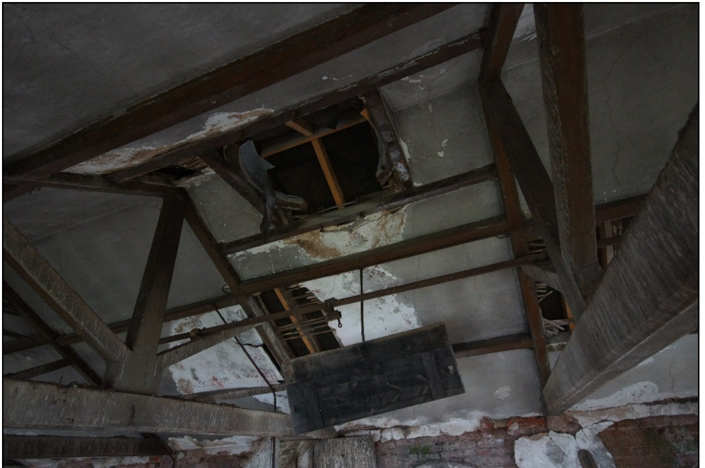
Plate 38: Ventilator and iron bar for the no longer extant winch in Bay 3, viewed looking south-east.
