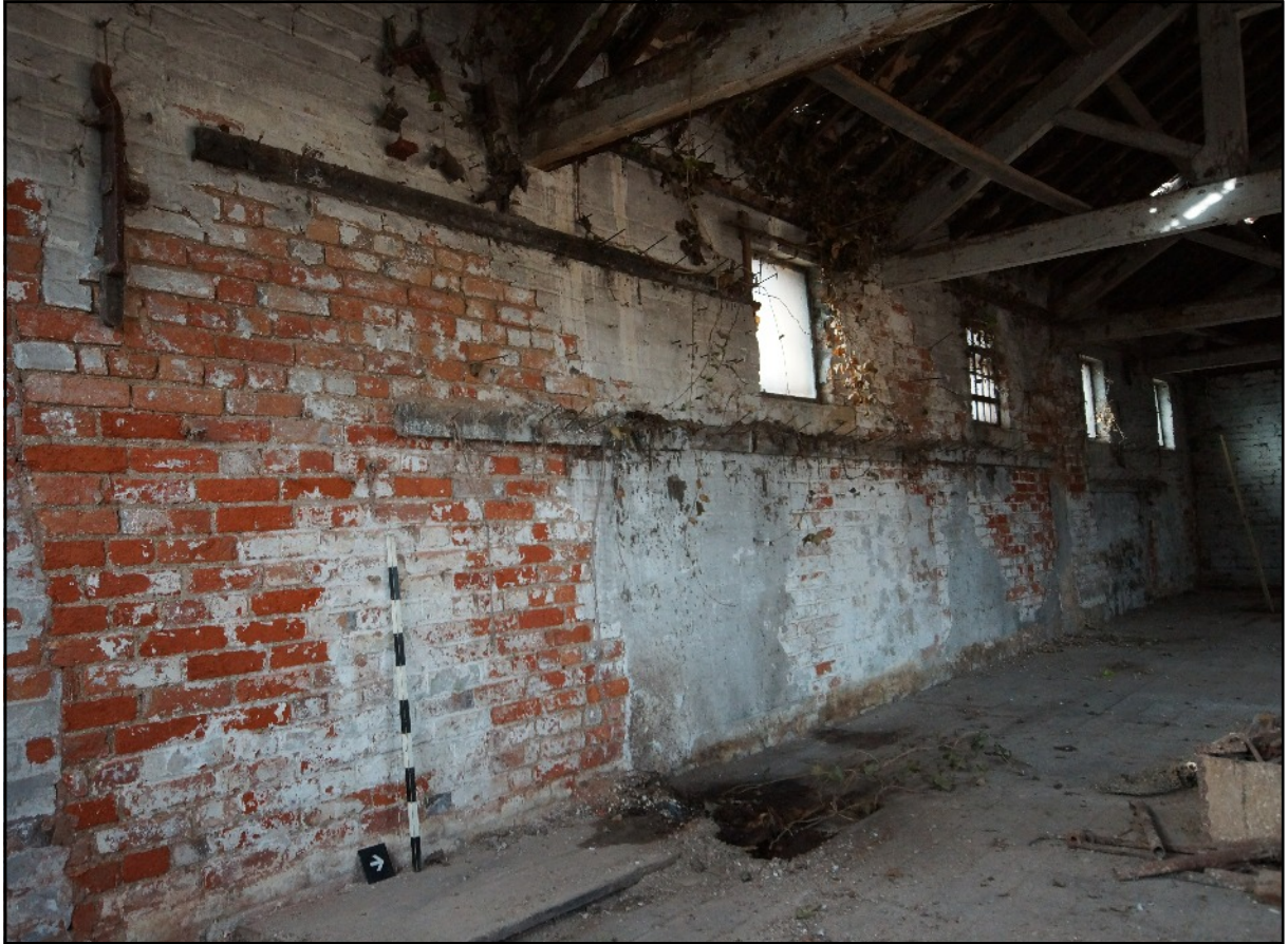
Plate 48: The bobbin racks extending down the west wall of the first floor of the west wing, viewed looking north-west.
