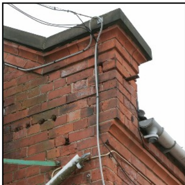
Plate 13: Stone kneeler and coping of the east gable and cornice of the north elevation, viewed looking south-west.
