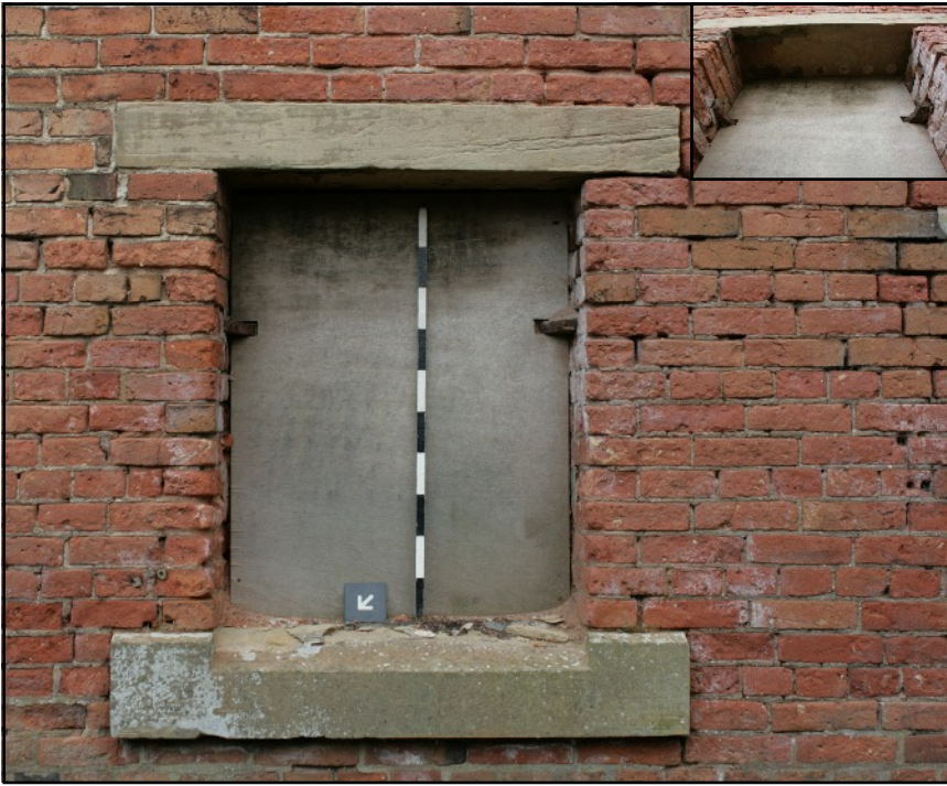
Plate 20: Detail of the original window type used on the ground and first floors of the north and south elevations. The insert depicts the holes for the diamond shaped iron mullion bars.
