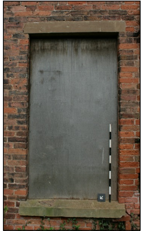
Plate 22: Southernmost ground floor window of the west gable, viewed looking east. Note that the same type of window is used on the floor above and in the east gable.
