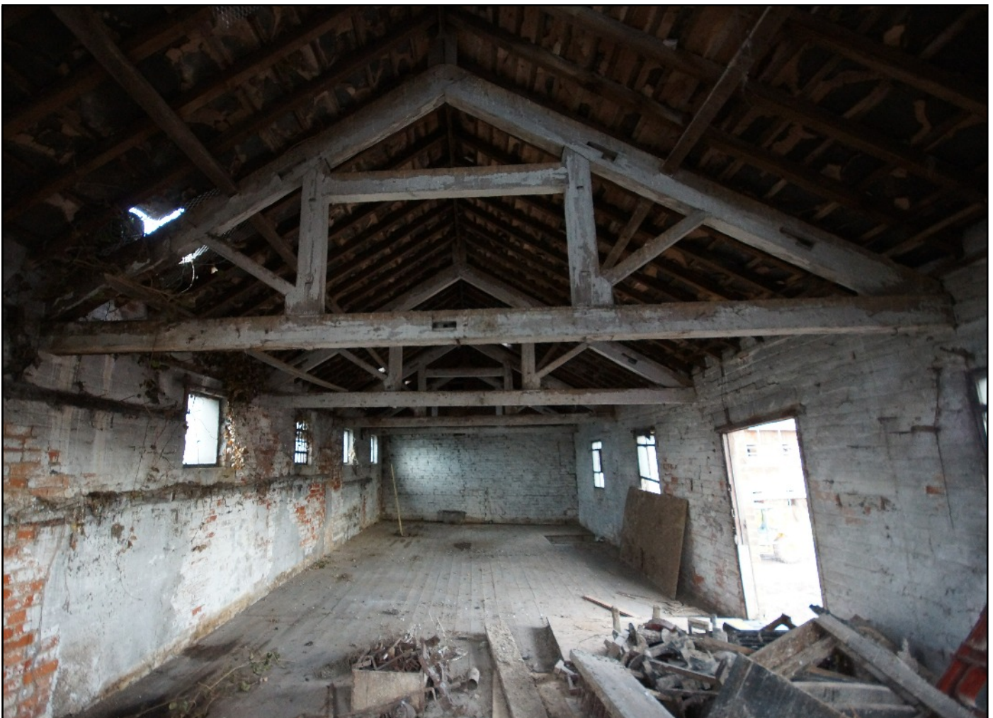
Plate 47: General view of the first floor of the west wing viewed from Bay 5 looking north.
