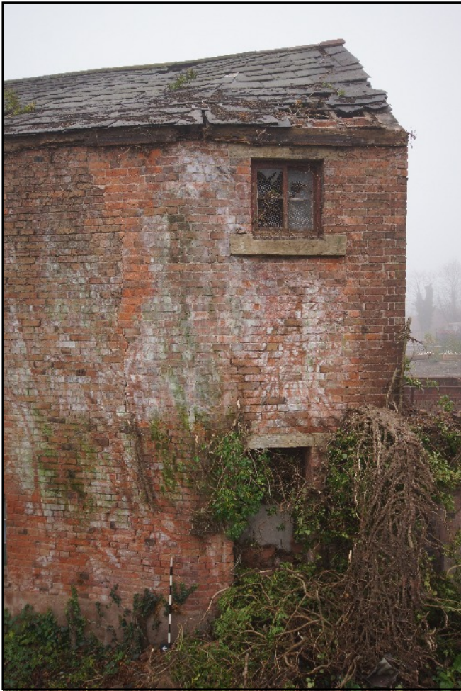
Plate 42: Building join on the west elevation of the west wing between the earlier phase to the north and the later phase to the south, viewed looking west.
