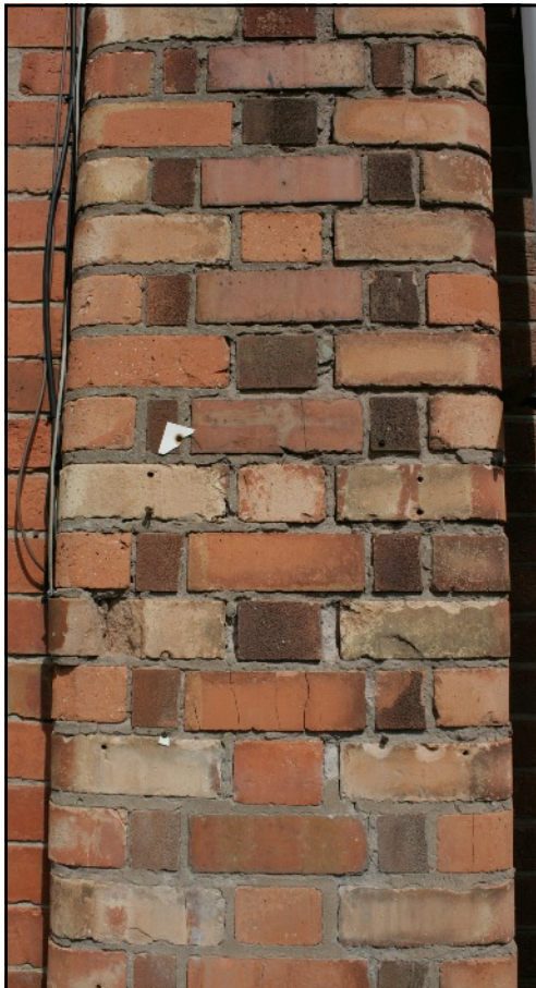
Plate 4: Decorative brickwork on the west face of the south wall of the former lace factory, viewed looking east.
