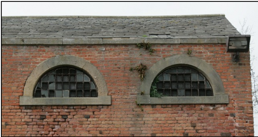
Plate 21: The semi-circular windows of the second floor of the south elevation containing the original iron glazing bars, viewed looking north.
