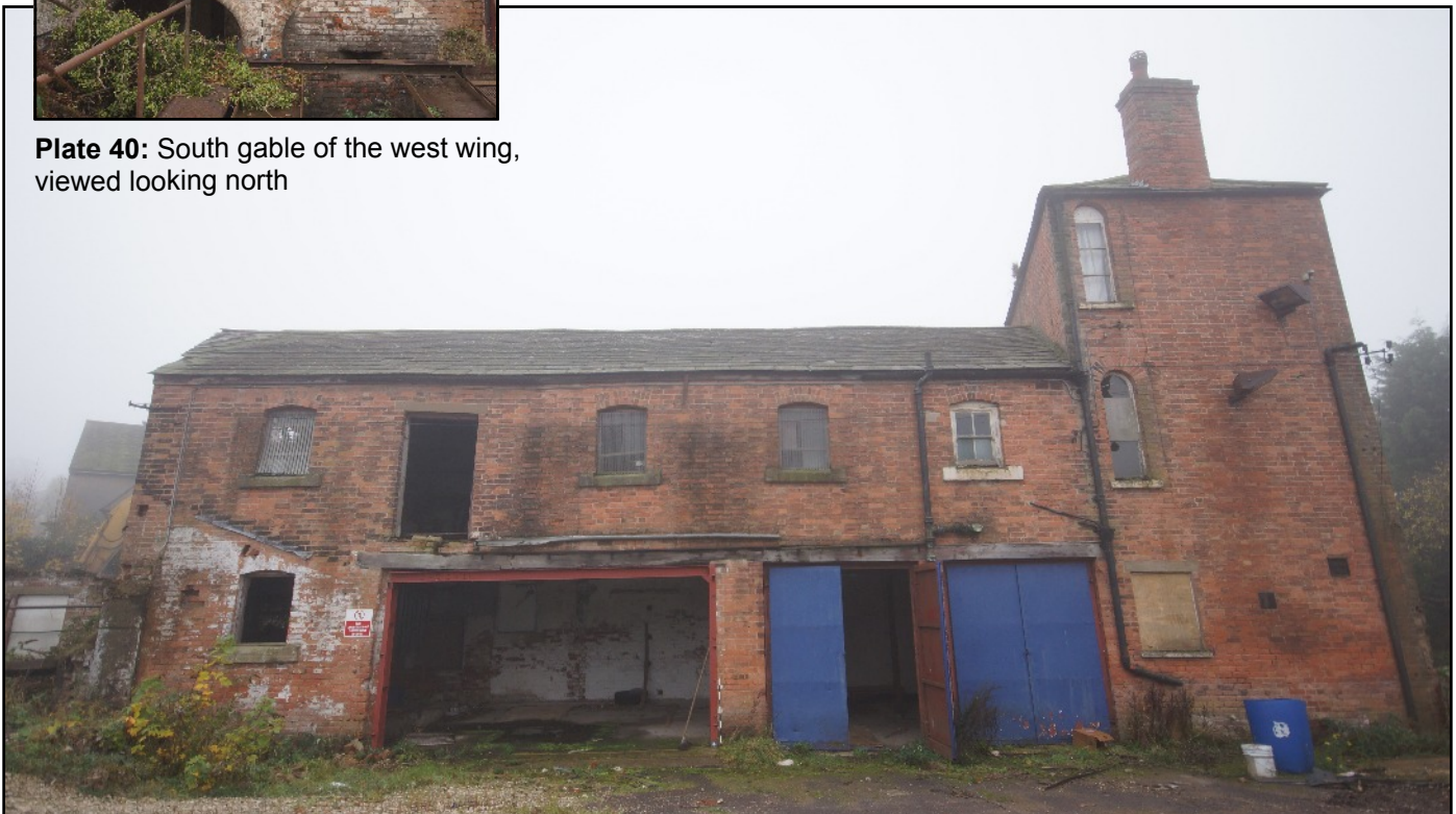
Plate 41: East elevation of the west wing and the east gable of the house, viewed looking west. Note that there is no building join between the two buildings indicating that they are contemporary.
