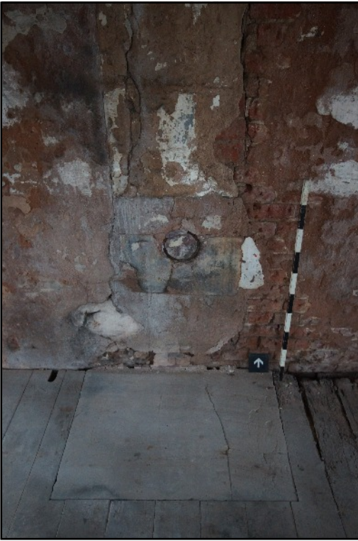
Plate 33: Hard standing for a former stove and inserted chimney in the north wall of the first floor of the west wing, viewed looking north.
