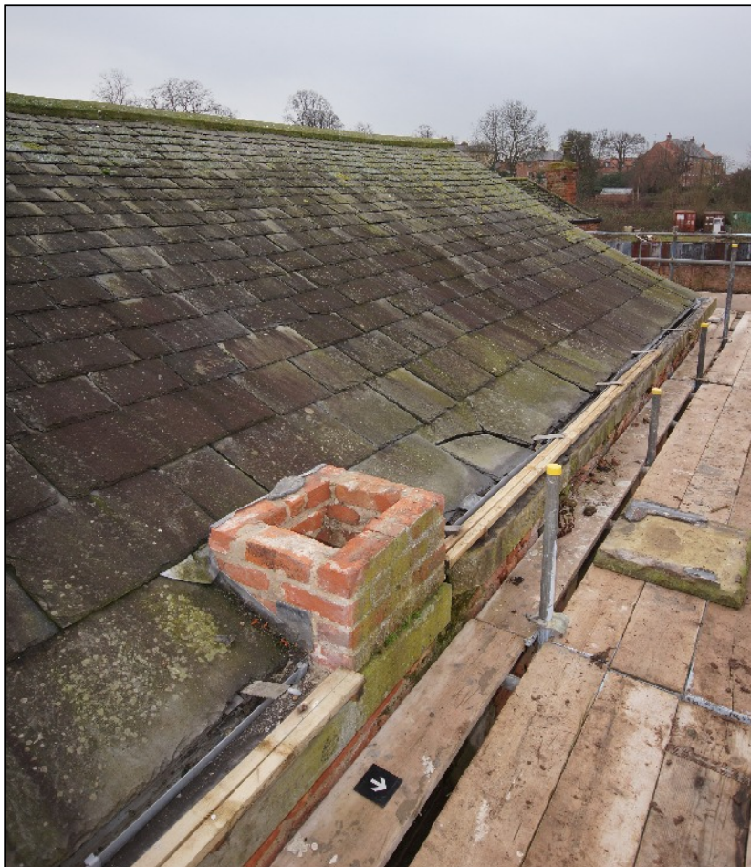
Plate 28: North face of the roof and the inserted chimney, viewed looking south-west.
