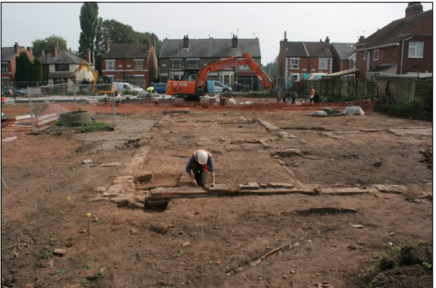
Plate 2: Trench 11 during excavation with the north end of the main range in the foreground, viewed looking east.
