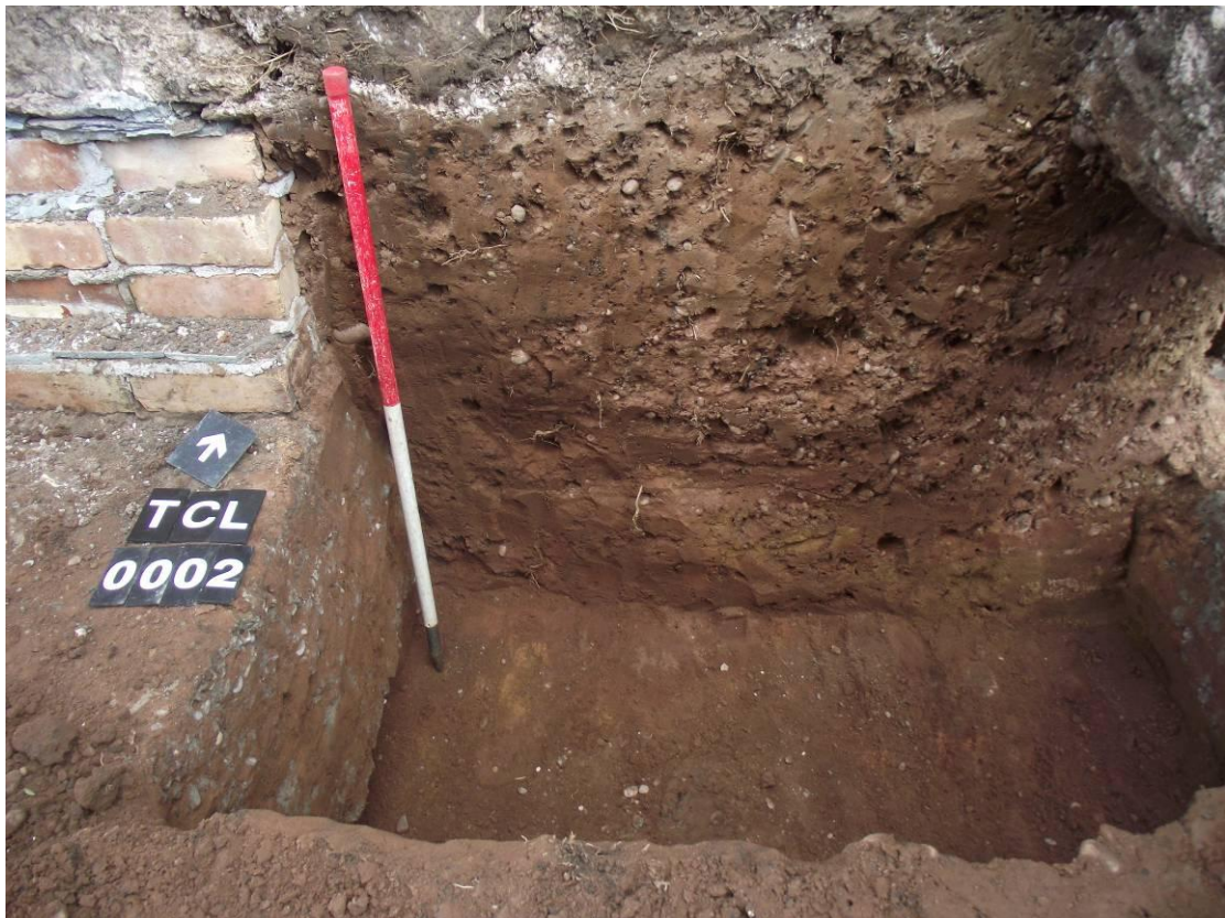
Plate 4: Second stage of excavations for underpinning (note the area of concrete to the left from the first stage). Scale = 1m
