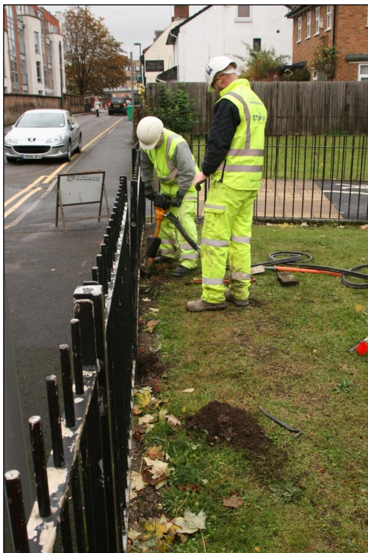
Plate 1: Pneumatic hammer used in the cutting of concrete, looking north along Old Church Street.
