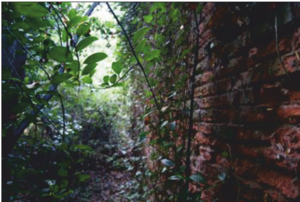
Plate 9: Wall face 4 showing soiled brickwork, looking north-west.
