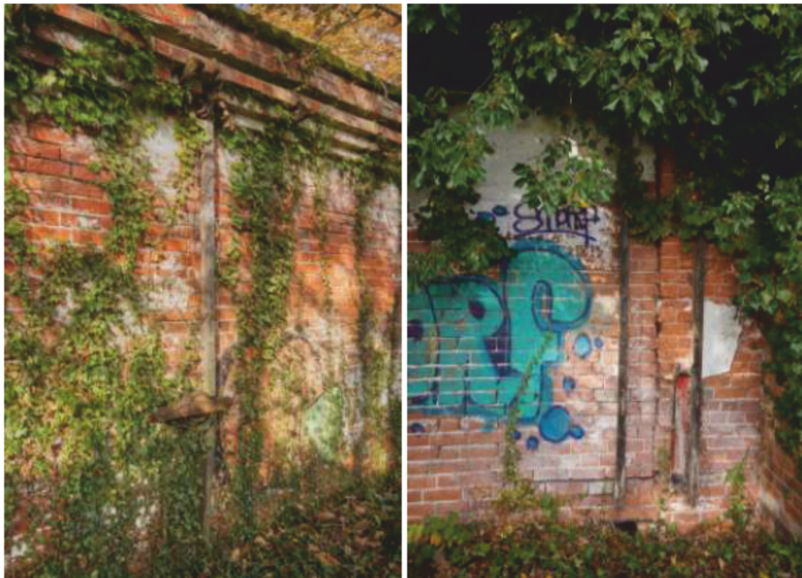
Plate 50, left, and Plate 51, right: Wall face 19, showing wooden battens and mechanisms for louvers, and straight joint. Looking north-east and east.
