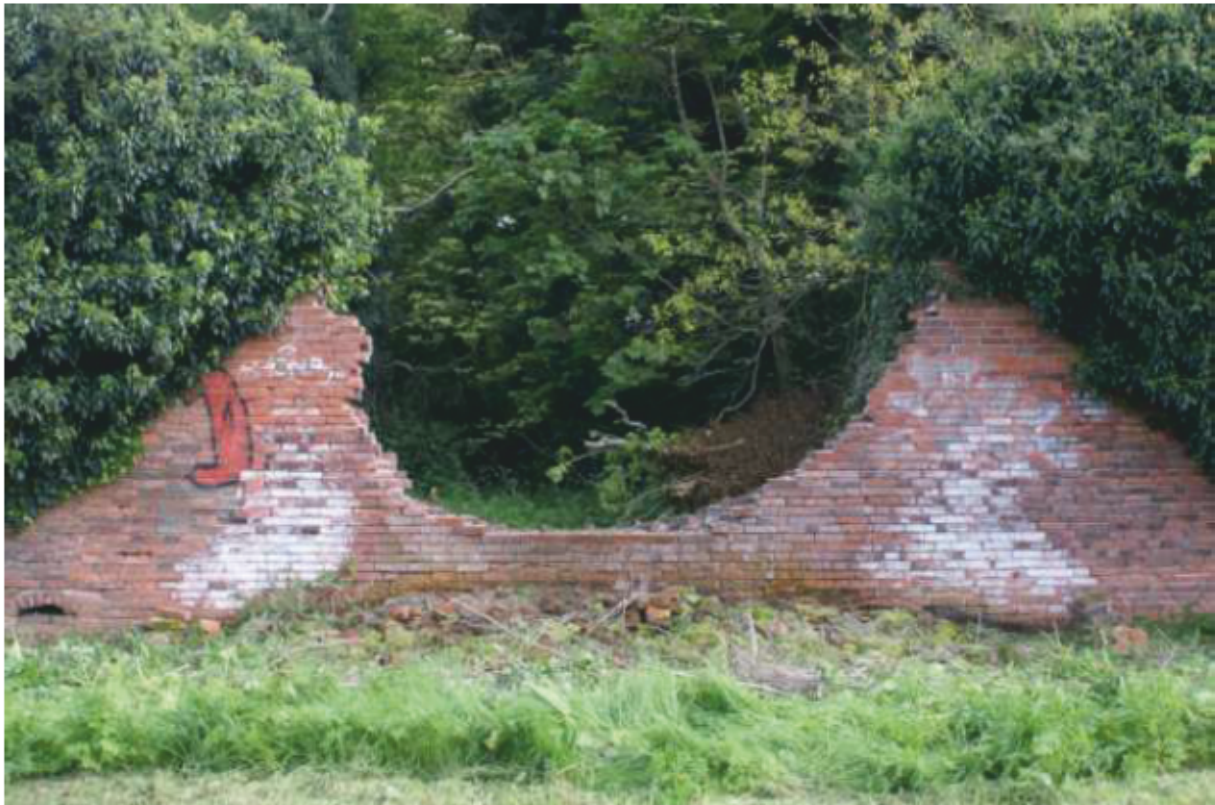
Plate 5: Wall face 3, showing damage caused by fallen tree. Looking north
