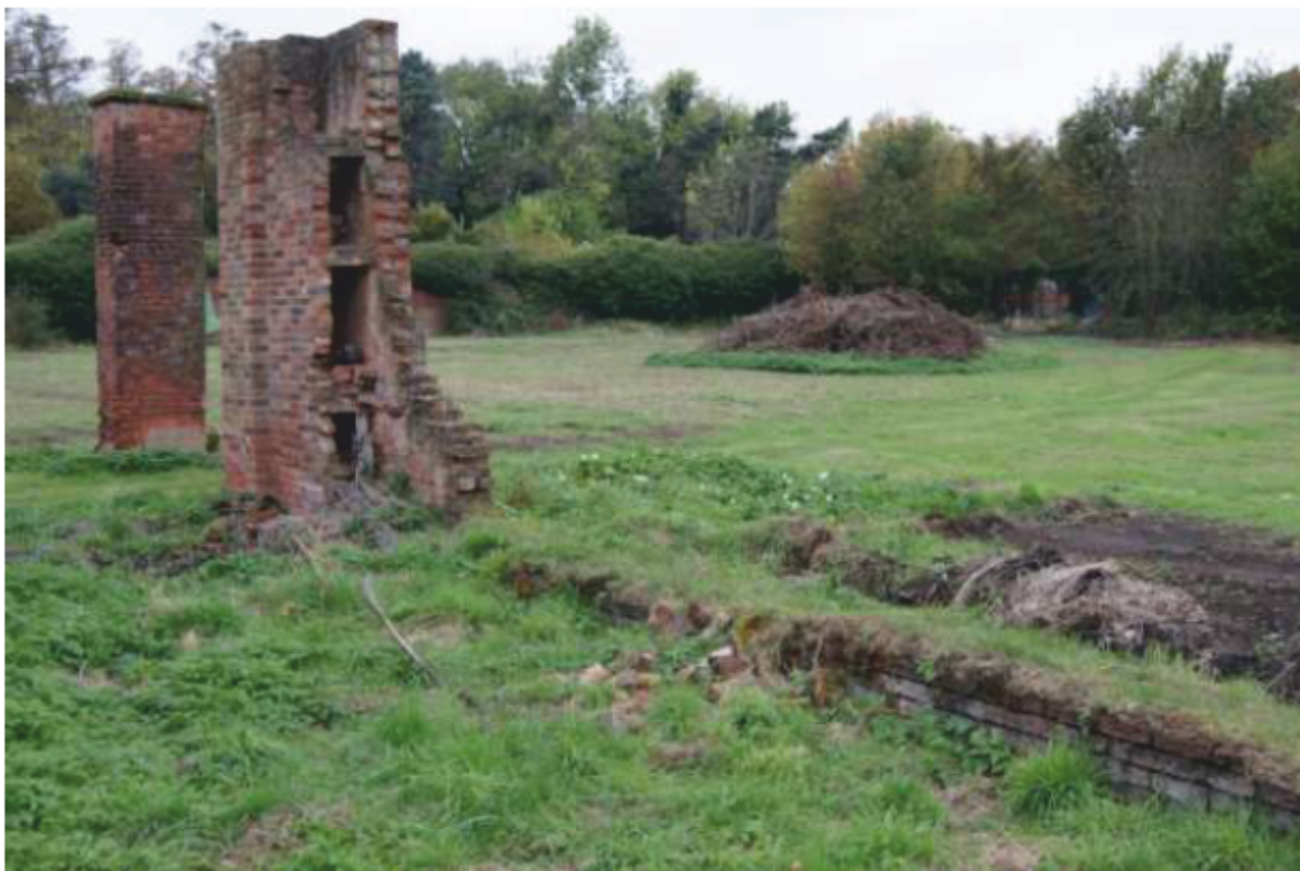
Plate 29: Wall face 15: pillar at western end of wall, showing damage and flues. Looking west-north-west.
