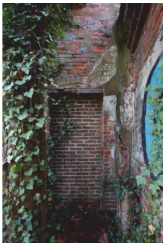
Plate 24: Wall face 13, blocked pedestrian entrance at northern end of wall face. Looking west.
