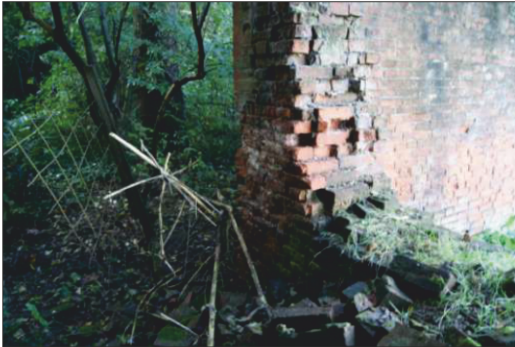
Plate 7: Wall face 4 showing damage to the wall face, looking west.
