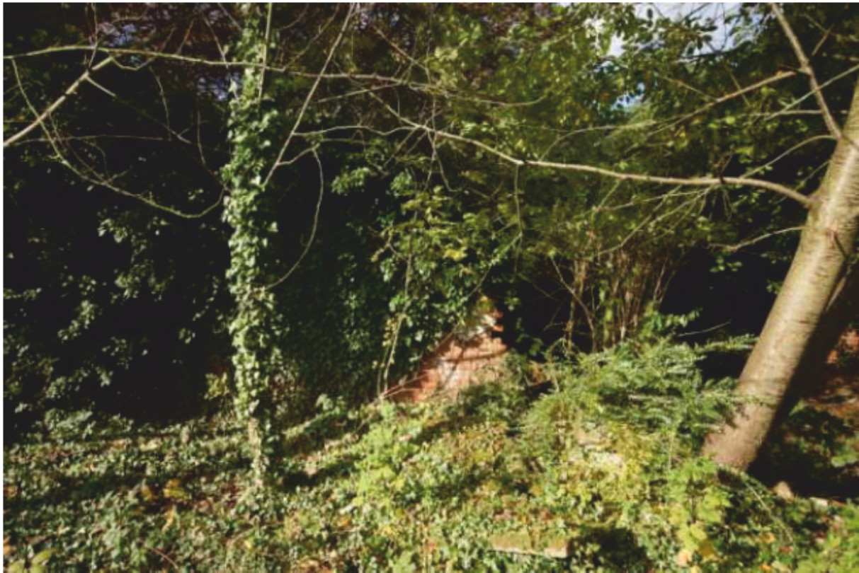
Plate 52: Wall face 19. Eastern end of wall, showing collapsed pillar. Looking north.
