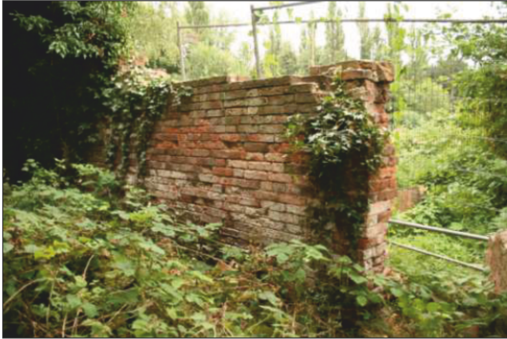
Plate 19: Wall face 8 showing damaged entrance, looking south-west.
