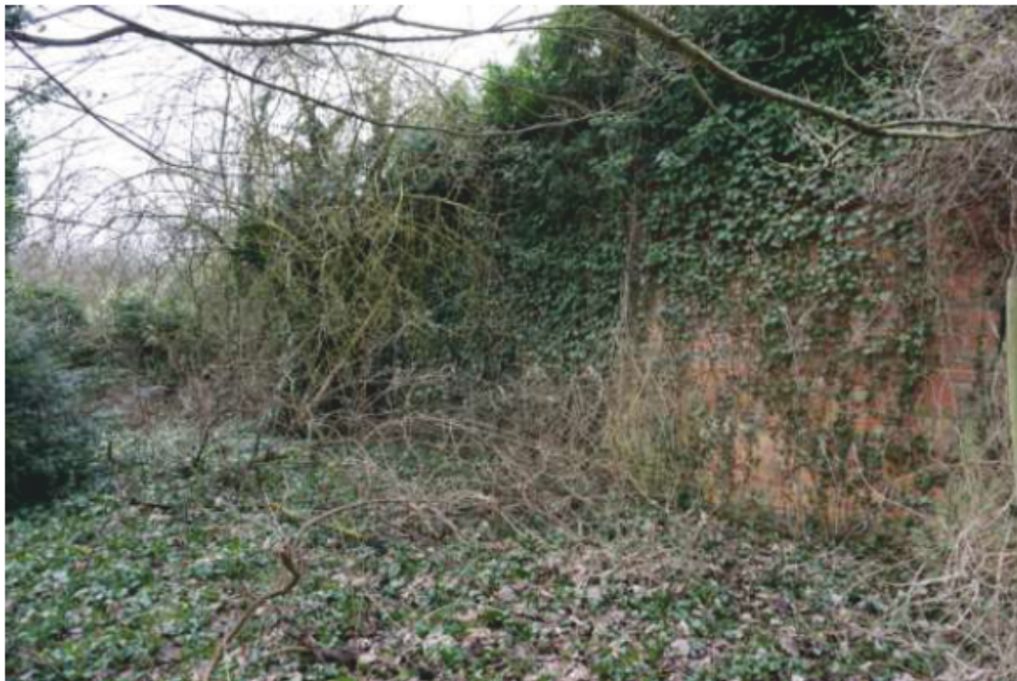
Plate 42: Wall face 17 showing overgrown vegetation and heavy ivy coverage, looking north-west.
