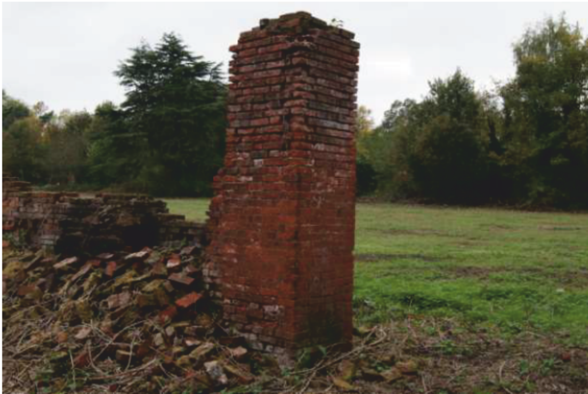
Plate 27: Wall face 15, damaged standing pillar at east end of wall. Looking north-west.
