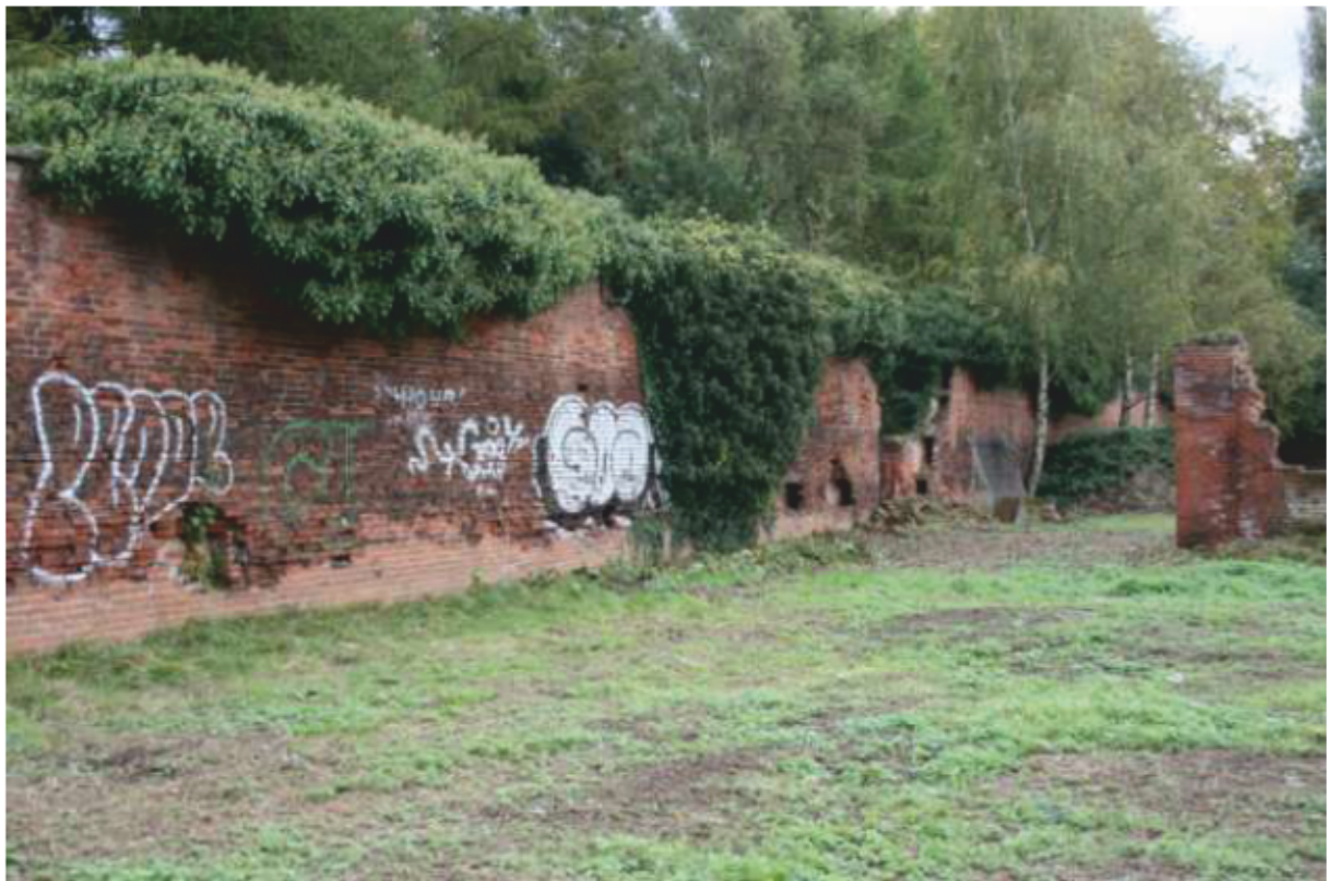
Plate 20: Wall face 9, showing missing brickwork and heavy graffiti. Looking south-east.
