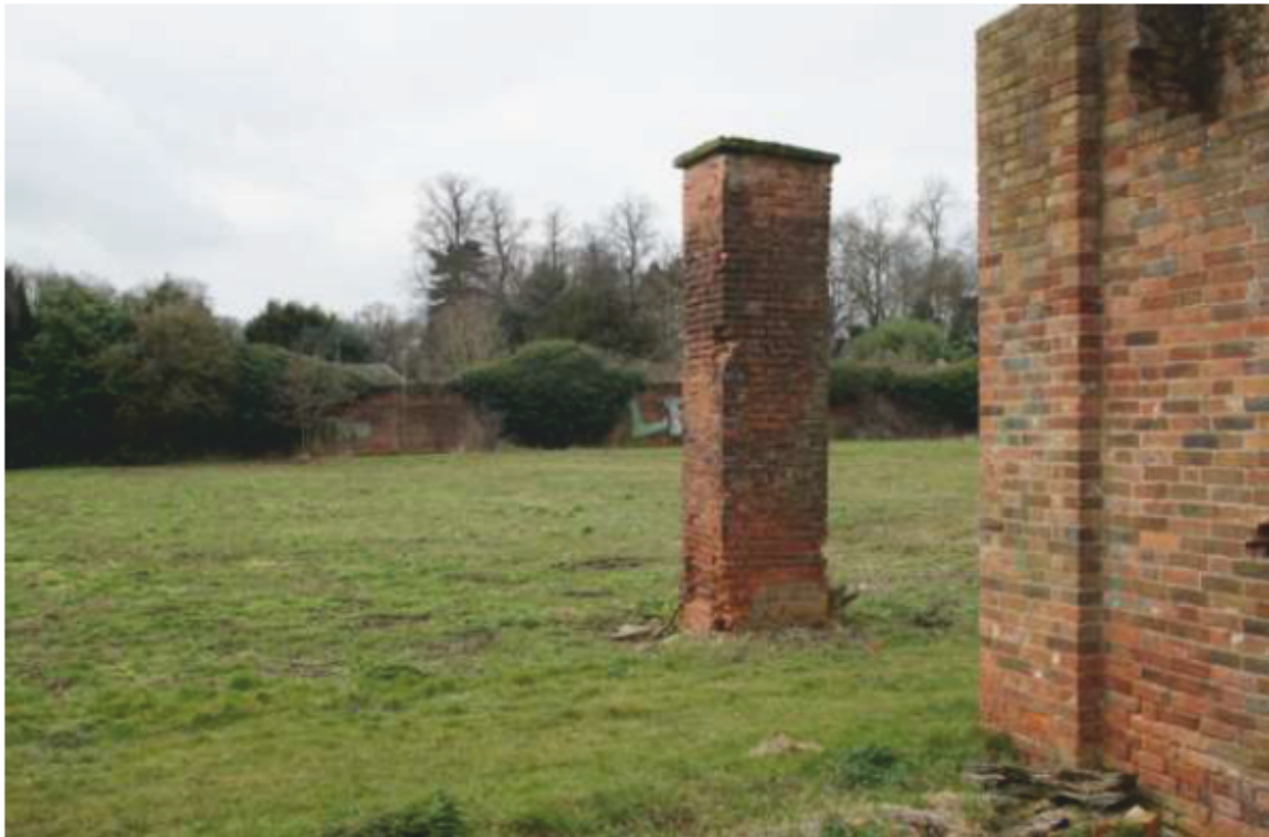
Plate 31: Wall face 21, now entirely missing. Looking west.
