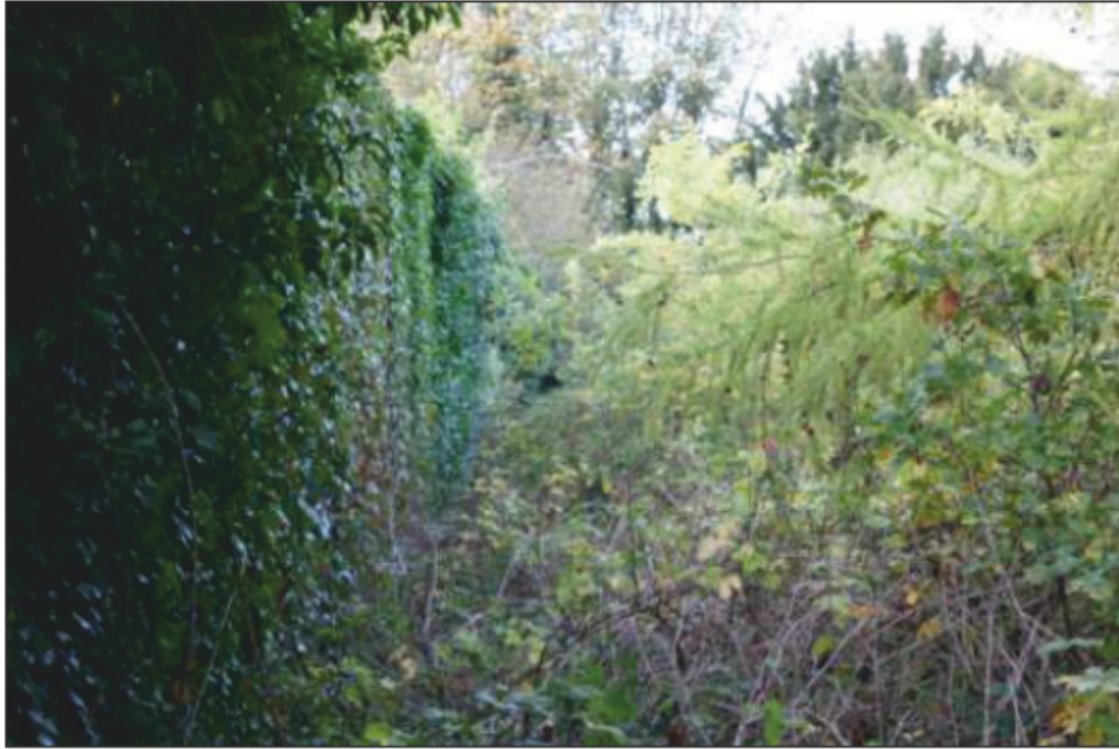
Plate 21: Wall face 10 showing overgrown vegetation, looking north west.
