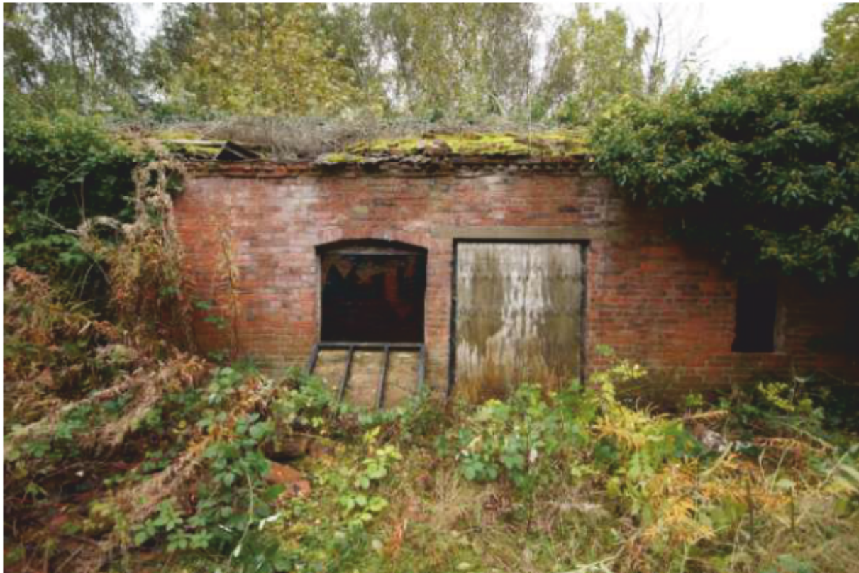
Plate 46: Wall face 18, Shed Phase 1, showing roof collapse, graffiti, boarded doors and architectural detailing. Looking south.
