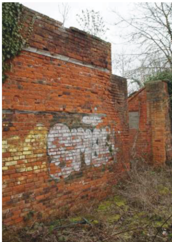
Plate 43: Wall faces 17 and 11 showing north-eastern entrance, graffiti, and inset wooden beams. Looking north-east.
