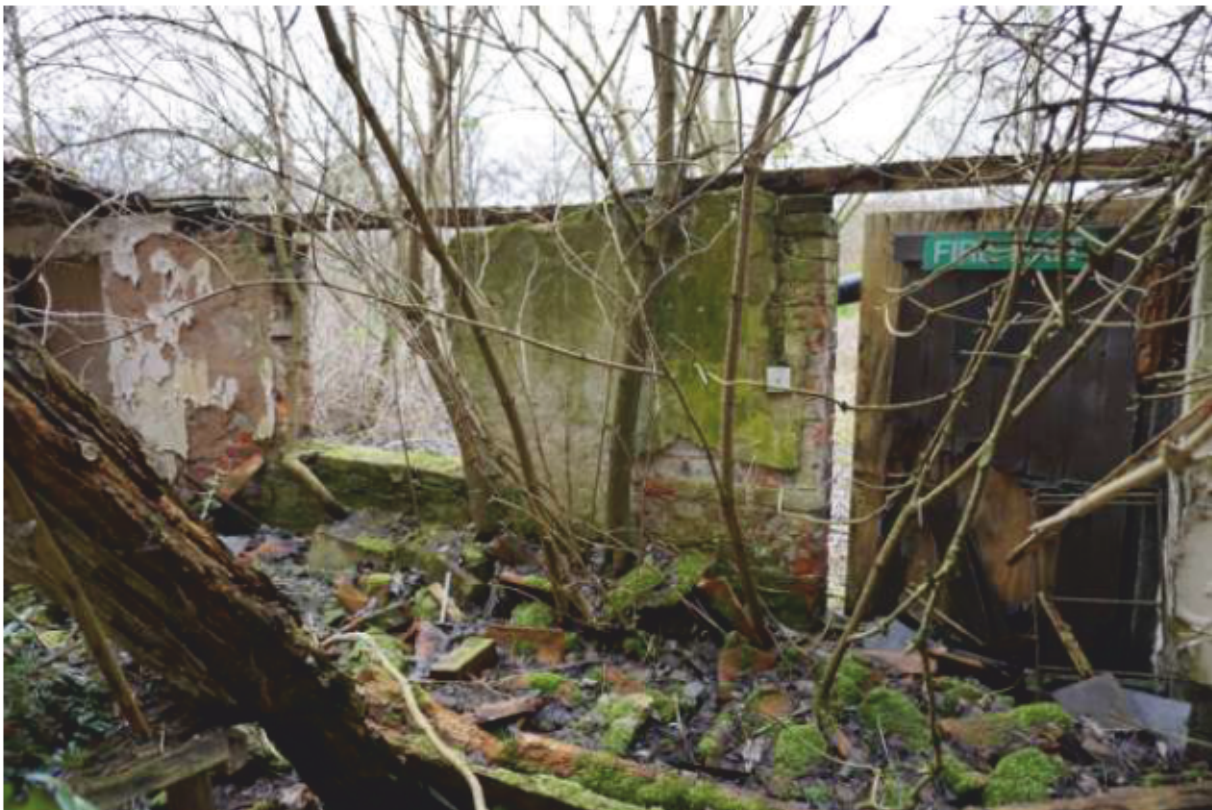
Plate 41: Shed Phase 2 interior, showing evidence of recent occupation, self-set trees, and massive timber damage. Looking north.
