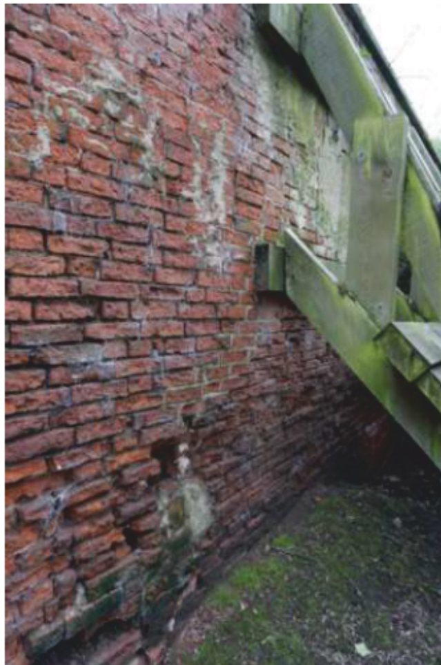
Plate 36: Wall face 12, showing degraded (double-skinned) brickwork and wooden buttress supports. Looking south-west.
