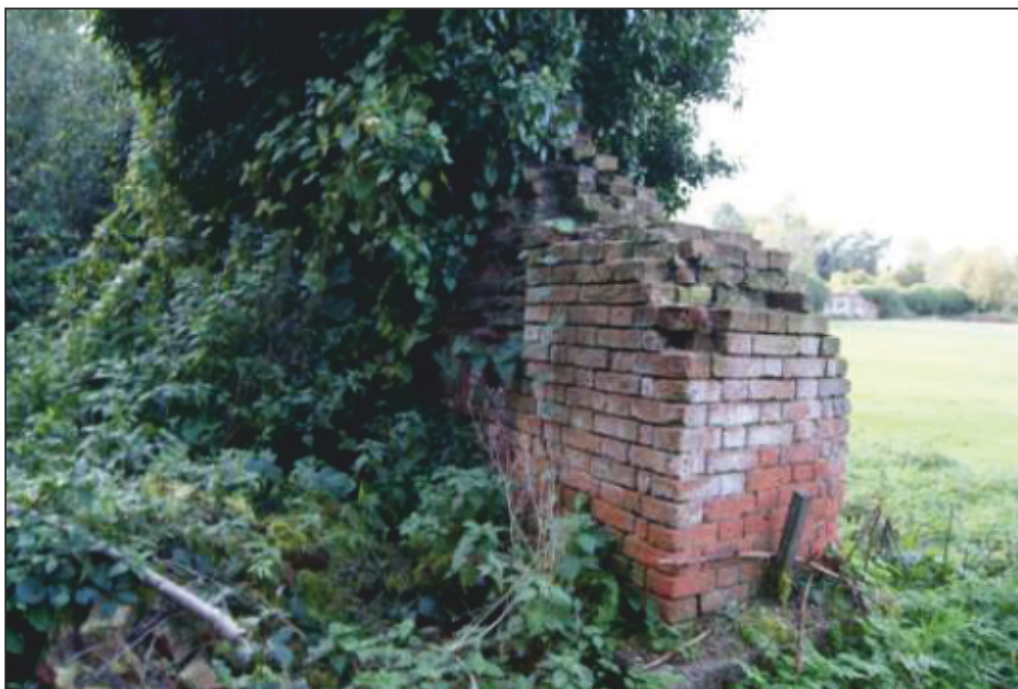
Plate 10: Wall face 4 showing damaged pillar, looking north-west.
