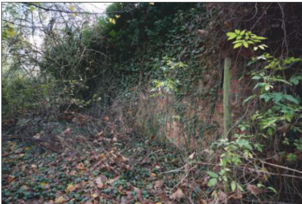
Plate 32: Wall face 11 showing overgrown vegetation, looking north west
