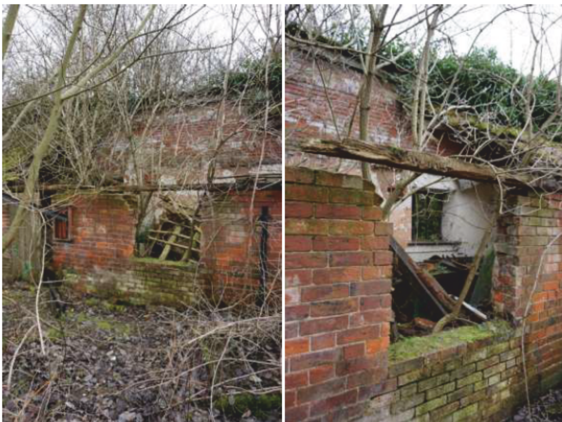
Plate 38, left, and Plate 39, right: views of Shed Phase 2, showing collapsed roof, self-set trees and the window shown in Plate 34. Looking south-east and south-west.
