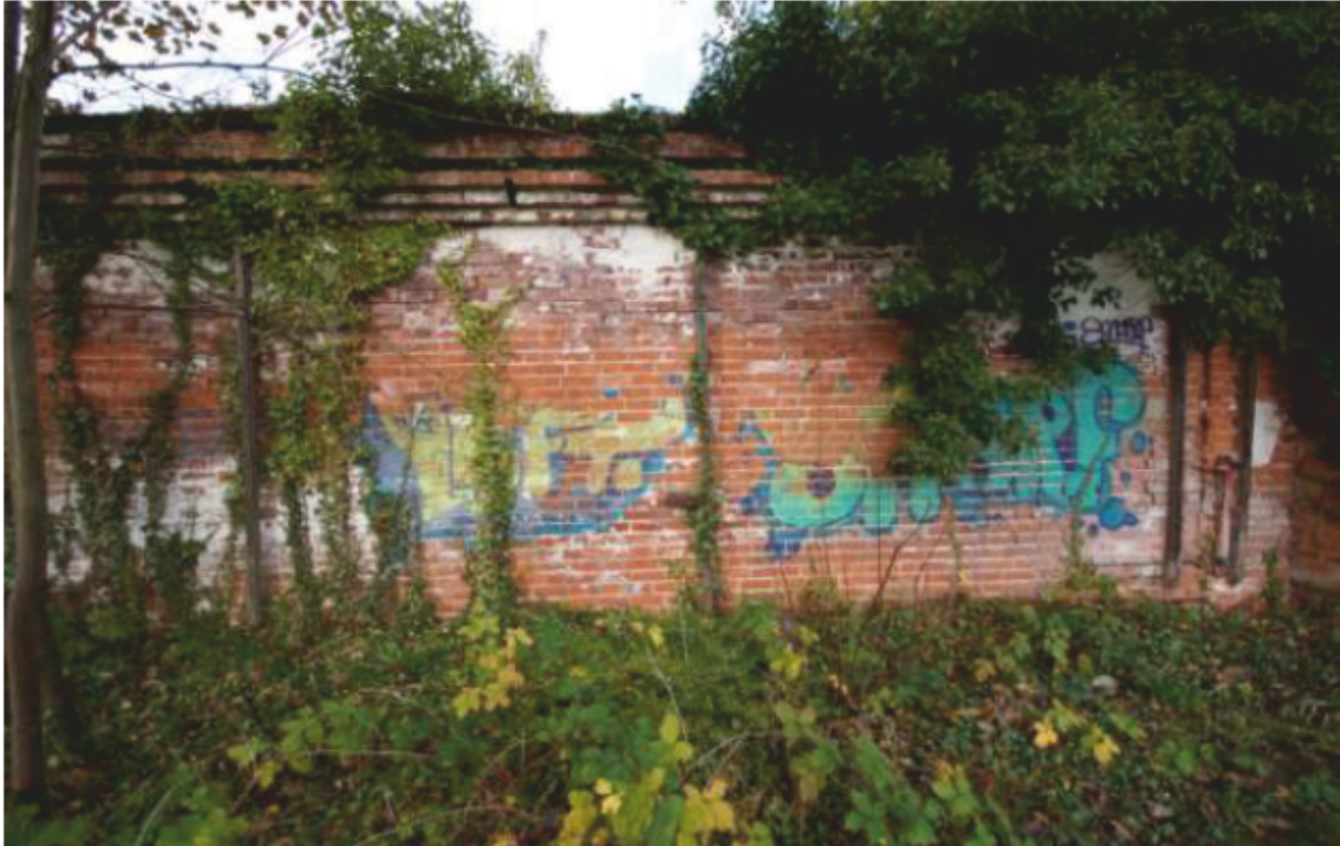
Plate 49: Wall face 19, showing graffiti and general condition. Looking north.
