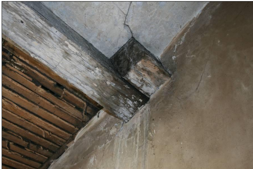
Plate 18: Detail of roof purlins and exposed lath for plaster in room 22, viewed looking south-west
