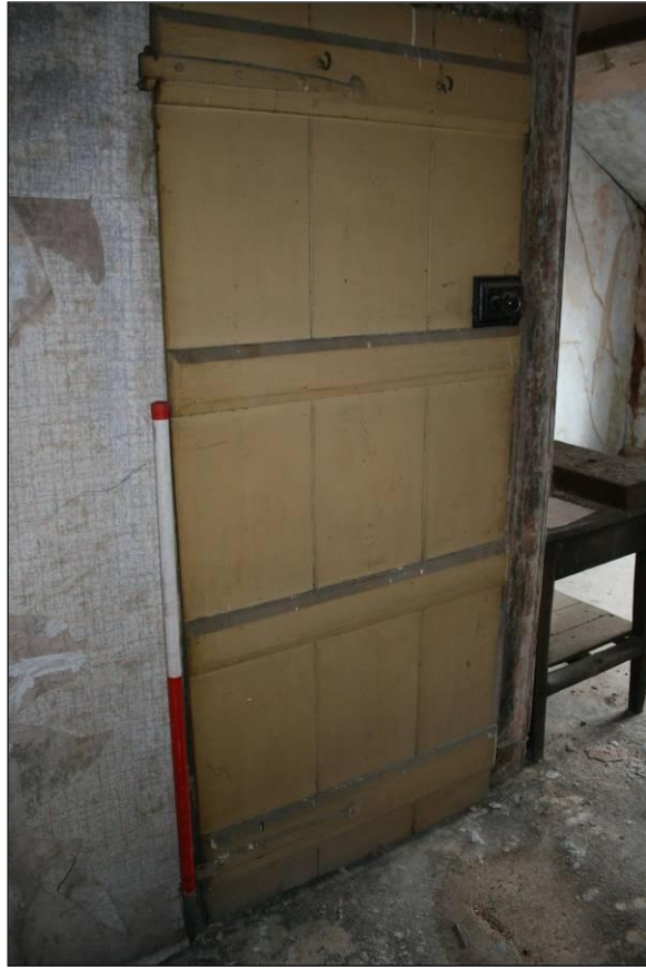
Plate 17: Detail of original plank and batten door in room 24, viewed looking south-east
