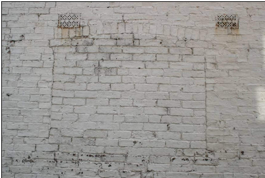
Plate 5: Detail of blocked up brick arch window in phase A, viewed looking east
