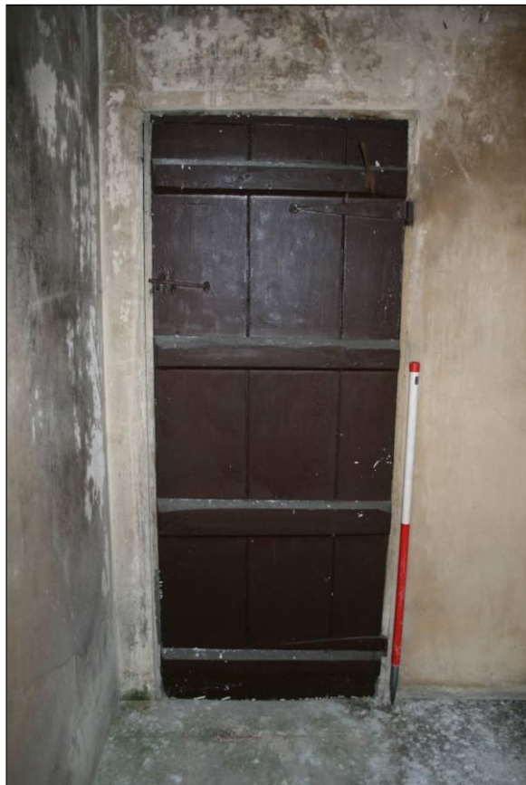
Plate 16: Detail of original plank and batten door in room 22, viewed looking north
