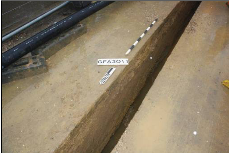
Plate 6: Representative section of vacuum sewer trench north of the West Glen River
