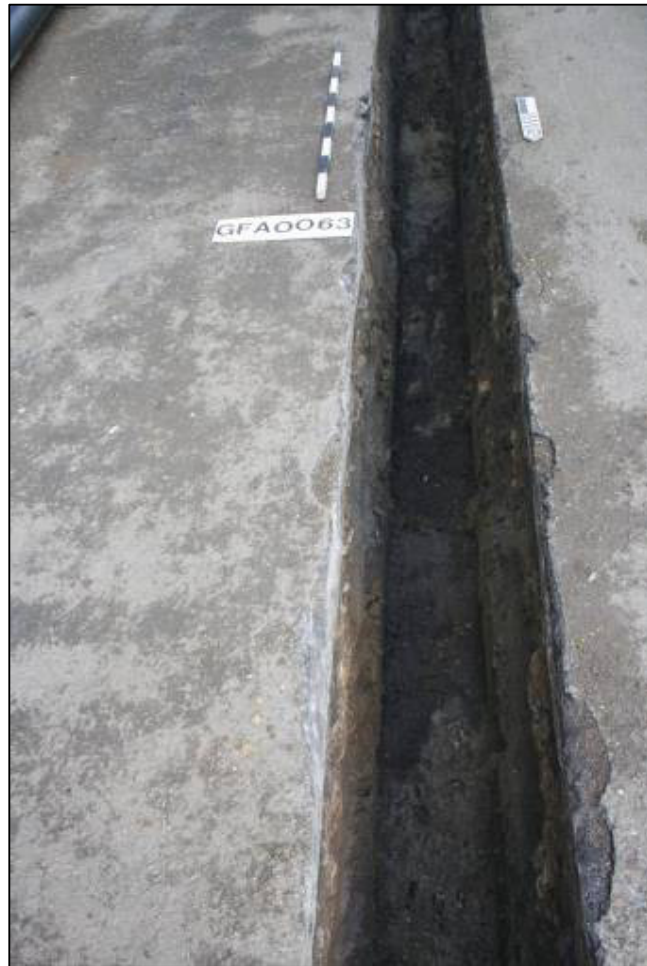
Plate 7: Vacuum Sewer Trench, north of West Glen River looking south, showing ditch [1064]
