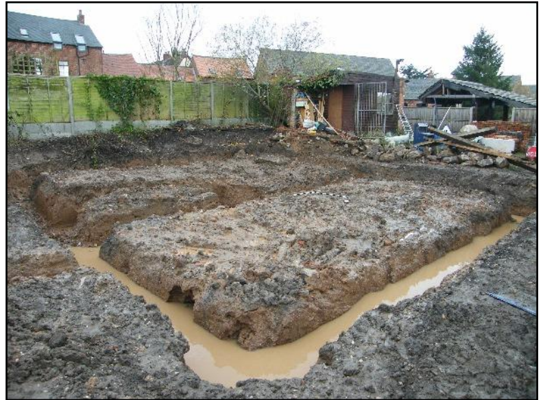
Plate 2: General view of the foundation trenches from the south-west corner of the development, viewed looking north-east.
