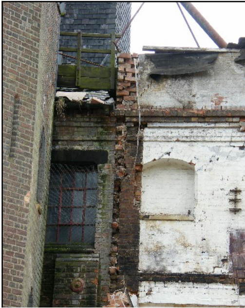
Plate 12: Position where stair-turret adjoined the Main Range's north-west wall and where the 1884 maltings extension was added.
