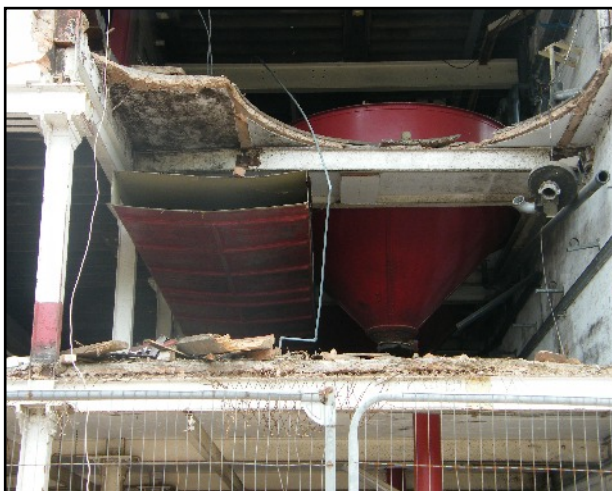
Plate 16: Metal funnel located in the south-west end of the Main Range, viewed looking south-east.
