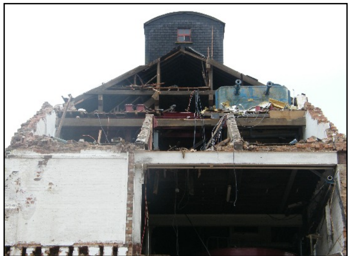
Plate 15: Roof structure of the Main Range at the south-west end, viewed looking south.
