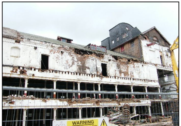
Plate 17: North-west wall of the Main Range, south western end, viewed looking south.
