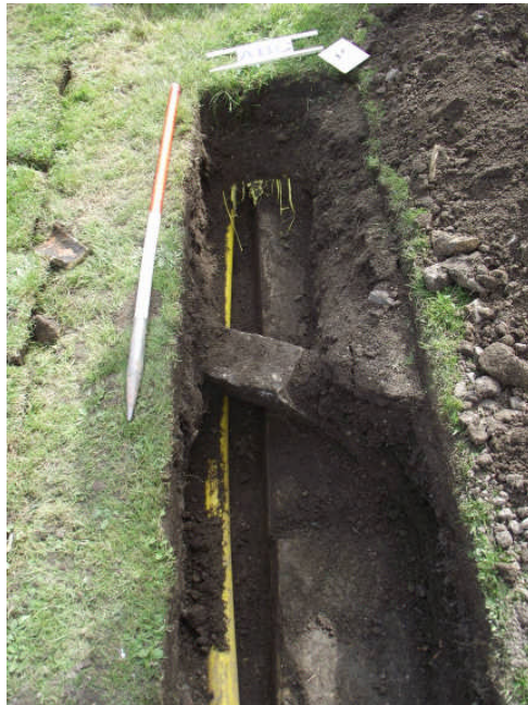
Plate 9: Area 05 showing 0025 stone slabs, with existing pipe in the trench to the left. Disturbed kerbing 0032 is present with in centre. Looking south.
