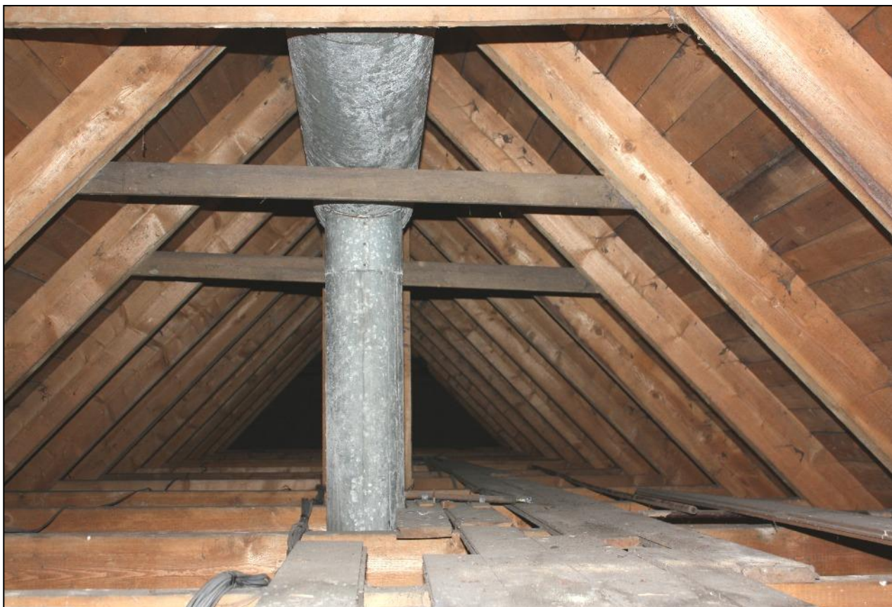
Plate 19: View looking towards the south-west end of the chapel's attic showing closely spaced trusses with simple collars and pipe-work for the ventilation system.
