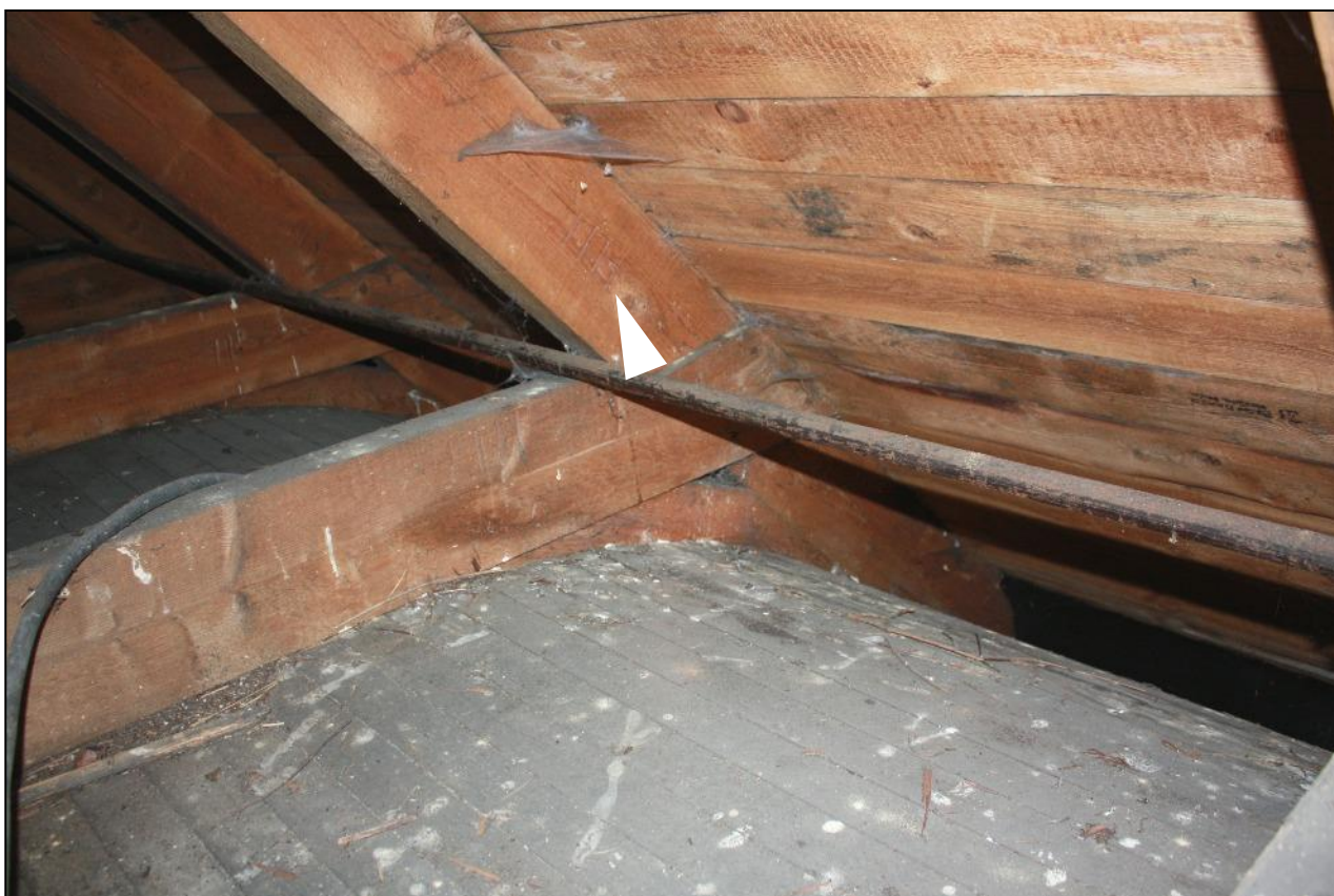
Plate 20: Junction of a tie-beam, principal rafter, connecting brace and curving ceiling timbers. The arrow points at an assembly mark.
