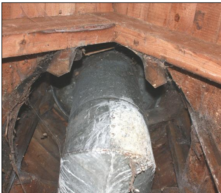
Plate 21: Where the ventilation pipe-work connects to the external spire.
