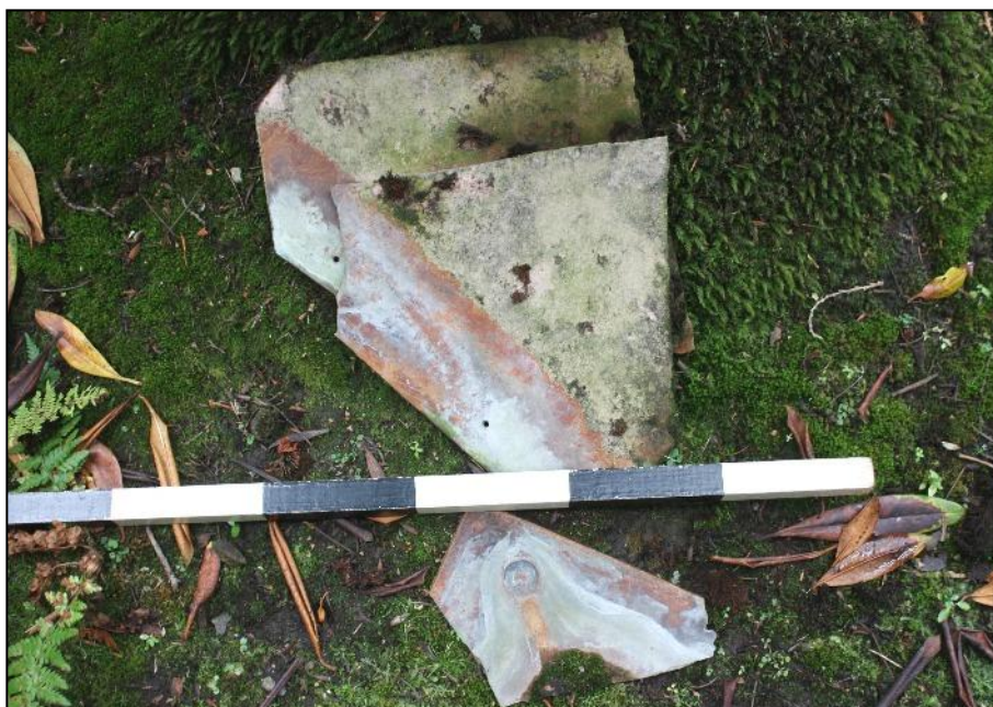
Plate 12: Fragments of asbestos tiles from the roof.
