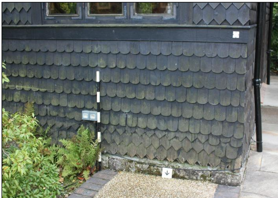
Plate 11: Stone and concrete base and closer-set shingles towards the bottom of the side walling.
