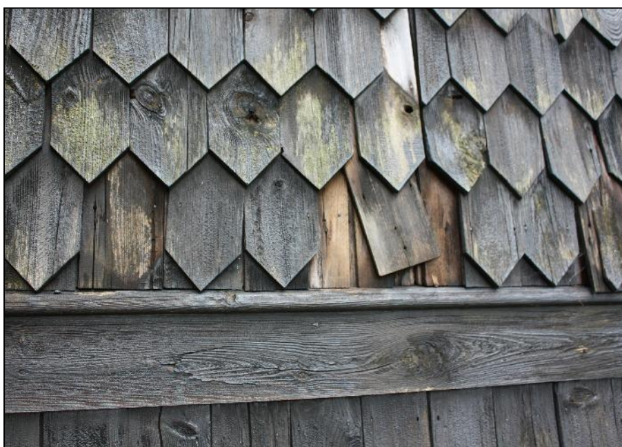
Plate 13: Area of lost and damaged shingles and exposure of timber layering.
