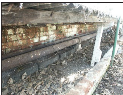
Plate 24: Heating pipes beneath the southern benches in the Hot-House, viewed looking south-west
