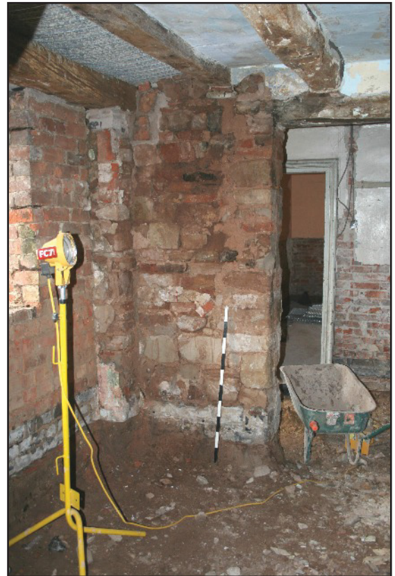
Plate 18: South-west corner of the ground floor of the Cottage, C, viewed looking south-west
