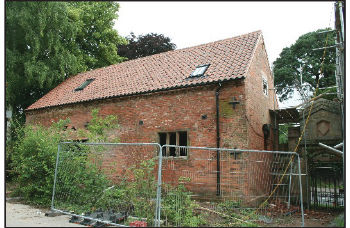
Plate 2: South elevation of the West Barn showing the stone mullion window, viewed looking north-west
