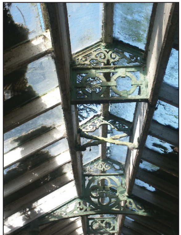
Plate 23: Decorative cast iron work in the apex of the Hot-house, viewed looking west
