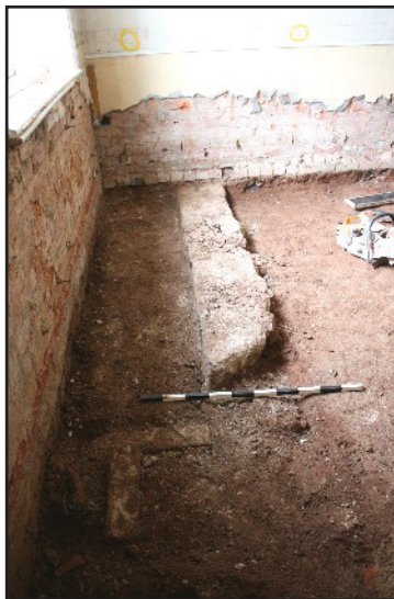
Plate 28: Walling pre-dating the addition of the House Keepers Room to Epperstone Manor House, viewed looking east
