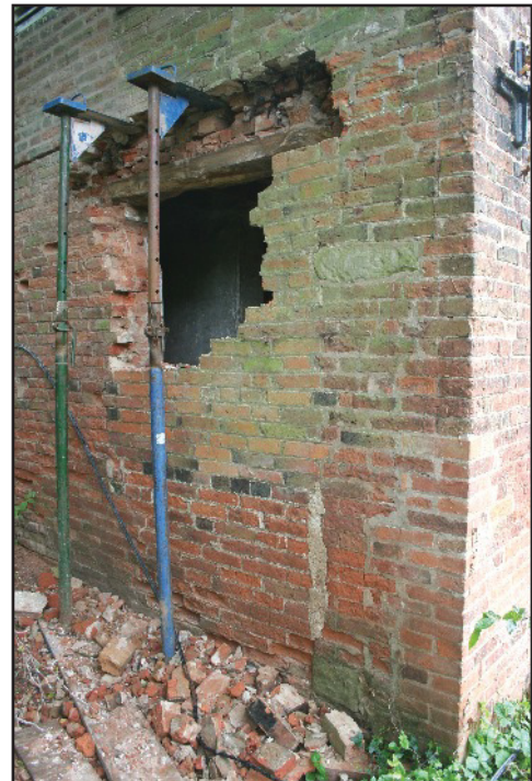
Plate 5: Former doorway in the west gable wall of the West Barn with wooden lintel and some stone quoins surviving, viewed looking south-east
