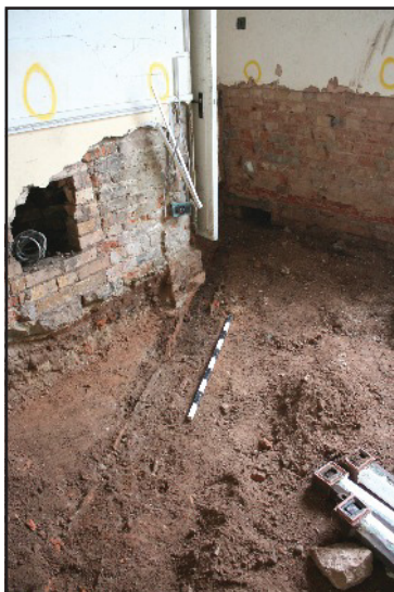
Plate 29: The drain beneath the walls and fireplace in the House Keepers Room, Epperstone Manor House, viewed looking east
