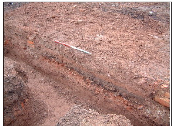
Plate 33: Two walls within the south-west facing section of Building Plots 27 and 28. Note the concrete foundation indicating they belong to the 1950's garage, viewed looking west
