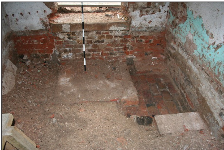
Plate 19: Exposed brickwork in the floor of the Cottage, E, and doorway, viewed looking south
