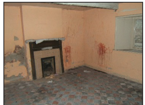
Plate 20: The fireplace and red and black tiled floor in the Cottage, A, viewed looking north-west
