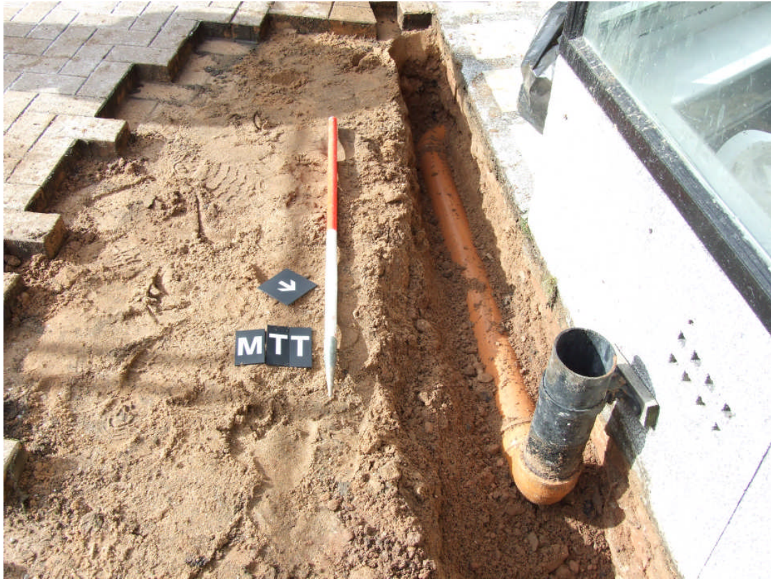
Plate 1. South-east facing section of trench with vent pipe in situ. Looking south-west.
