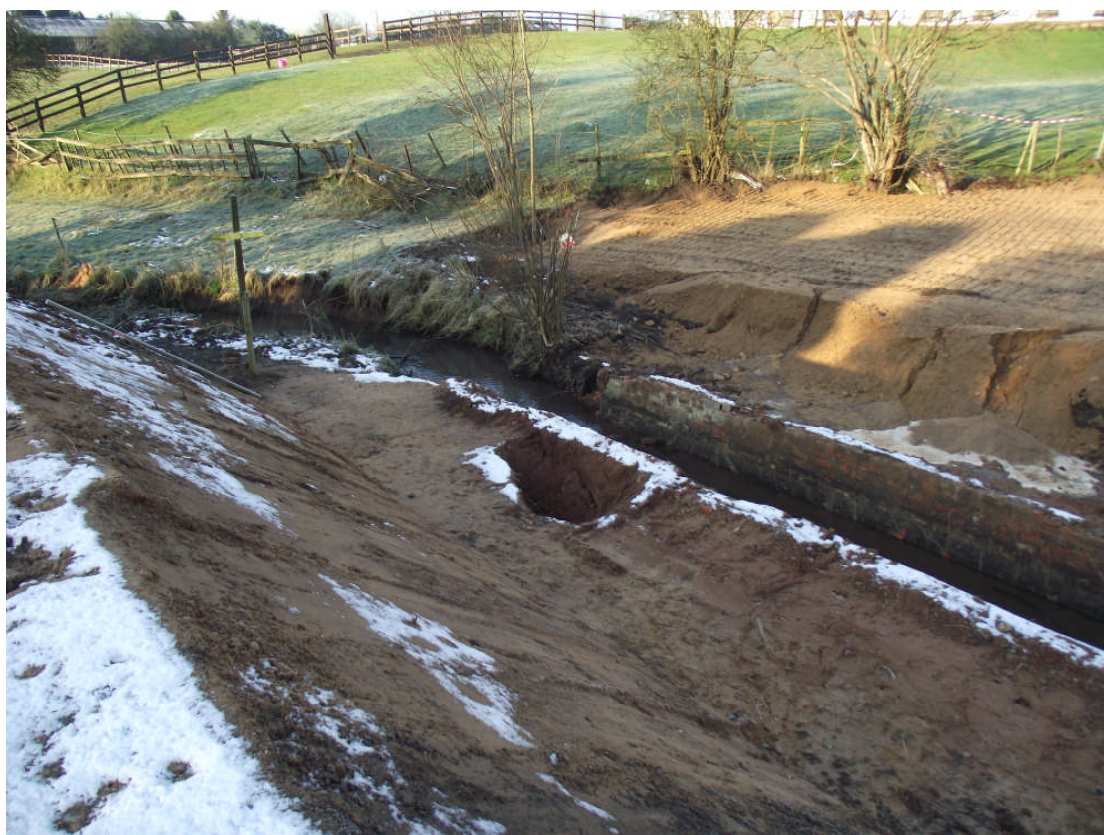
Plate 4. The partially demolished culvert with exposed sections of the embankment to either side after the sections had been battered and stabilised. looking north east.
