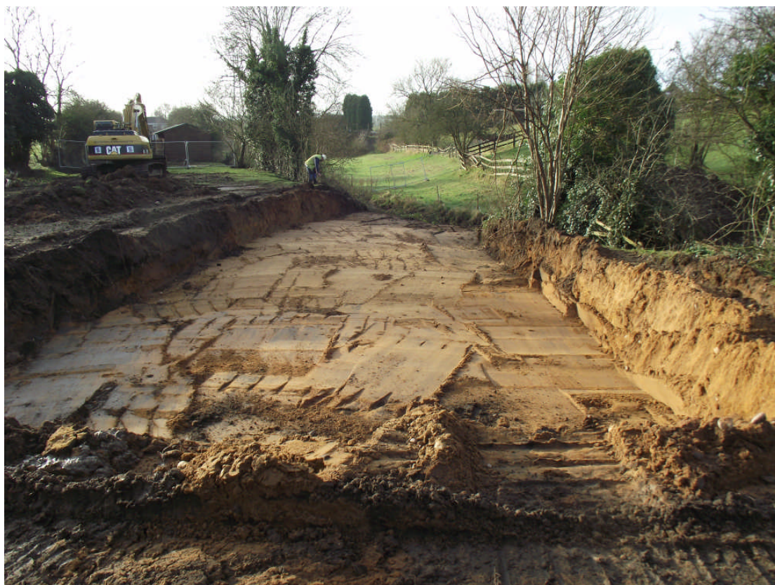
Plate 3. Excavated section through the embankment showing the sand which comprises the main element of the structure. Looking south west.
