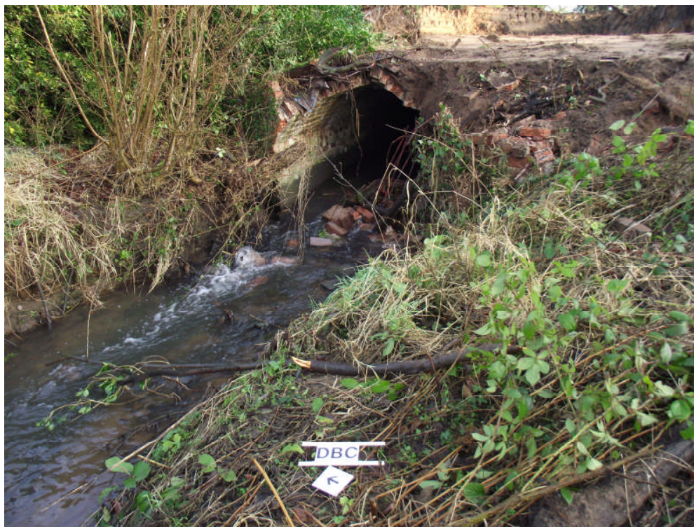
Plate 5. South West facing end of the culvert prior to the start of the demolition. Looking north east.
