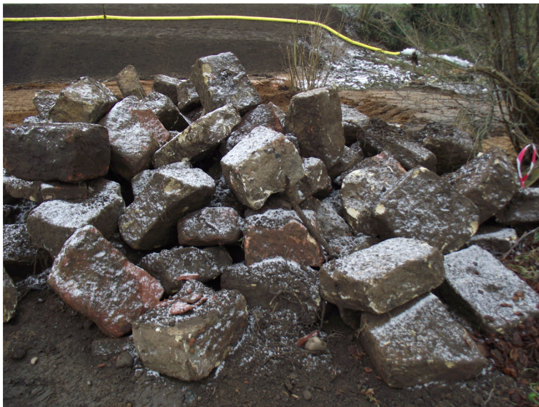
Plate 9. Blocks of masonry following their extraction. These were subsequently used to reinforce the newly created bank of the Dawley Brook. Looking south west.
