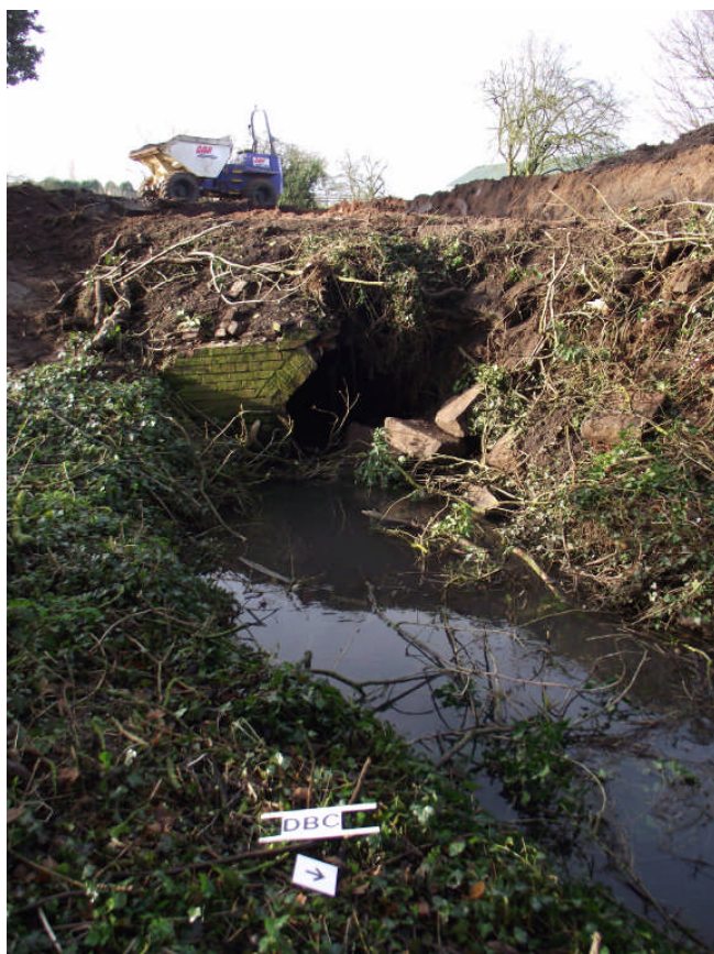
Plate 6. North East facing end of the culvert with part of the retaining wall intact. Looking south west
