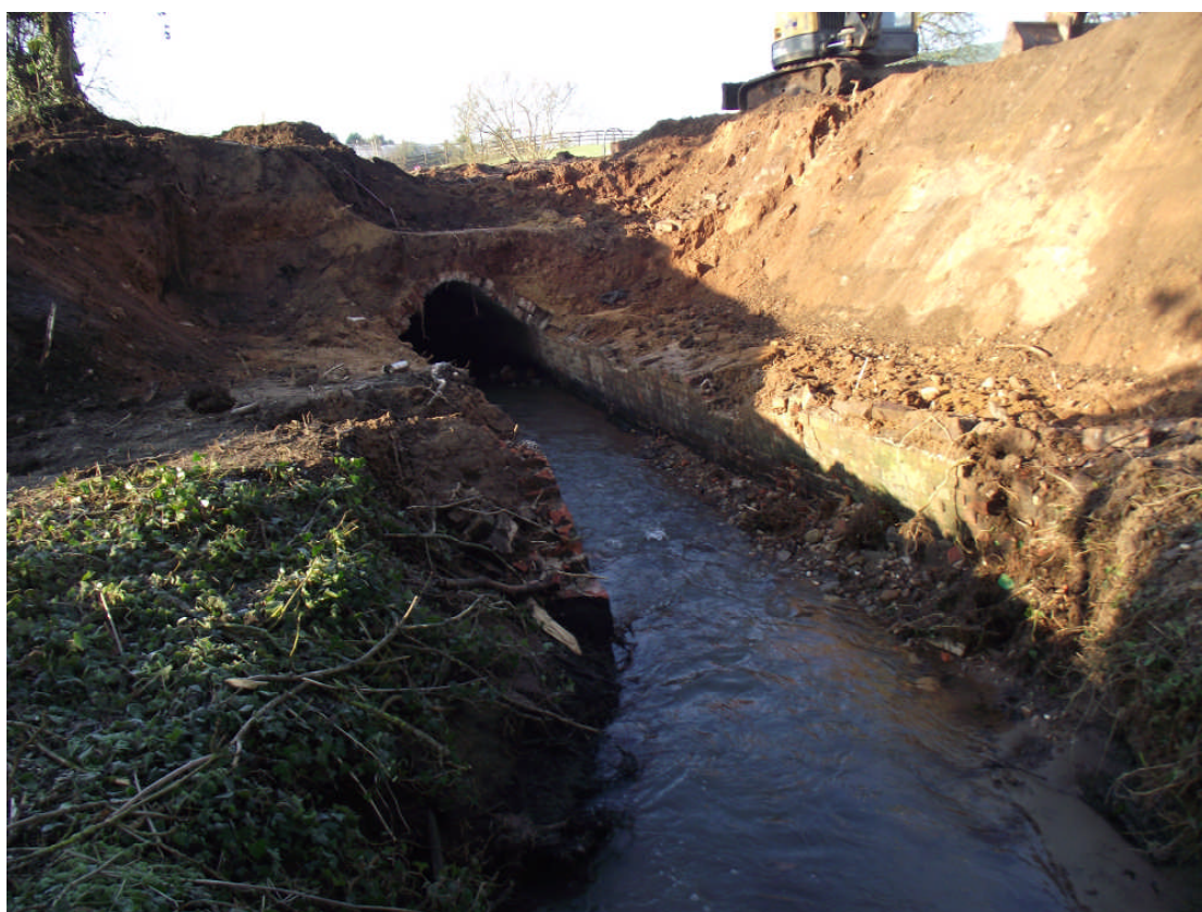
Plate 8. The culvert during demolition showing the removed overburden and stabilised bank. Looking north
