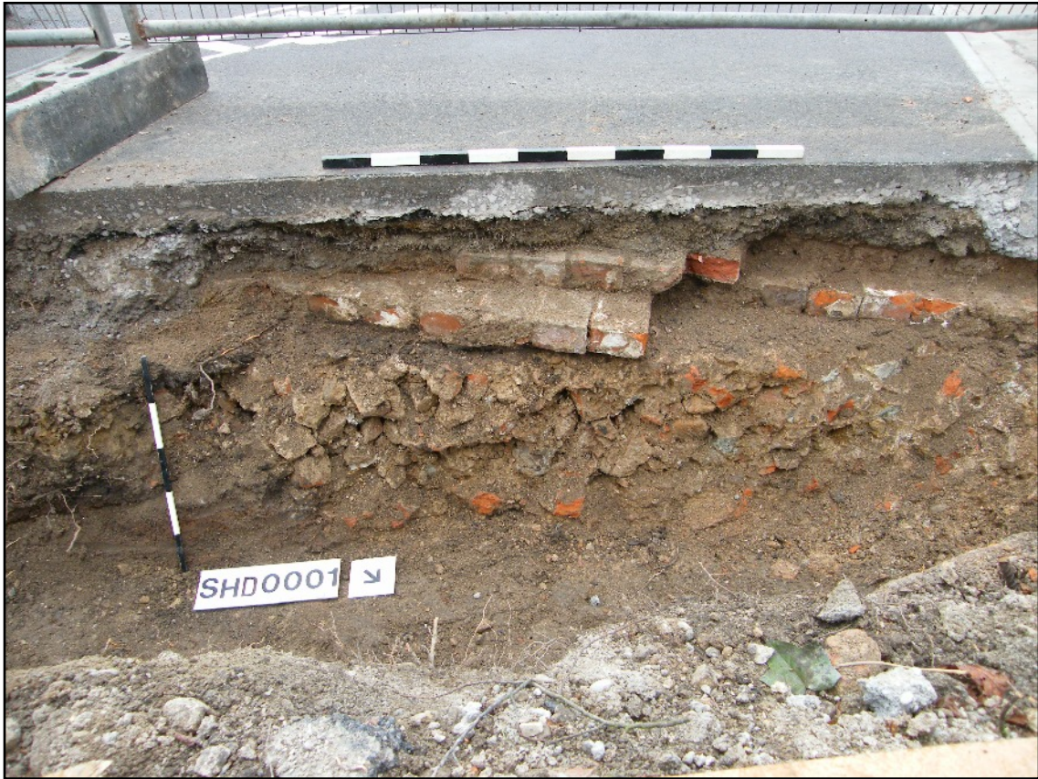
Plate 38: The foundations 0001 and 0002 for the western boundary wall of St. Helen's House, viewed looking south-west.
