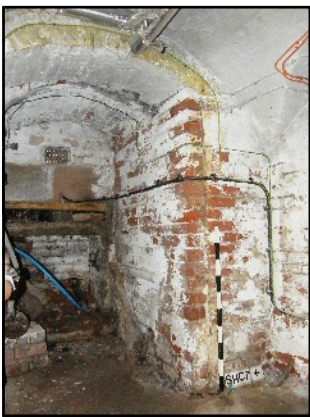
Plate 10: Former opening for the delivery of stock in the east wall of SHG7, viewed looking east.
