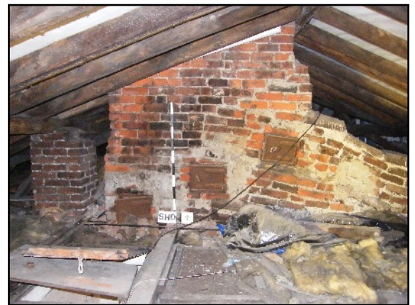
Plate 24: Northern chimney within the roof space with a brick pillar used to support the purlin to the west and part of the early external wall to the east, viewed looking north.
