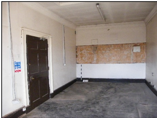
Plate 18: Metal hatches in the north wall of room SH27, viewed looking north-west.
