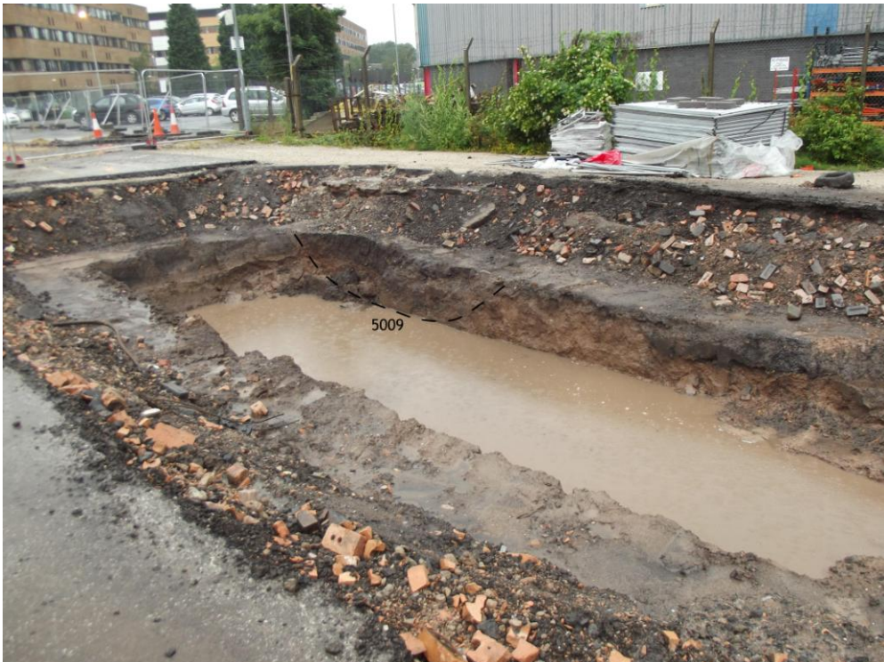
Plate 2: Western end of Trench 05 during excavation. The post-medieval ditch 5009 is marked in the south-facing section.
