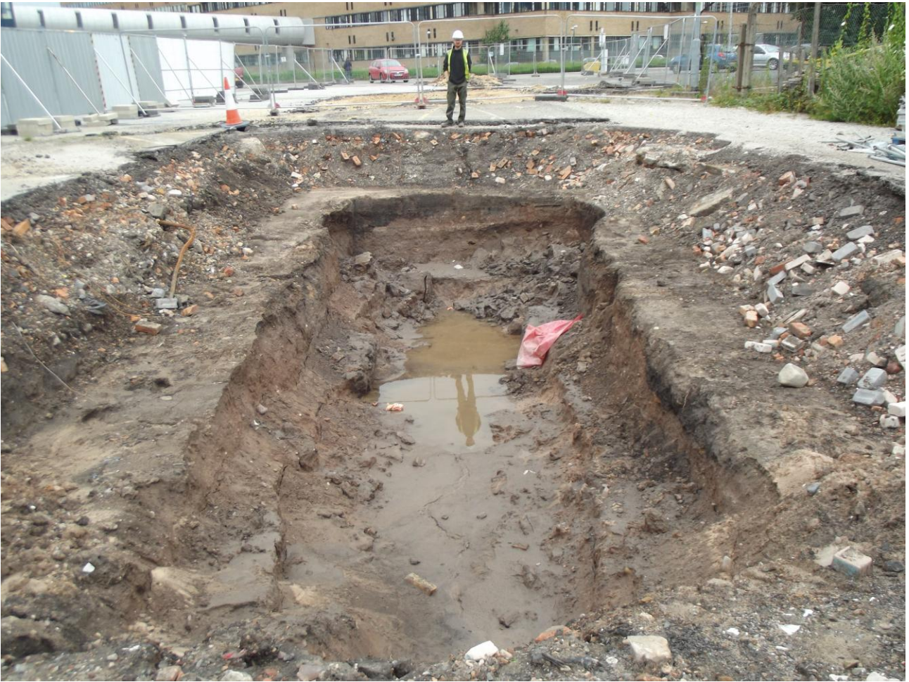
Plate 5: Trench 05 fully excavated post-flooding, looking west. The previously-inspected areas of diesel contamination and live services can be seen beyond the standing figure.
