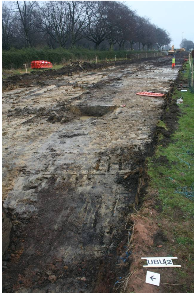
Plate 3: University Boulevard: East facing view of Area 1 after topsoil removal showing west facing section of [UBU2005]
