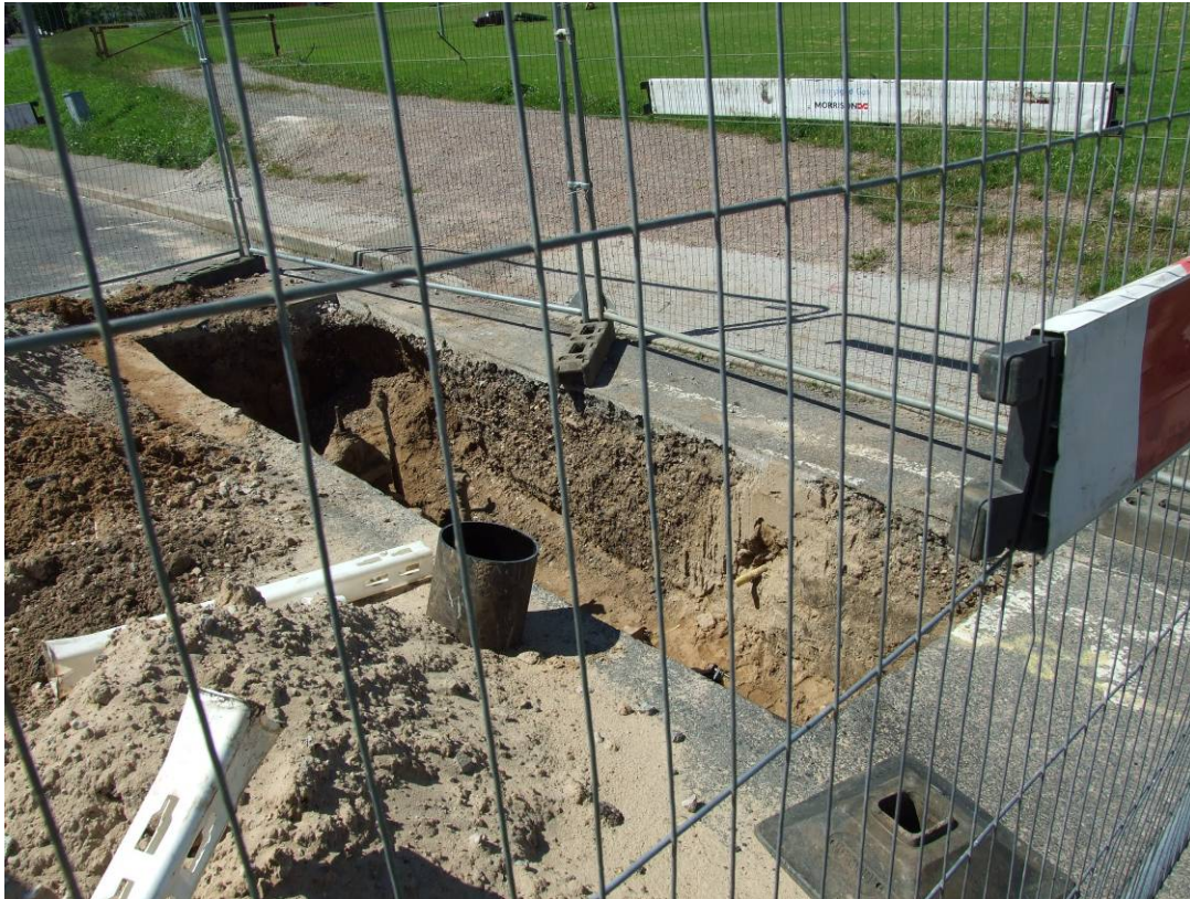
Plate 23: Wilford Toll Bridge: Small trench containing modern drain cut [WTB0004] in Area 02. Looking Southwest.
