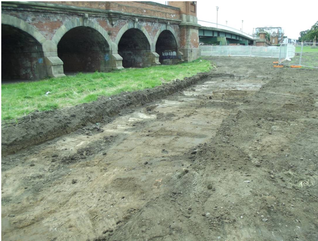
Plate 24: Excavation of flood plain adjacent to Wilford Toll Bridge including (WTB0023) and (WTB0026). Looking North.
