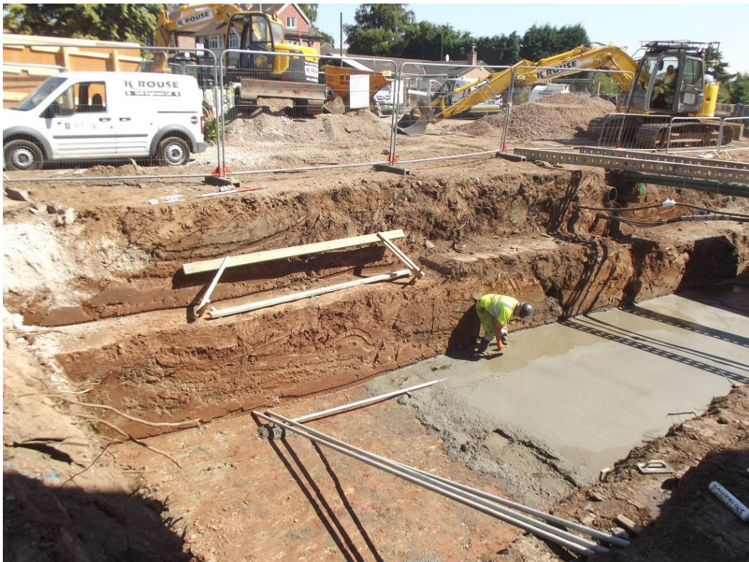
Plate 2: Chilwell: Wide trench near Sandby Court with concrete trackbed foundations. North facing shot.
