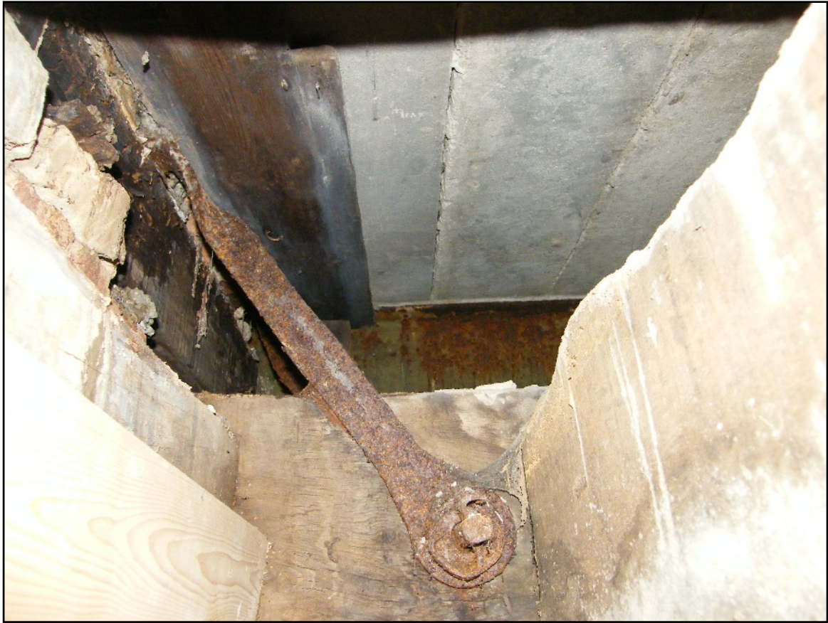
Plate 8: Metal tie in the South-east tower extending from a modern machine sawn timber in the west wall down to the original oak ceiling beam below. Viewed looking north.
