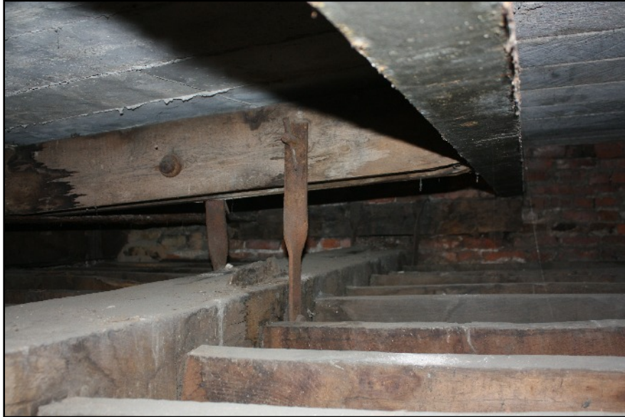
Plate 1: View of the void within the South-west corner tower showing the timber and metal girder supports for the concrete plank floor and the additional metal ties between the later timber and the original ceiling beam below. Viewed looking north-east.
