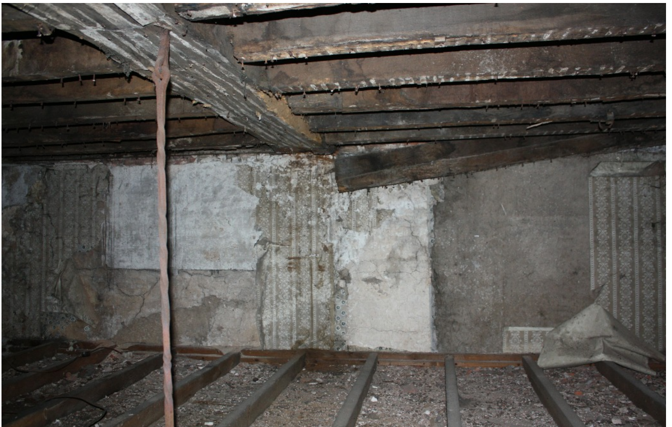
Plate 5: East wall of the Upper Room in the South-west corner tower illustrating the differing wall paper heights, viewed looking north-east.
