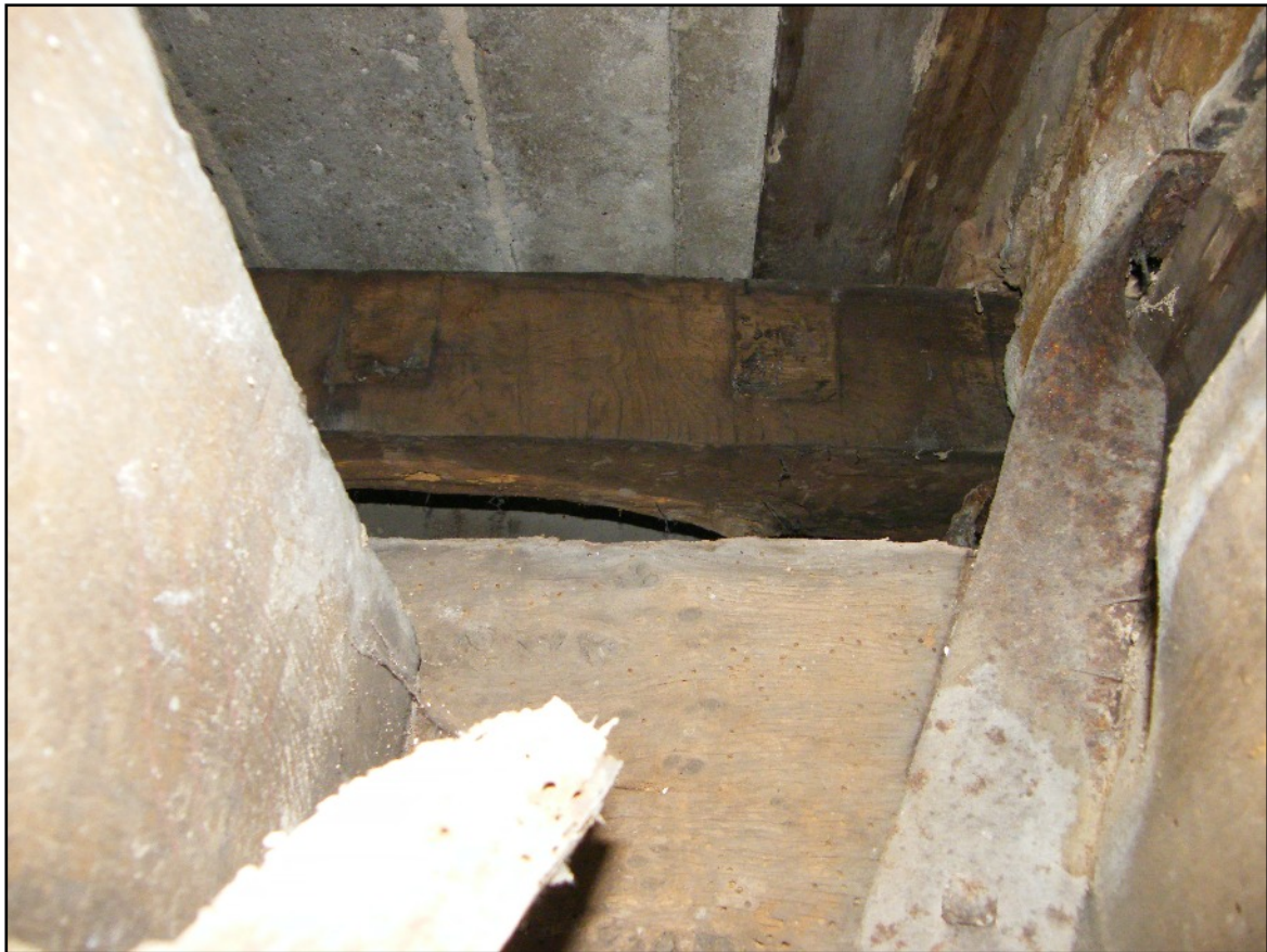
Plate 9: The reused timber beam in the North-east tower supporting the concrete planks, viewed looking south. Note the metal tie extending from the timber embedded in the brickwork of the west wall to the main ceiling beam.
