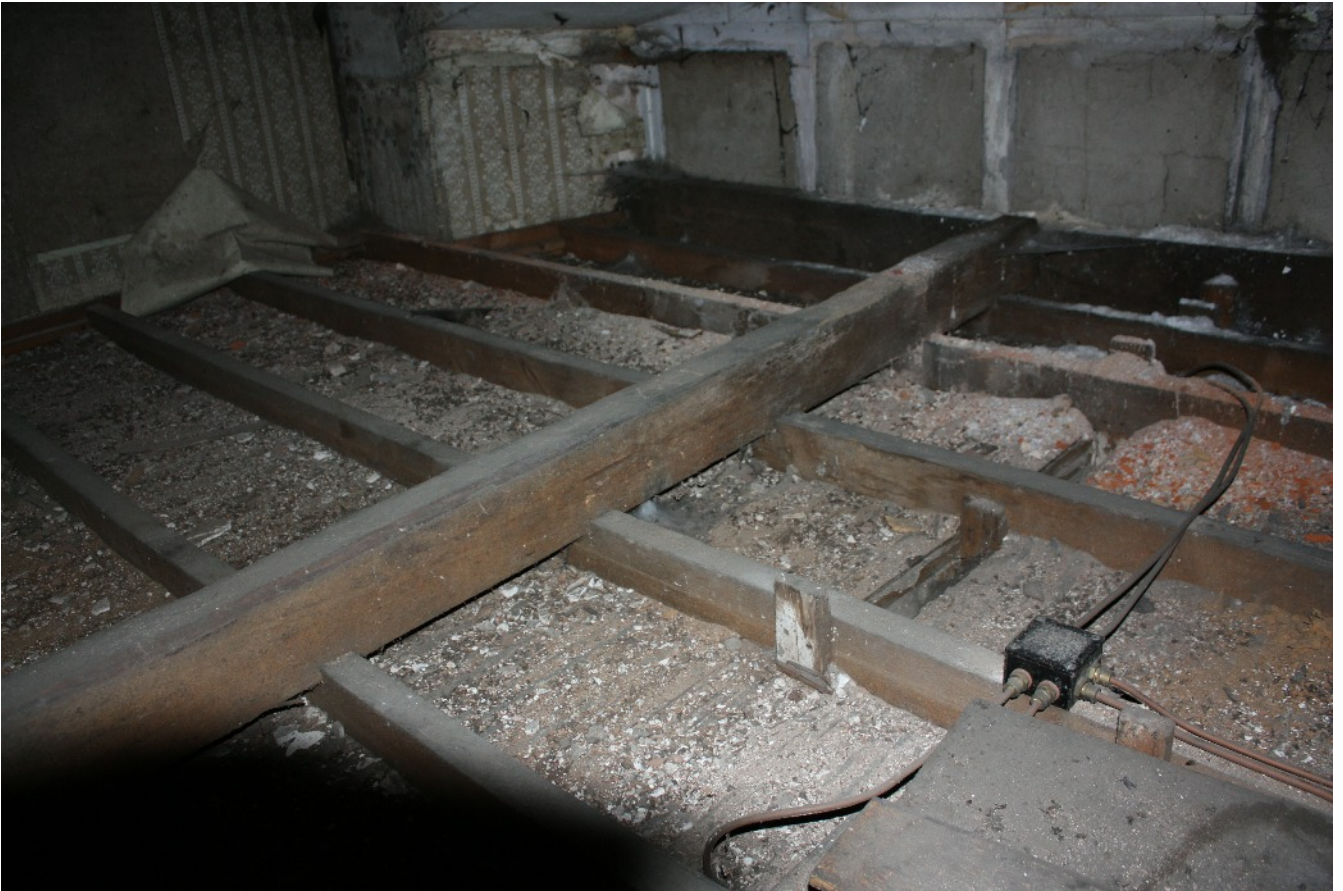
Plate 4: View of the floor structure of the inserted floor structure within the South-west corner tower, viewed looking south-east.
