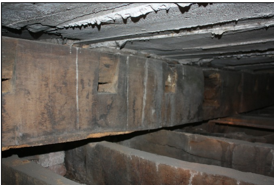
Plate 3: Detail of the re-used ceiling beam supporting the concrete roof in the void of the South-west corner tower. Viewed looking north-east.
