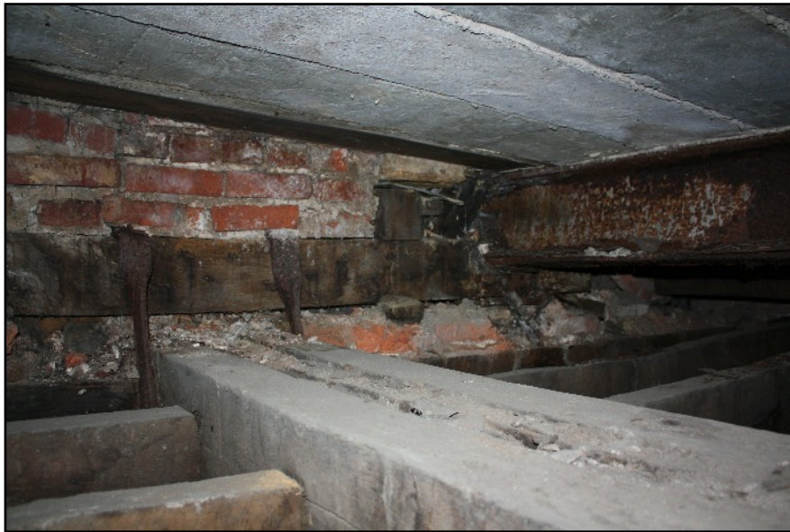
Plate 2: Northern metal girder supported by a timber embedded in the west wall in the void of the South-west corner tower. Note the metal ties between the wall timber and joists below. Viewed looking north-west.
