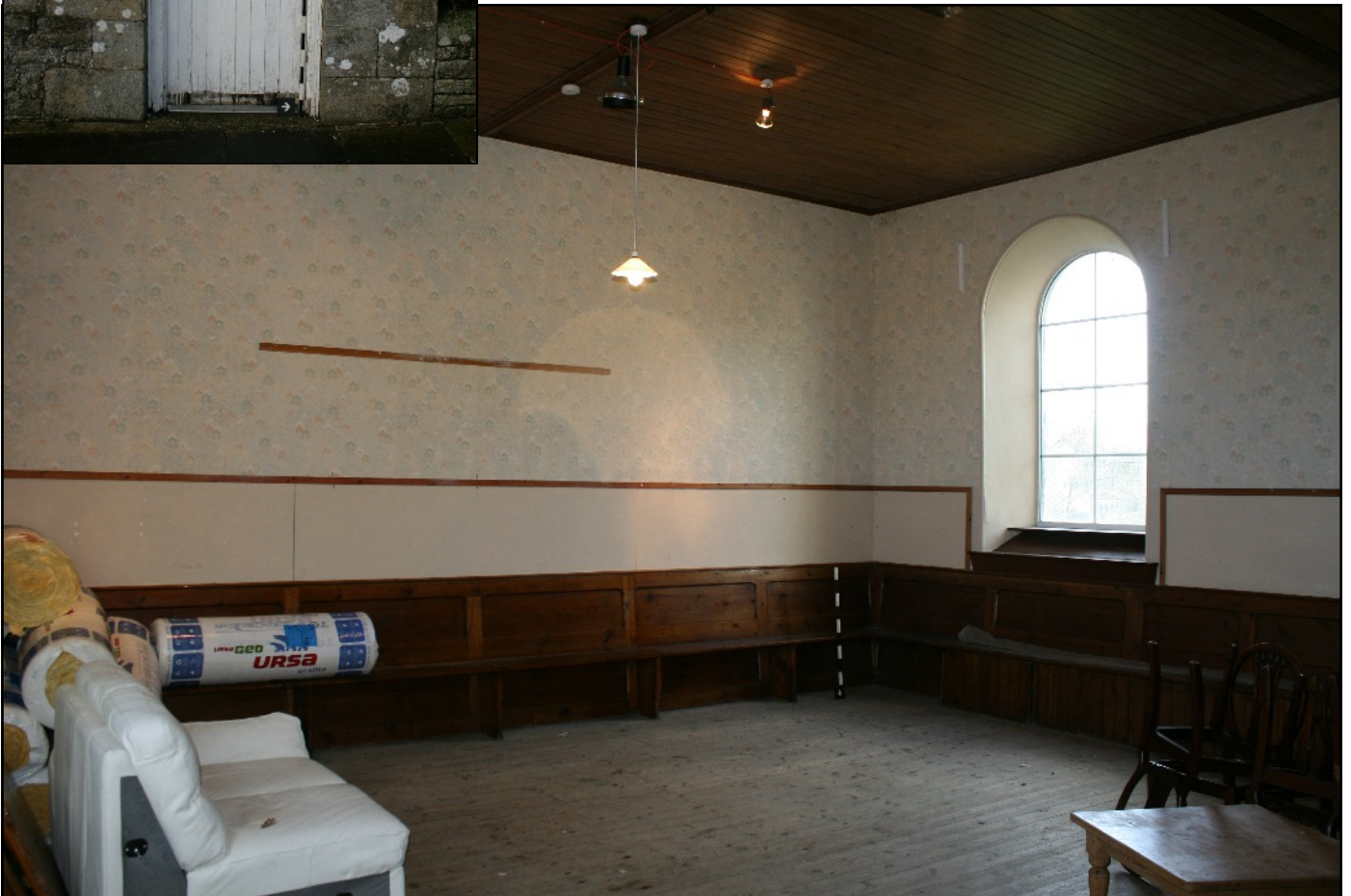
Plate 5: General view of the interior of the Sunday School, viewed looking south-west.
