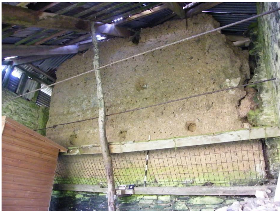
Plate 4: The northwest back wall of the shippon containing holes for a ridge and ceiling beams, viewed looking southeast.
