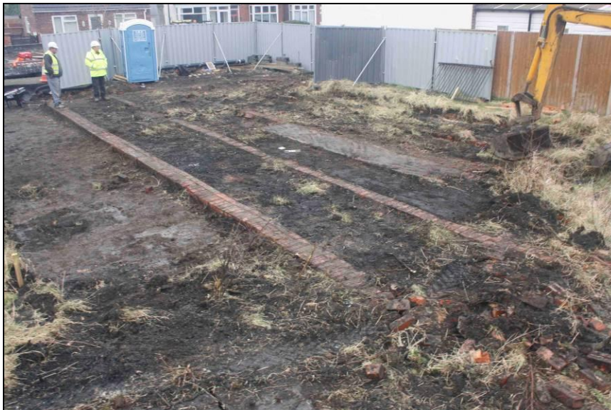
Plate 3: General view of south end of Trench 1, showing footings of the 1912 structure
