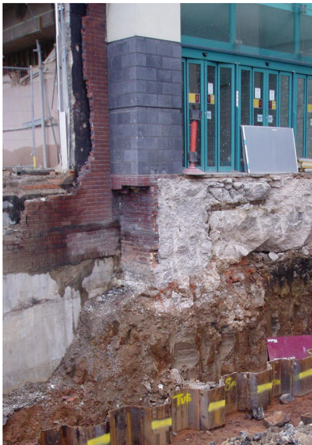
Plate10 Area 21, at entrance to Eagle Centre in the area of the now demolished Castlefields Centre. Evidence of sub-basements to the bottom left of the plate and beneath the doors shows the depth and extent of the truncation that happened during the 1960s and 1970s.
