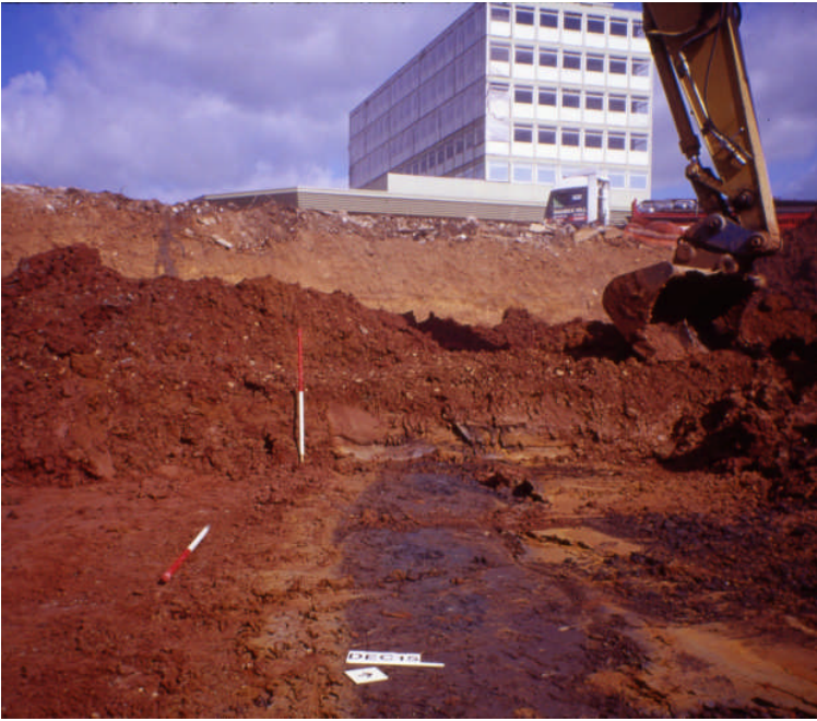
Plate 7 Area 15: silts of the Palaeochannel that occurred at the base of the excavation of the sub-basements (6.87m lower than London Road). The thickness of the silts at the base was less than 0.05m and only slightly thicker in section.
