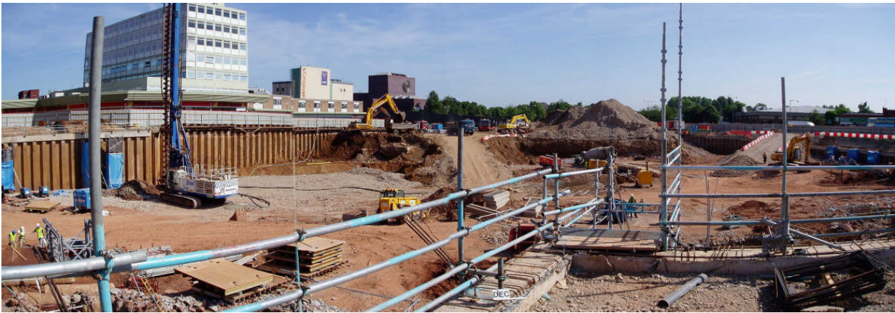
Panoramic view across the site during groundworks ahead of the new Eagle Centre
