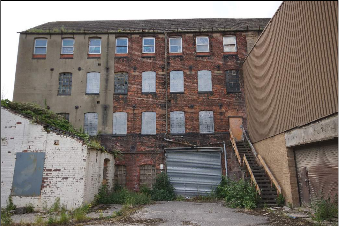
Plate 12: The southern brick extension Phase E viewed looking west. Note that the mill is abutted by the sub-station Phase H, the white brick building on the left and the modern shed Phase M.
