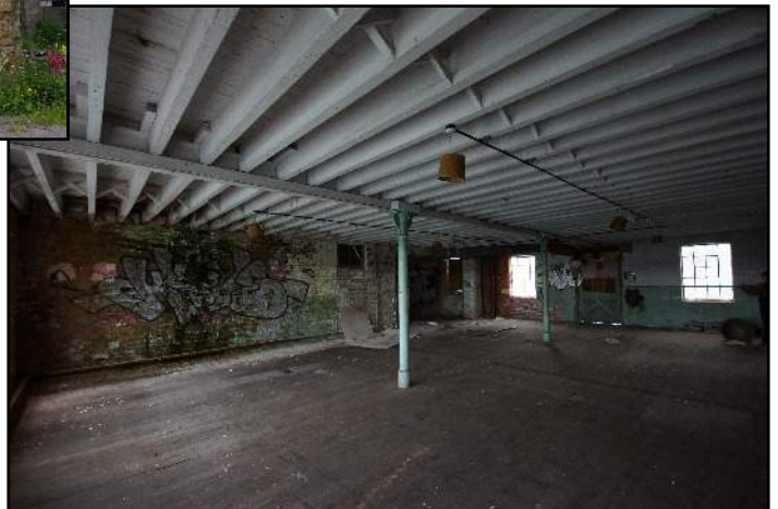
Plate 16: General view of the second floor of Phase G, viewed looking south-west.
