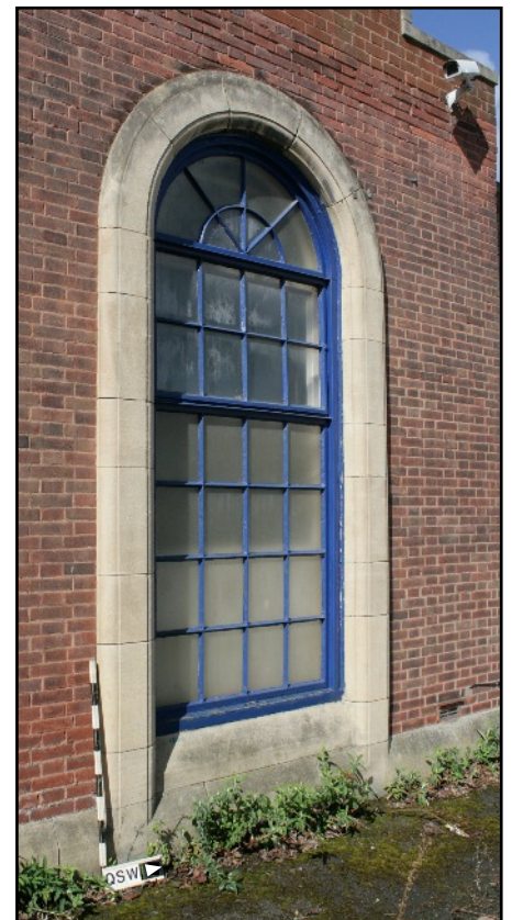
Plate 3. Art deco style window in the east elevation of 30 Watson Road, viewed looking north-west.
