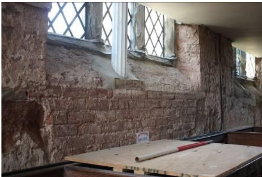
Plate 8. Area 01. Interior of the church showing the bricked up entrance of the south porch. Looking south west.
