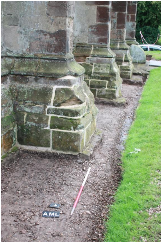
Plate 18. Area 06. Oblique view showing shallow excavation and the gravel infill from the 1975 drainage works in situ. Looking west.
