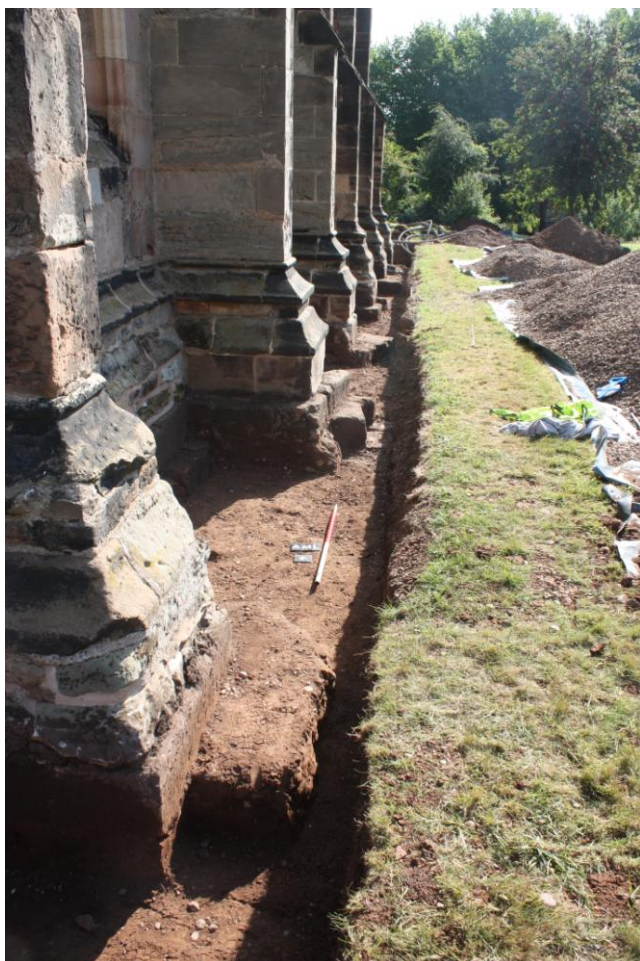
Plate 4. Area 01. View along south facing wall of south aisle after excavation. Looking east.
