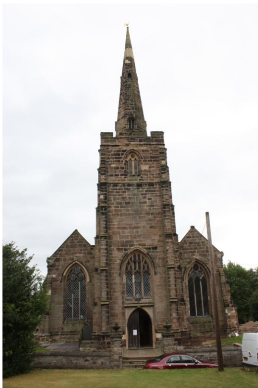
Plate 1. North and south aisles of the church flanking the west tower. Looking east.
