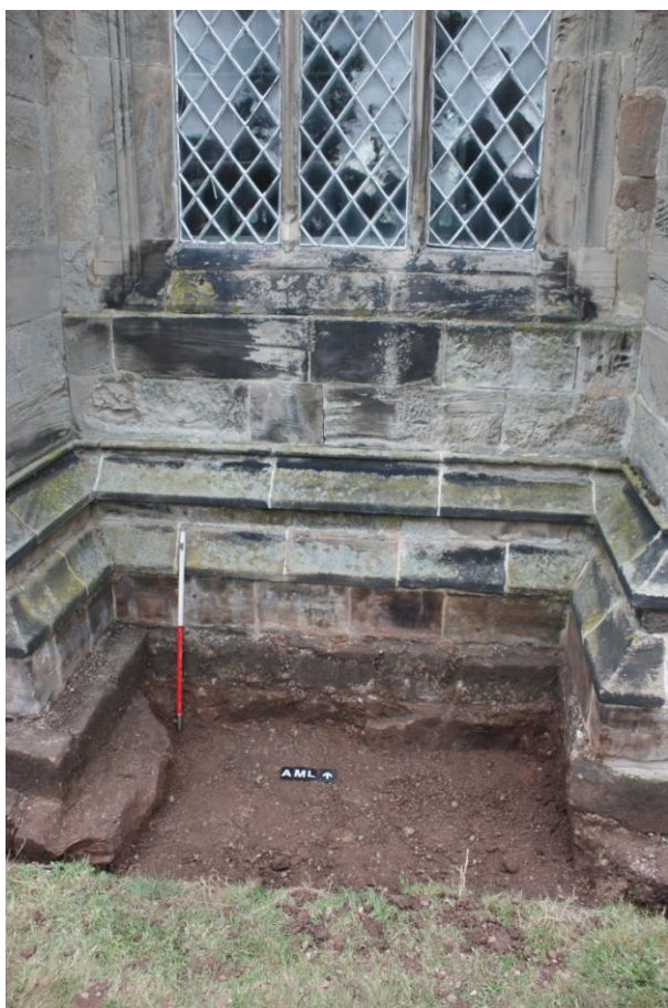
Plate 7. Area 01. South facing wall at the location of the now demolished south porch. Looking north.
