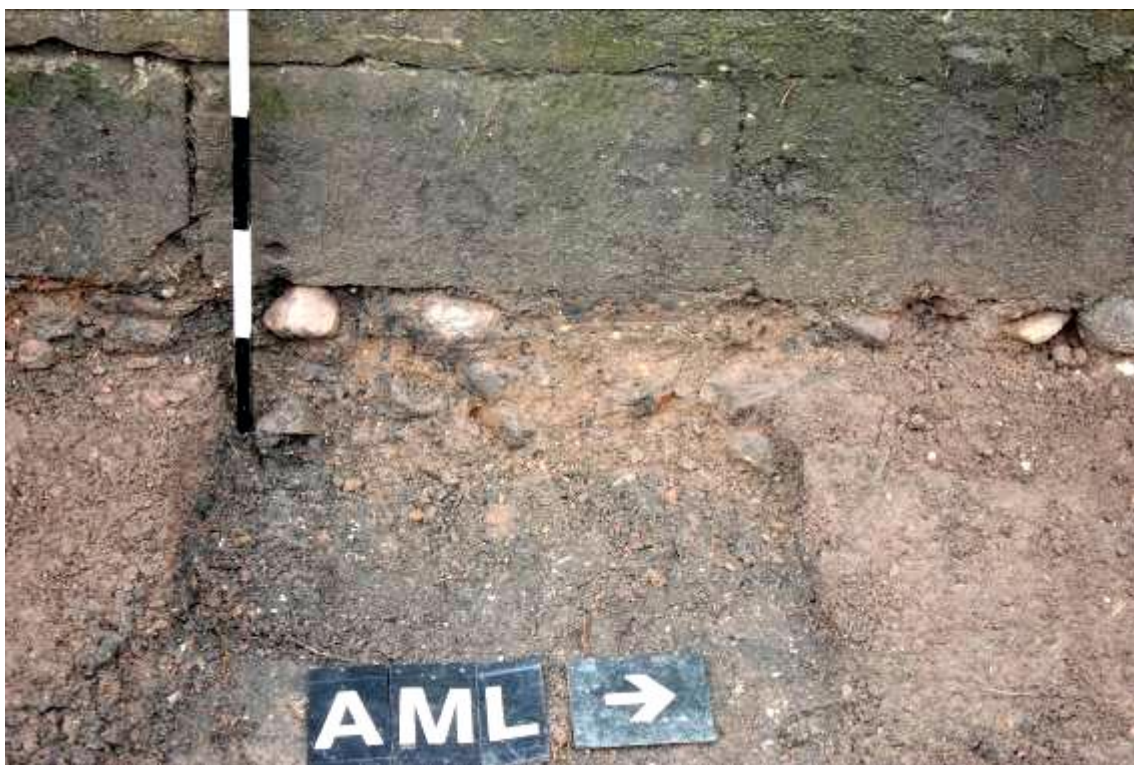
Plate 15. Area 04. Detail of east facing wall of Appleby Chapel with sondage showing extent of pebble foundation. Looking west.
