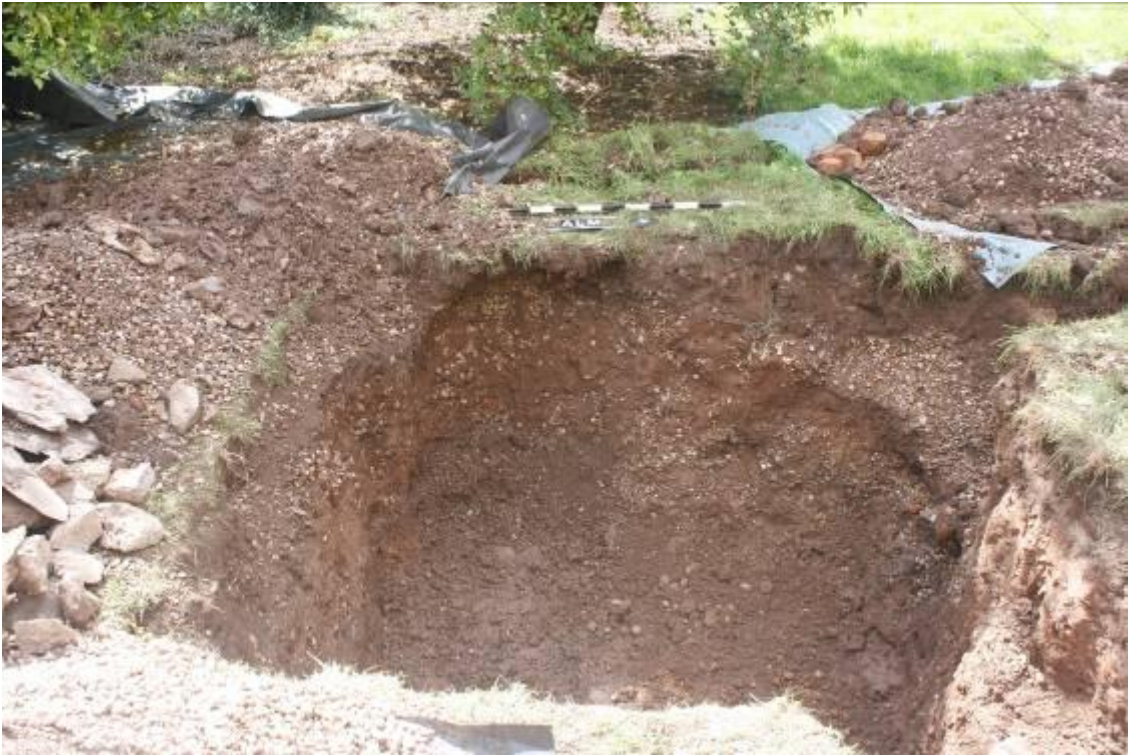
Plate 22. Area 12, soakaway showing unstable section. Looking south.
