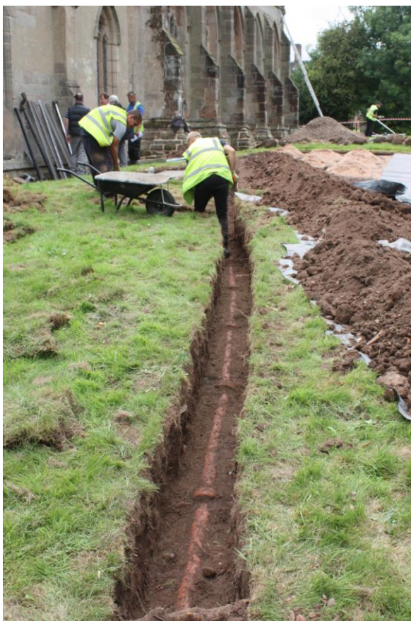
Plate 20. Area 07. Drainage trench showing existing ceramic pipes laid in 1975. Looking south west.
